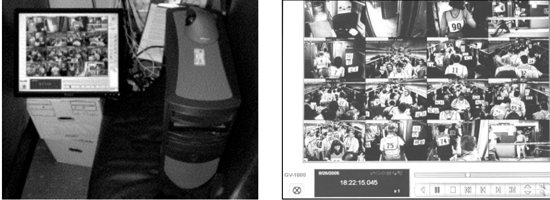
Figure 10. Video Data Recording Screen and Hard Drive; Screen: Close-up
