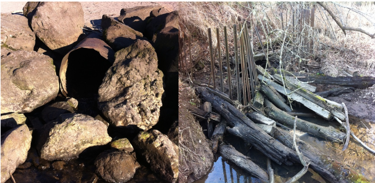
Figure 4. Current conditions of Culvert Outlet (left) and culvert inlet (right) with trash rack on Tributary 3.
