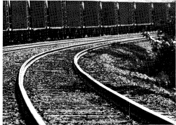
(d) Alignment Kinks in Spiral Location D, Looking East
