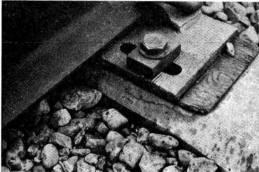
Damage Caused by Excessive Anchor Bolt Torque Fig. E-13
