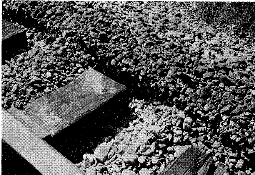
Migration of Ballast Inside of Stabilized Shoulder - July 1975 Fig. F-8
