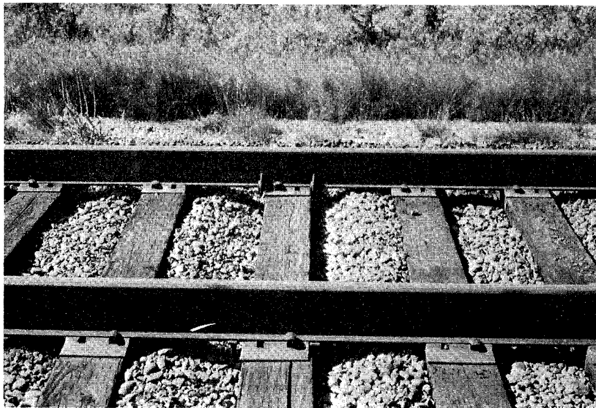
Signs of Back and Forth Tie Movement - July 1975 Fig. F-10
