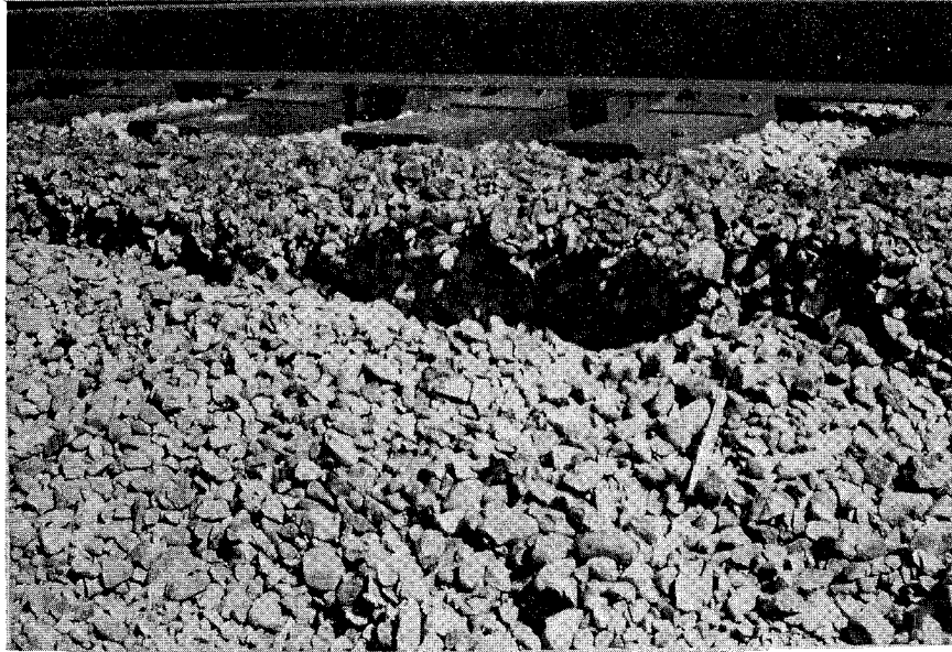
Settlement of Ballast Outside of Stabilized Shoulder - July 1975 Fig. F-7
