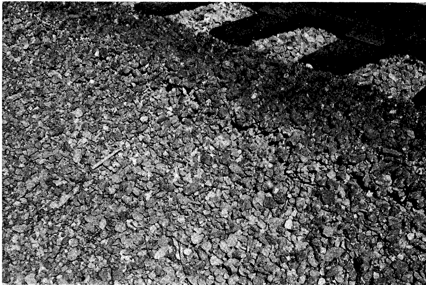
Beginning of Ballast Settlement Outside Stabilized Shoulder - July 1974 Fig. F-4
