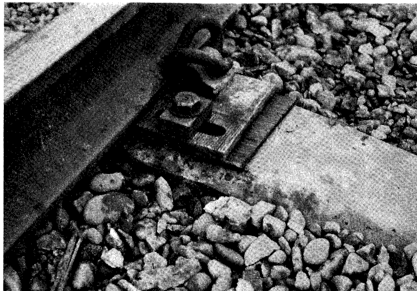
Spalled Concrete Caused by Over Torqueing Anchor Bolts Fig. E-12
