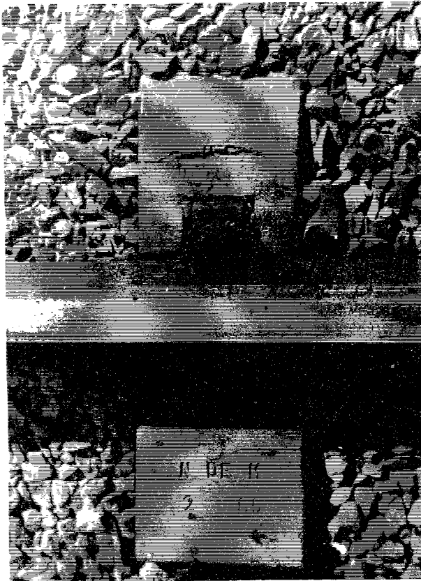
PLATE 37. DAMAGE TO CONCRETE AT SEAT OF RAIL CLIP CAUSED BY SLACK IN FASTENING
