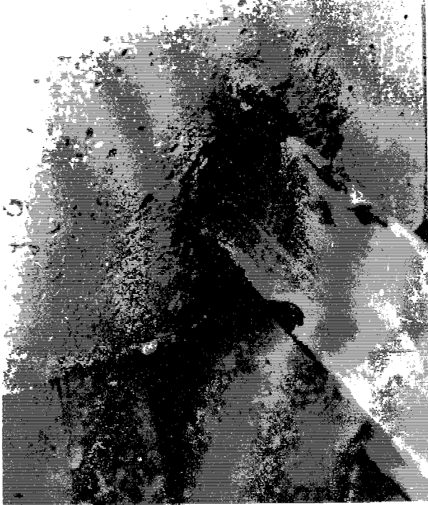
PLATE 40. CORROSION OF STEEL TIEBAR IN SWAMPY REGION
