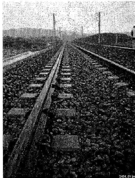
Figure 1. TGV Line – Ballast Track with Dual Block Sleeper
