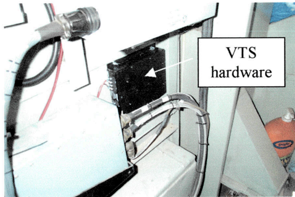
Figure 2. Locomotive Installation of Vehicle Tracking System Hardware (Courtesy of Radio Satellite Integrators, Inc.)
