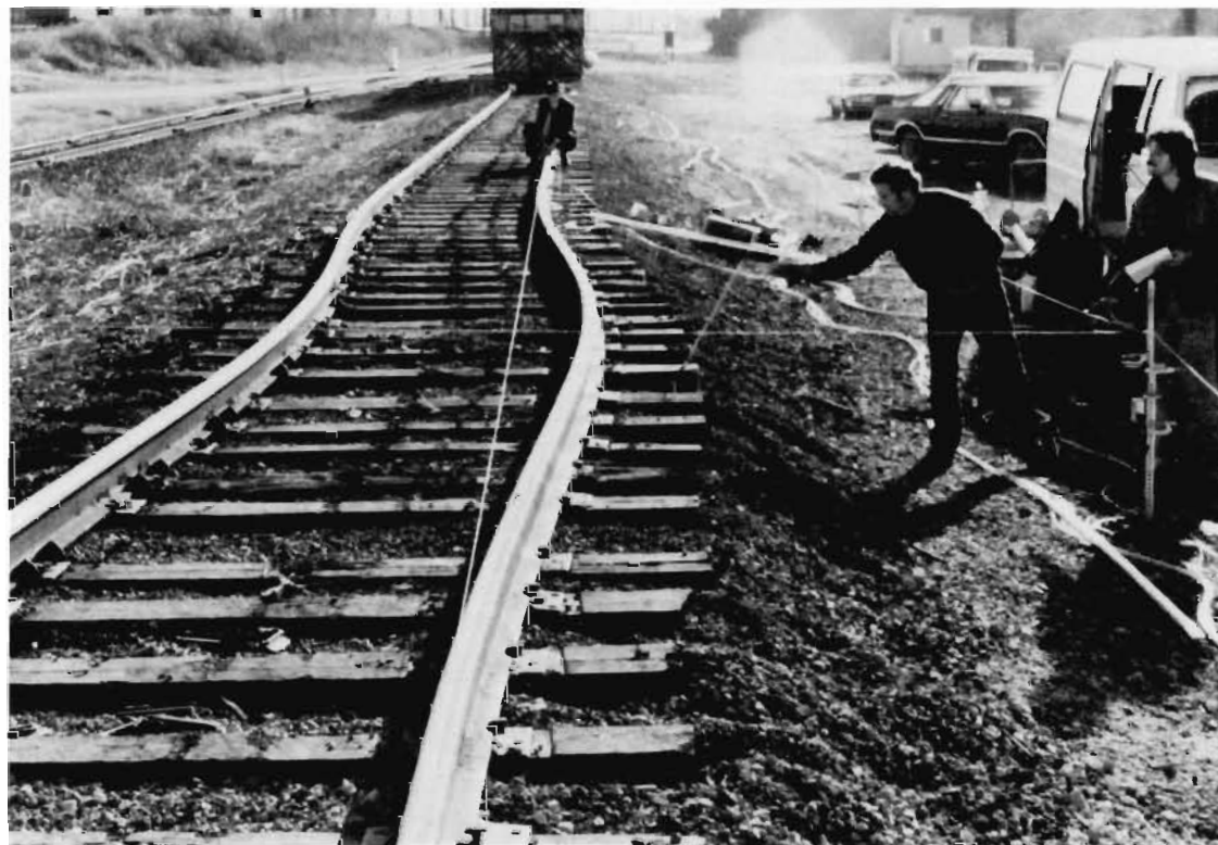
TYPICAL THERMALLY-INDUCED LATERAL TRACK SHIFT (BUCKLE)
