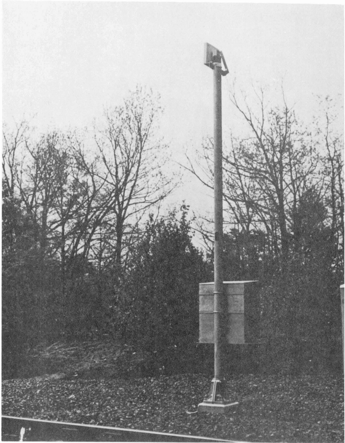
Figure 3.3 Transmitter Installation - Typical of Later Sites
