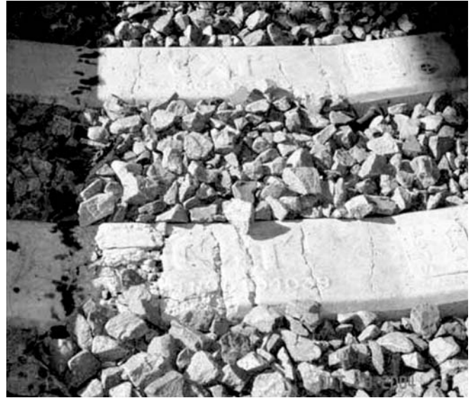
Figure 2 Cracked concrete ties at the abutment of a freight railroad ballast deck bridge caused by impact loads.
