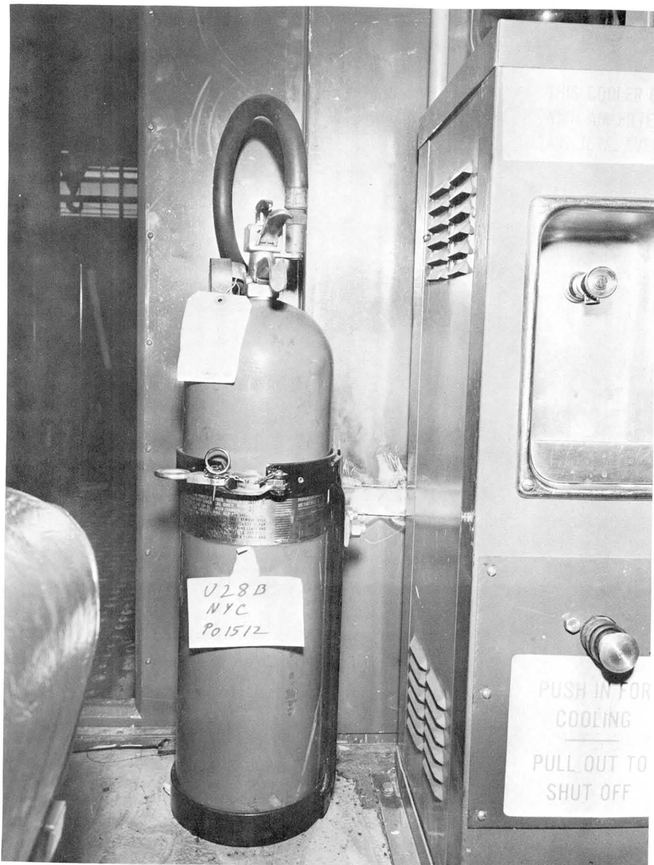
Fig. 1.22 Undesirable location of fire extinguisher and water cooler, obstructing passageway (GE U28B model)
