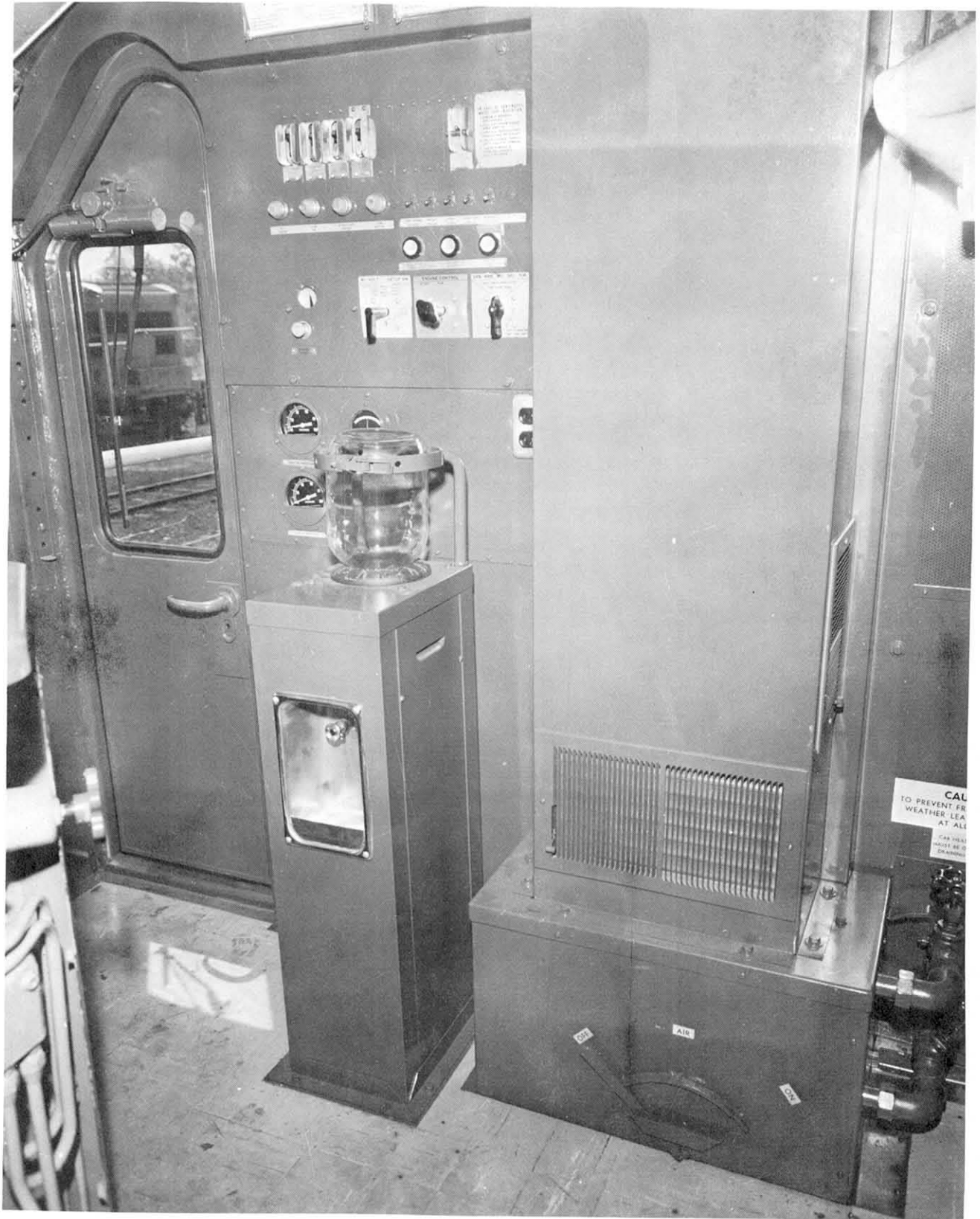
Fig. 1.21 Undesirable location of water cooler and heater in the middle of the cab. Note sharp edges and corners, free piping and valves (GE U25 model)
