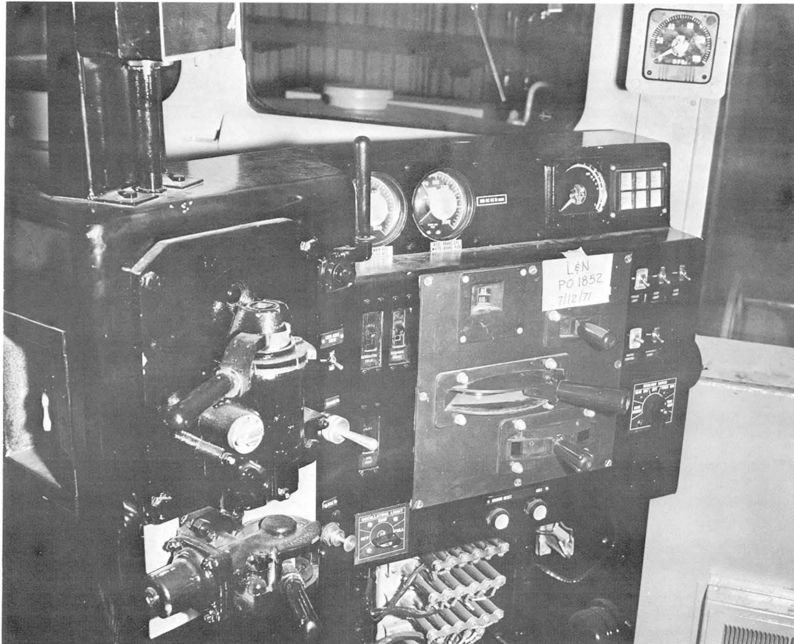
Fig. 2.14 GE control stands were equipped with EMD controllers in 1971
