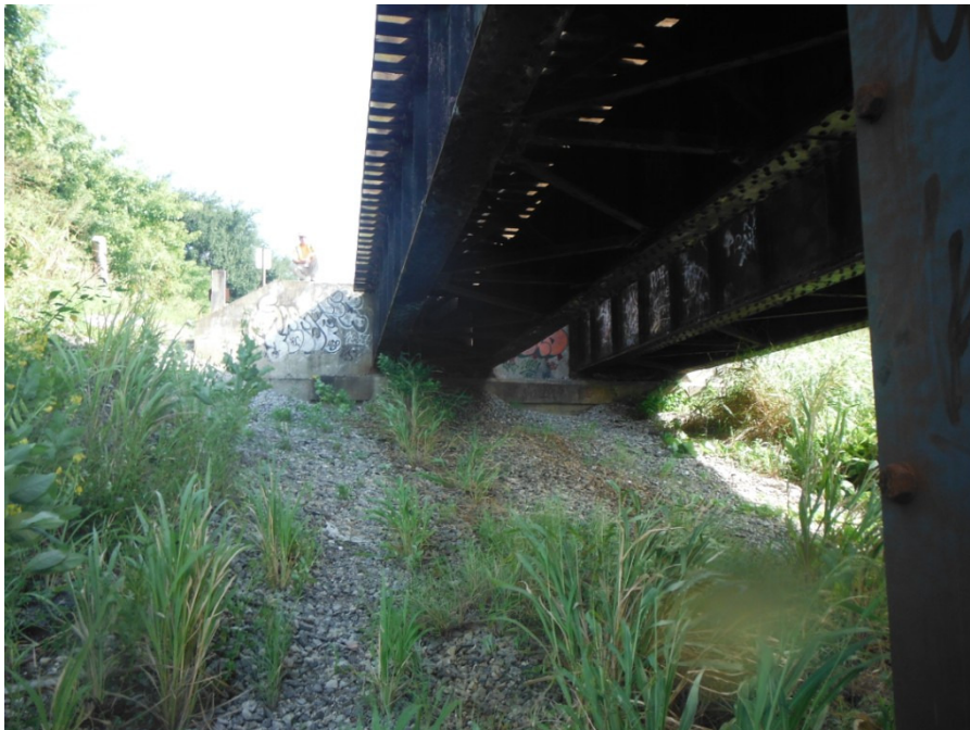
Photograph 8. Sebastian River (Mile Post: 212.07), South Side of the Sebastian River Railroad Bridge
