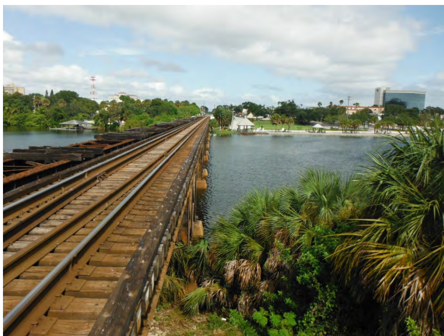
Photograph 4. Crane Creek Bridge (Mile Post: 194.47), Facing north toward to the waterside park
