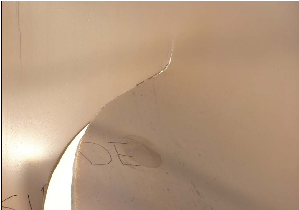
Figure A-10. Cracked Shell above the Ram (Interior Side)
