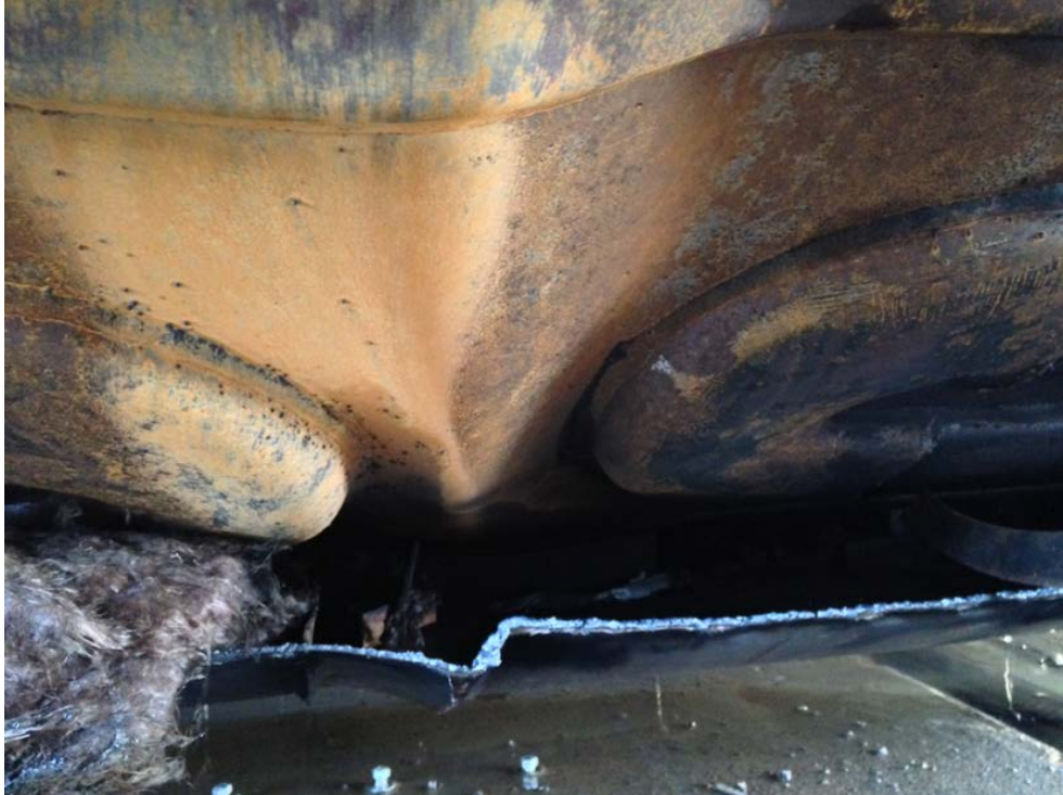
Figure 44. Localized tank buckling between coils at tank center, near base of tank. Jacket cut away locally to expose inner tank.
