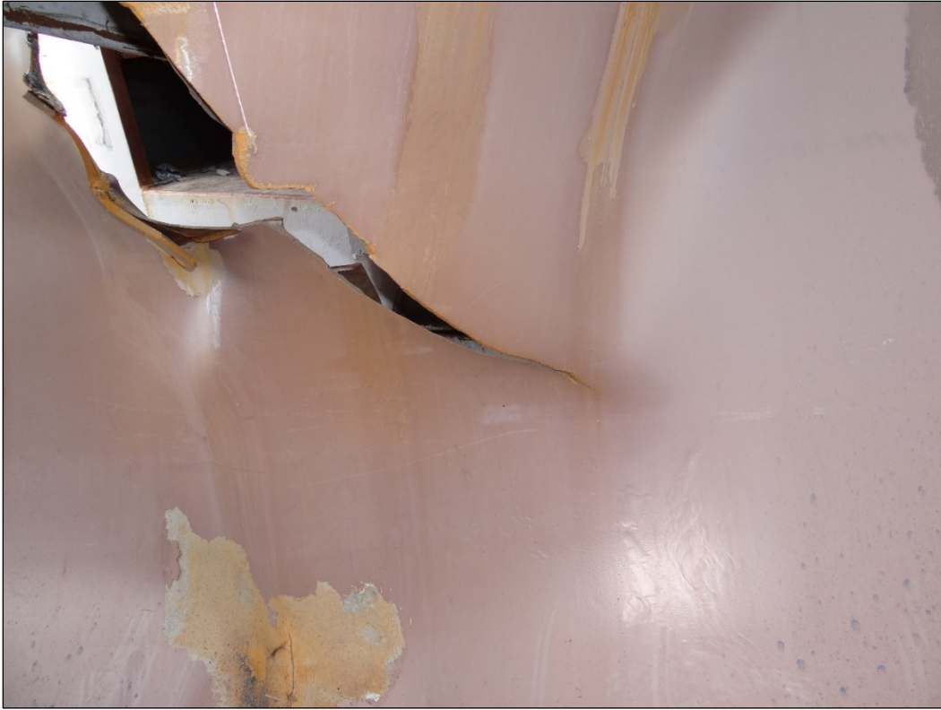
Figure A-9. Cracked Shell below the Ram (Interior Side)
