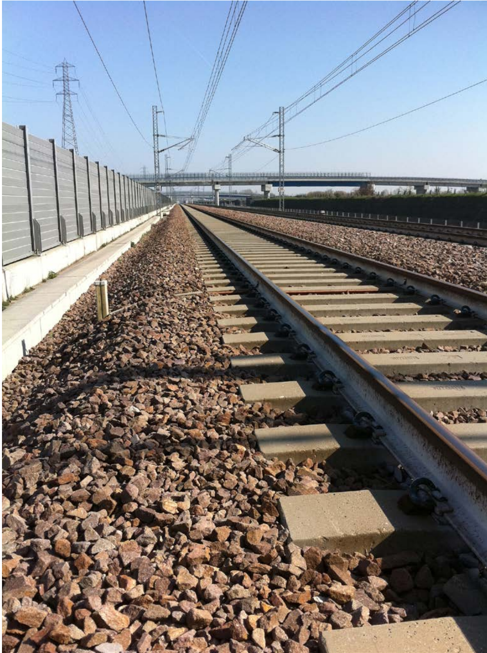
Figure 4.9: Example of HS track where no ballast particles are present on top of the sleepers.
