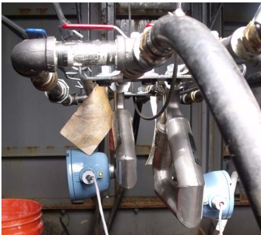
Fuel Mass Flow Measurement System
