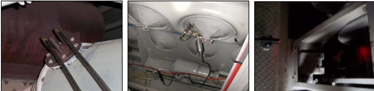
(a) exhaust sampling port and metal tubes; (b) manifold absolute pressure (MAP) sensor; (c) RPM sensor
