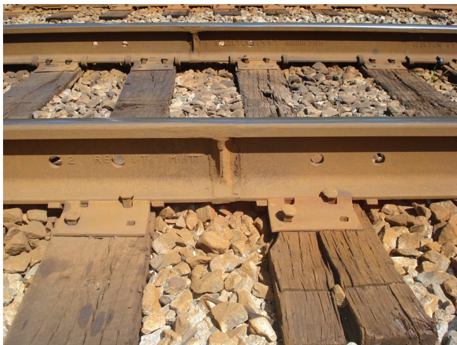
Figure 58: Boutet Weld in Track
