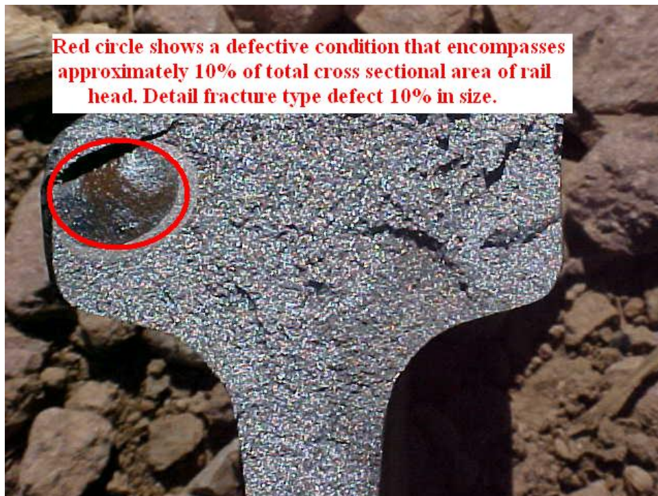
Figure 1: Identifying Transverse Defects in Relation to Cross Sectional Area of Rail Head
