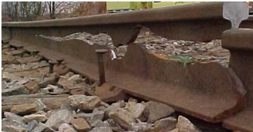
Figure 31: Web Failure Resulting from High Residual Stress
