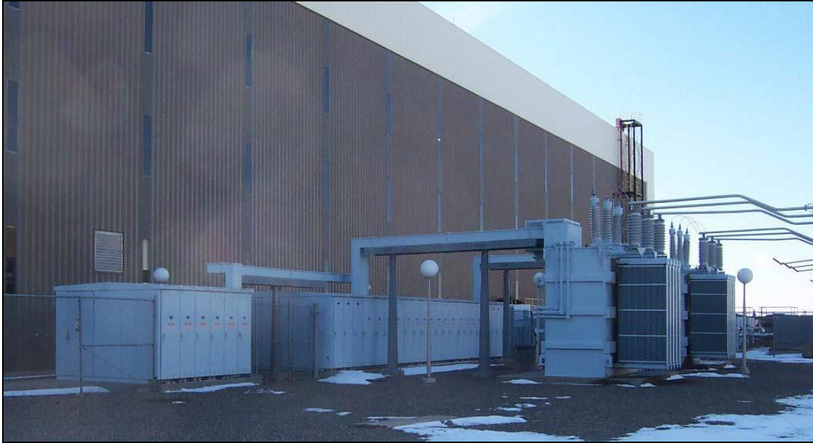
Figure 49. Main Core Area Substation
