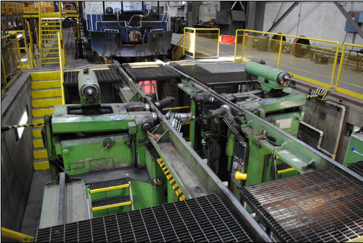
Figure 9. Wheel Truing Machine in the CSB
