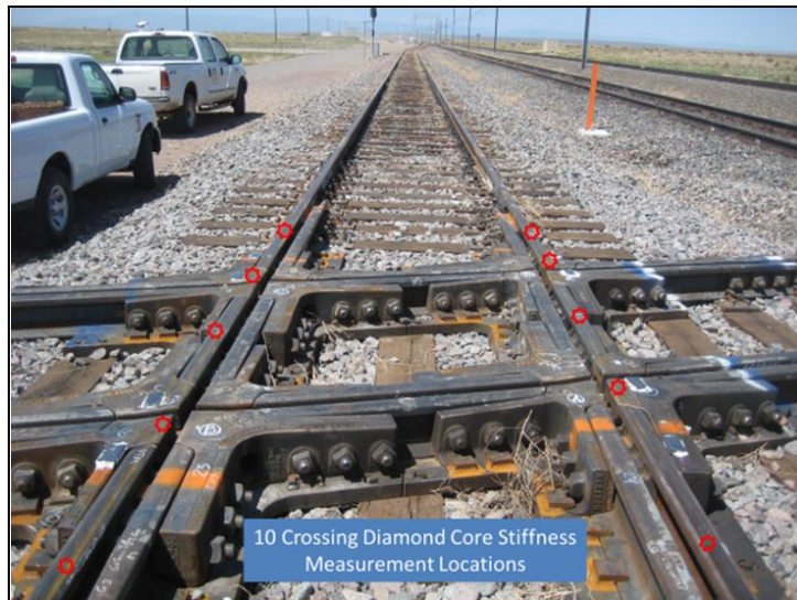
Figure 71. Locations of the 10 (5 on each rail) vertical track stiffness measurements taken at the core of the crossing diamond for each test case
