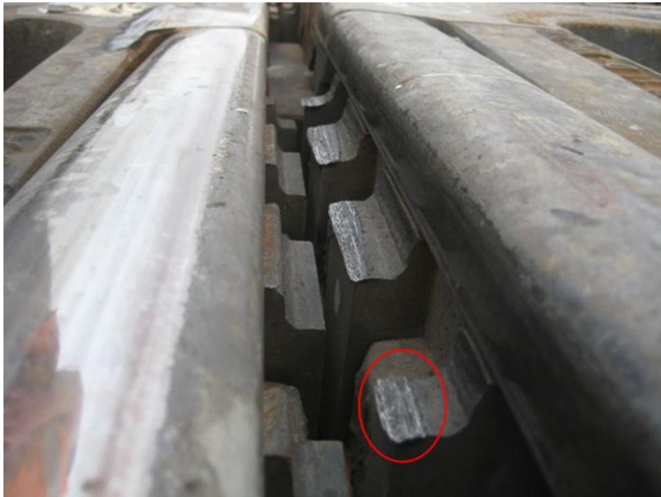
Figure 99. Wheel flange marks on the split spacer fastened to the rising guardrail
