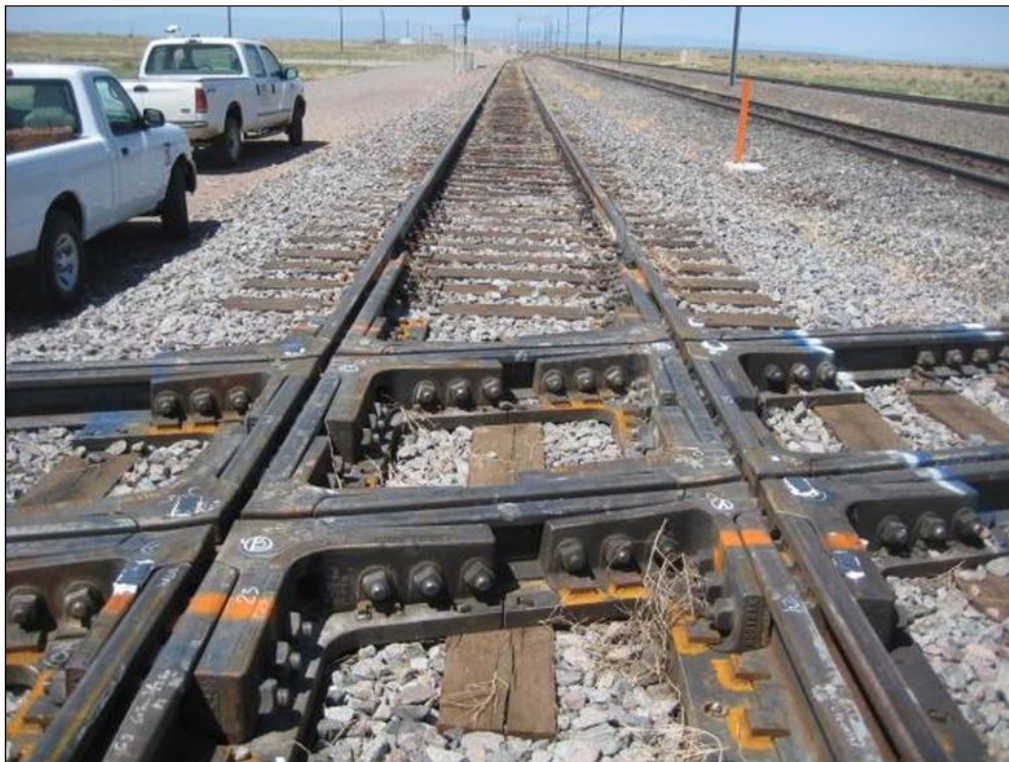
Figure 5. The test prototype crossing diamond as installed is a modified version of the basic SRR crossing diamond design
