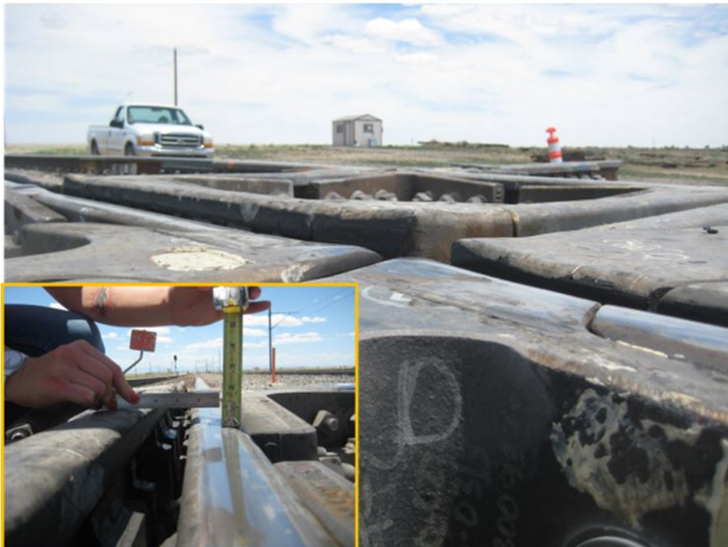
Figure 97. Differential elevation between the guardrail (left) and the running rail (right), about 1 in
