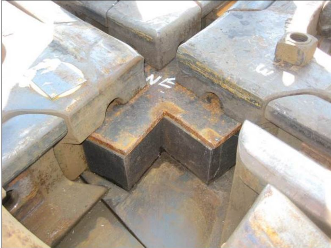
Figure 23. The solid rubber flangeway spacer tile embedded in the Getzner Type B full-coverage rail seat pad resting directly on the platework. The strike plate between the rubber tile and the bottom of the casting corners was designed to protect the rubber.
