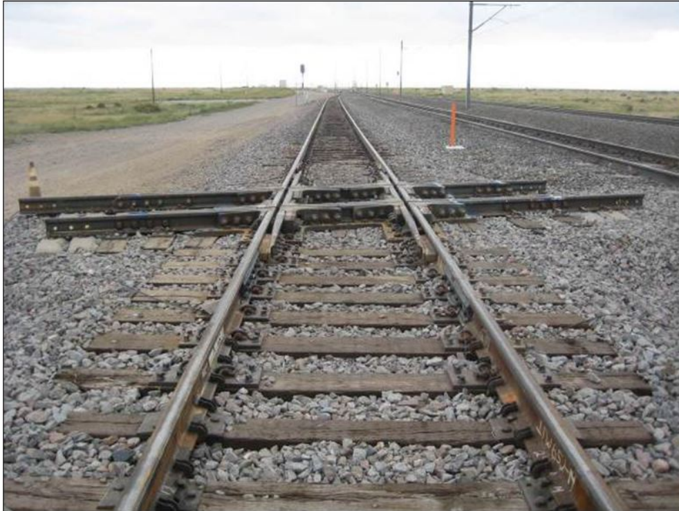
Figure 6. The crossing diamond was installed in typical HTL test configuration, where traffic runs over a single route
