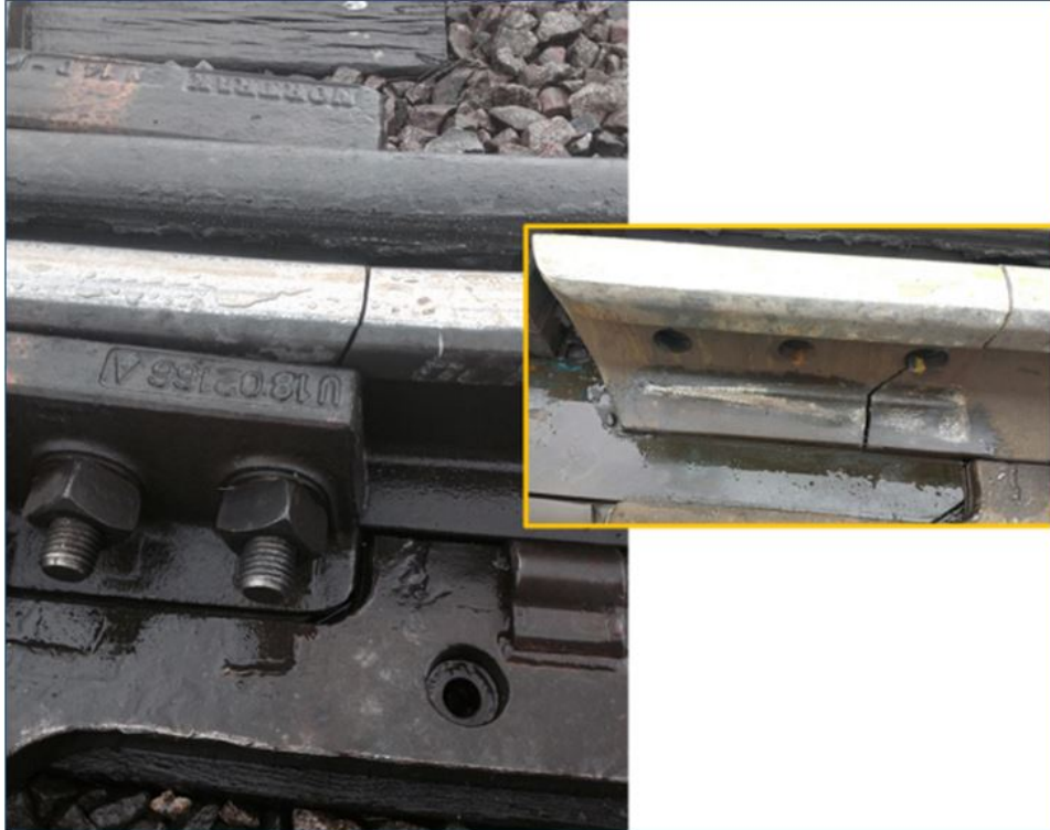
Figure 103. Wear on the top of a flangeway spacer tile where the casting corners bear
