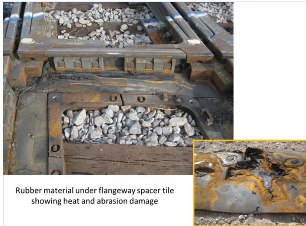
Figure 93. The full-coverage rubber pad failed to resist heat and abrasion between components. Removed after 102 laps of the HAL train
