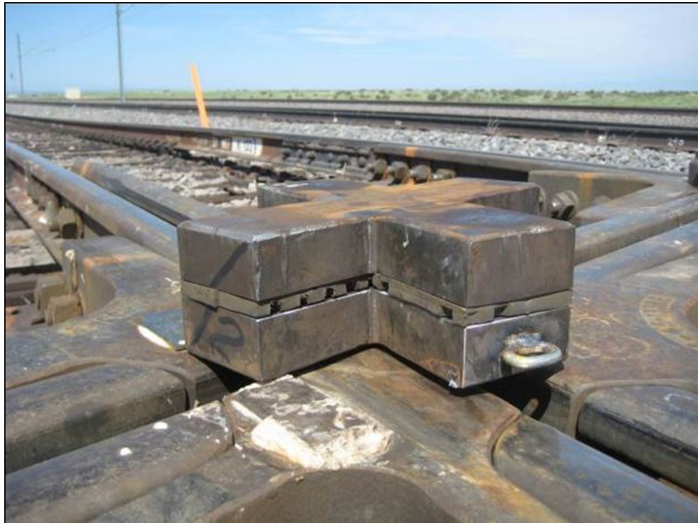
Figure 19. The steel flangeway spacer tile was cut in half and \frac{1}{4} in of material was milled from each half to accommodate a layer of the \frac{1}{2} -in Nortrak pad material
