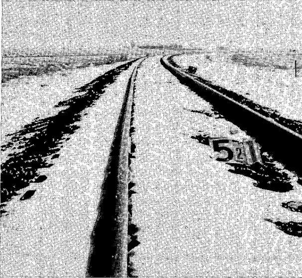
14. SECTION 5.21 - VIEW OF HIGH RAIL ALIGNMENT PERTURBATION, LOW RAIL UNPERTURBED IN ALIGNMENT
