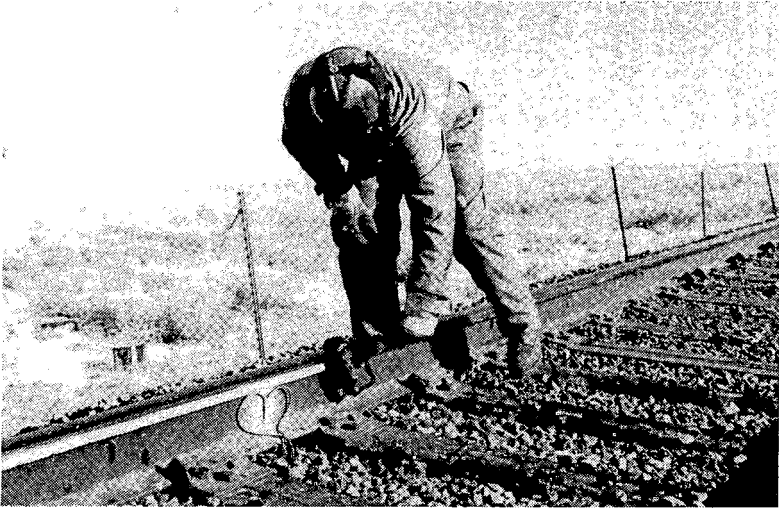
117. CLOSE-UP OF GREASED RAIL
