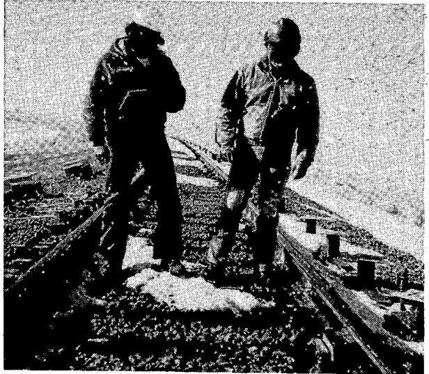
193. TRACK INSTRUMENTATION FOR FREIGHT TEST
