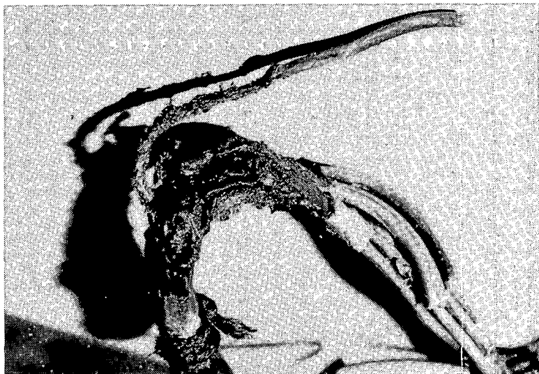
182. DETAIL OF DAMAGED WIRING AFTER REMOVAL
