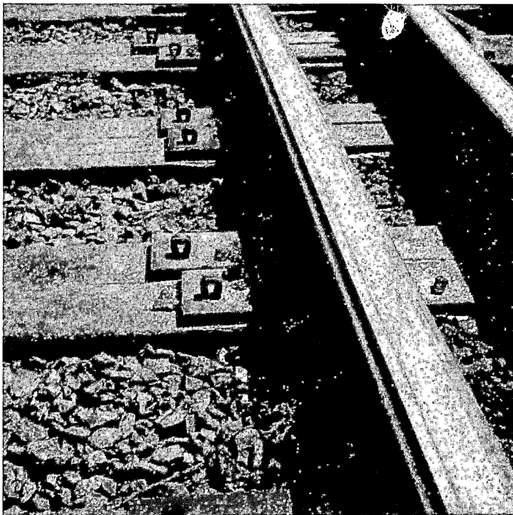
FIGURE 10-2. GAGE FACE WEAR IN AVONDALE YARD.
