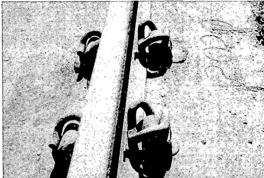
FIGURE 6-2. ADDITIONAL FASTENERS INSTALLED BETWEEN LOOSE ONES
