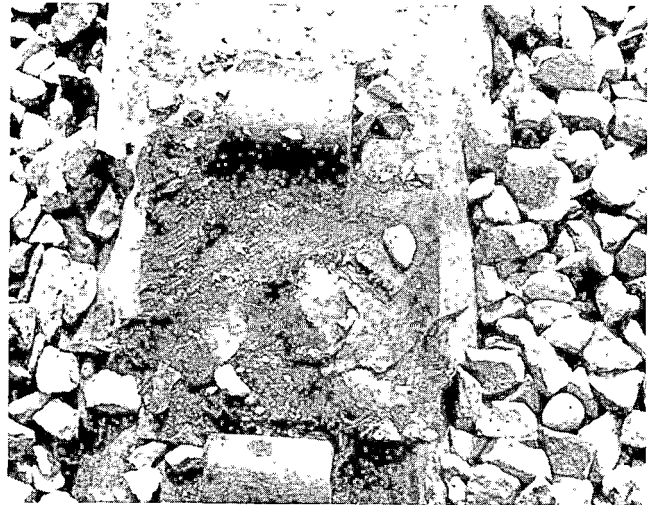
FIGURE 12. FAILED CORDED RUBBER PAD.
