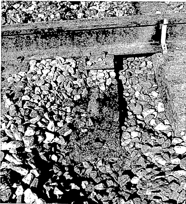
FIGURE 4. CEDRITE TIE DELAMINATIONS T-A-6.
