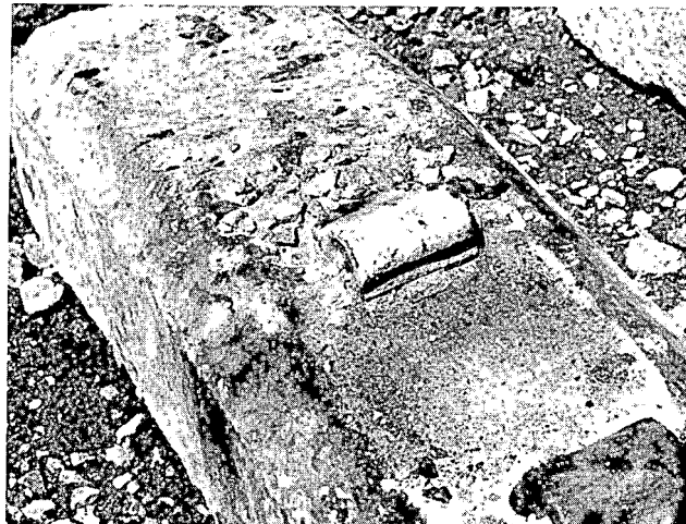
FIGURE 3. WEAR ON CONCRETE TIE EMBEDDED SHOULDER.
