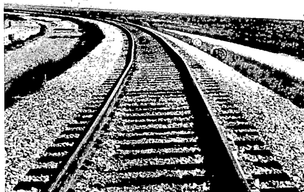
FIGURE 21. A KINK ASSOCIATED WITH WELDED RAIL END BATTER.
