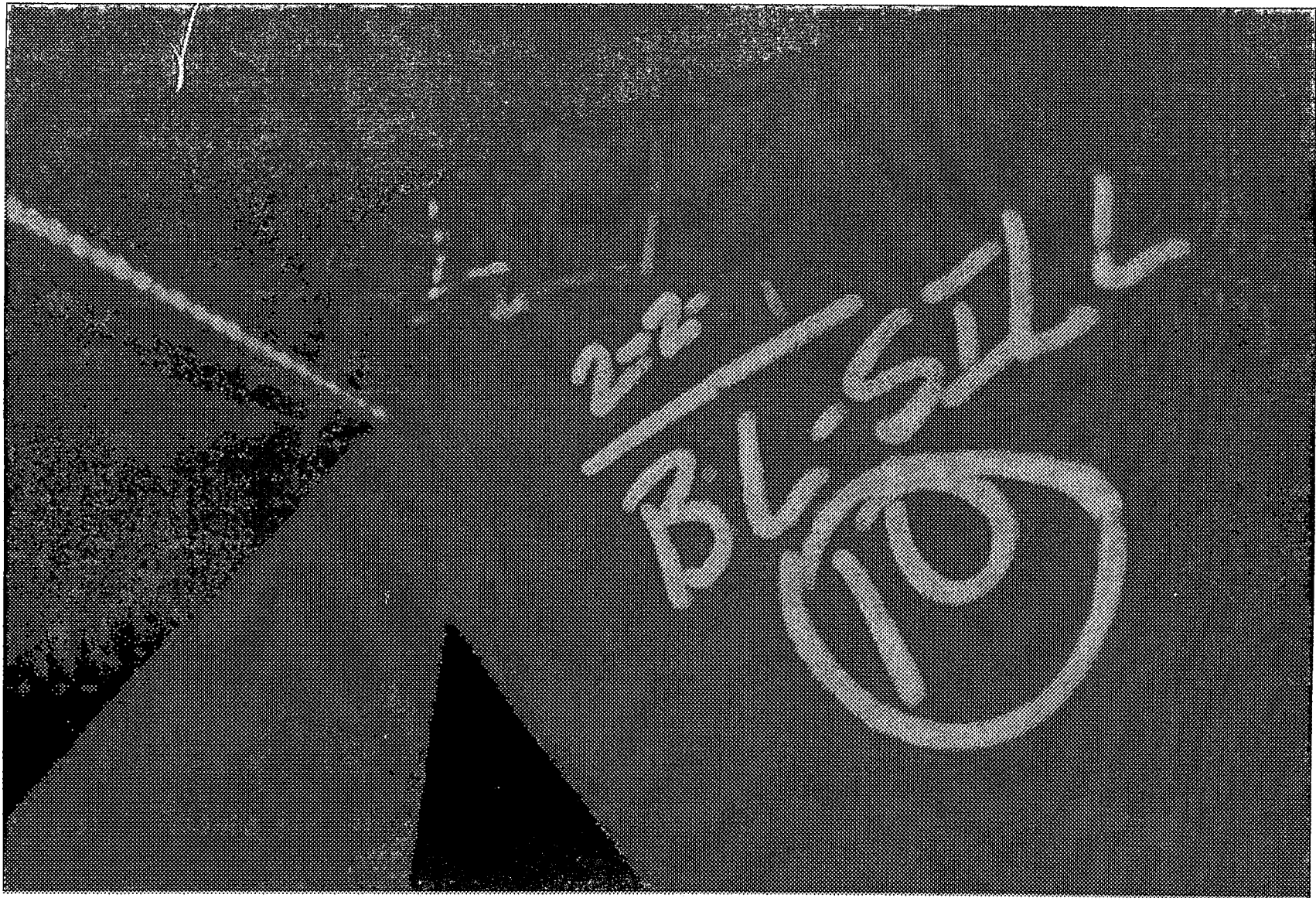
Exhibit 10.5 Photograph of Stub Sill Crack..
