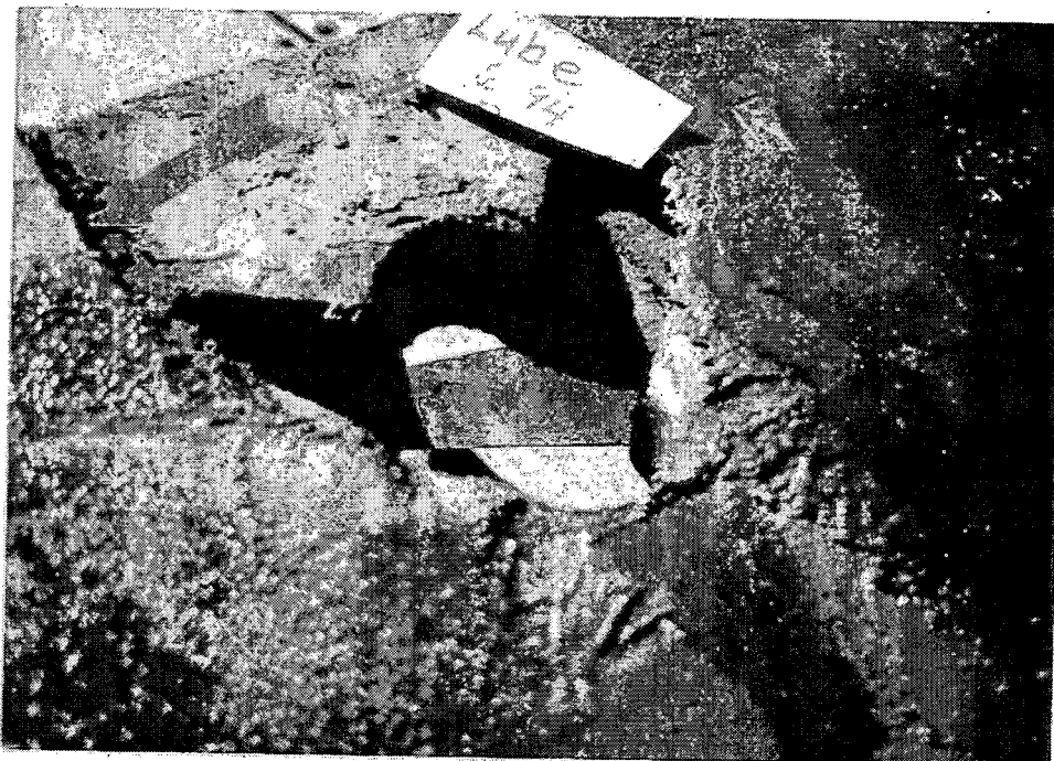
T - 21 Excessive old lubricant. Screw type hitch lubricated and inspected 6-94. No lubricant on sliding surface. Omaha, NE. 6-23-94
