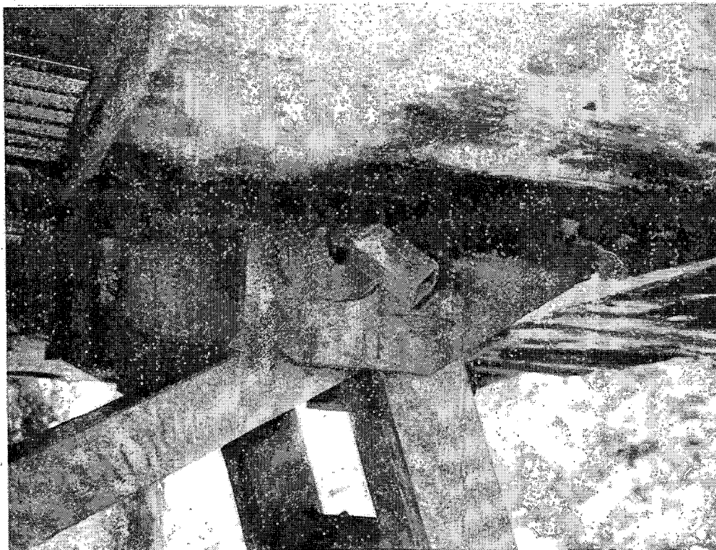
T - 4 Bent operating rod makes hitches difficult to operate. Kansas City, MO. 6-19-94
