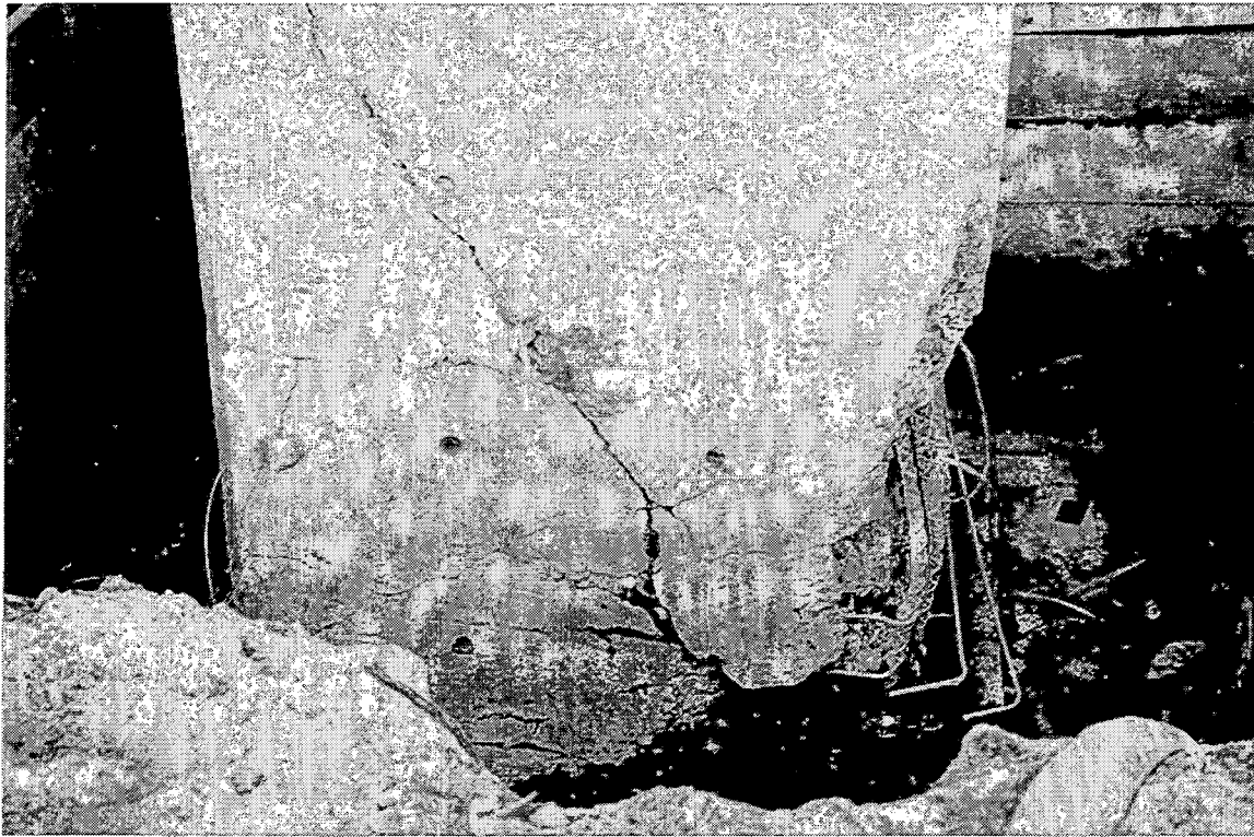
JRS-19. This column was close to failure. The ties are opening, main bars are buckled and the shear crack is opened. Note the angle of the shear crack is more vertical than 45 degrees. Response was in the longitudinal direction.
