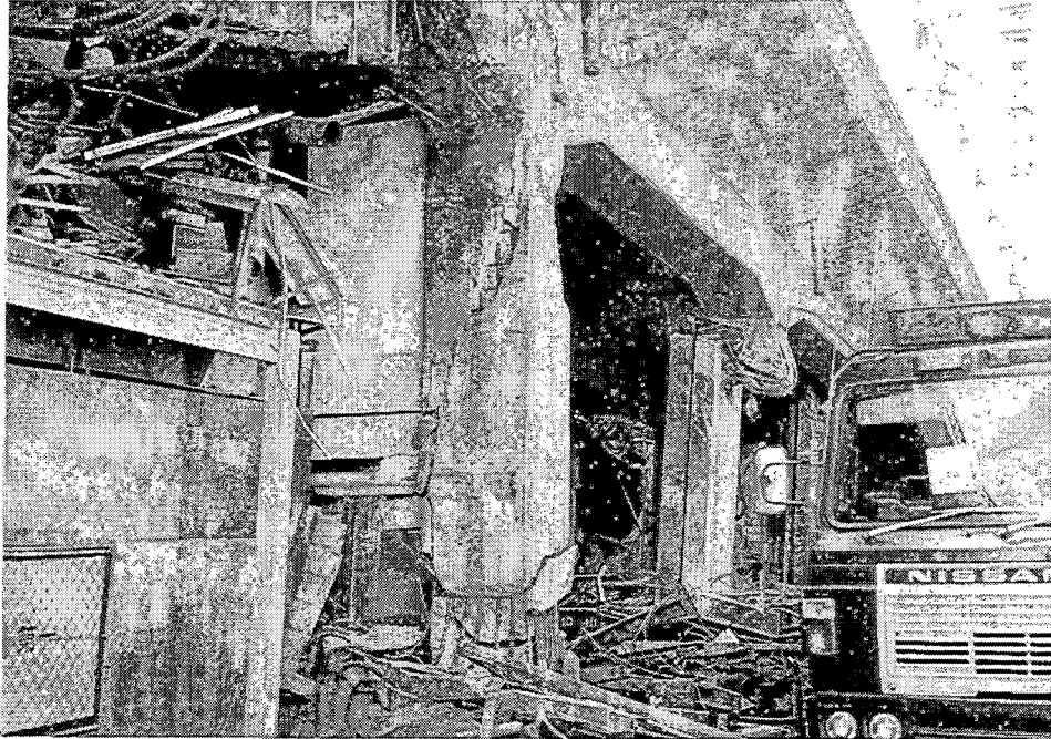
HER-19. This shear crack in the column is inclined much more than 45 degrees. Without the secondary frame system, damage extends to the footing.
