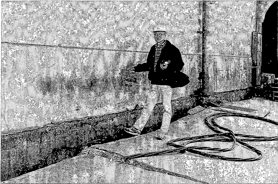
PI-7. This loading dock adjacent to the people mover displaced over 300 mm horizontally and over 400 mm vertically from the side of the warehouse.
