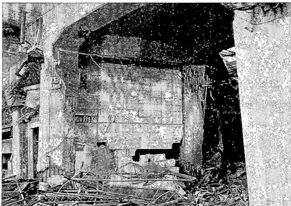
HER-22. This unreinforced infill wall did not have adequate shear capacity. Note the shear cracks in both columns at greater than 45 degree angles and the flexure damage at the base of the columns.
