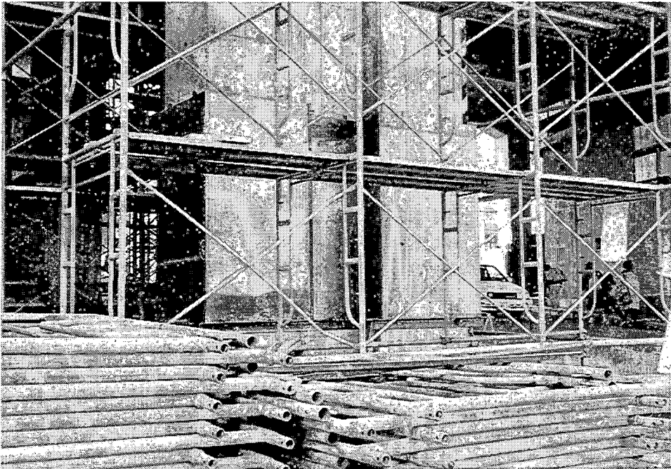
JRT-34. Unusual shaped steel plate jacket on this pier wall.
