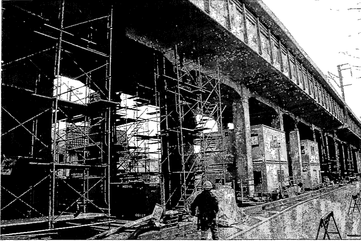
JRS-1. Many consecutive columns were damaged.
