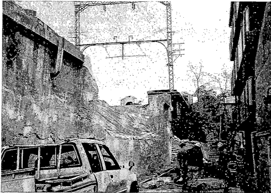
HER-5. Another section of failed gravity retaining wall; there is another failed section above the sandbags in the background. Note the horizontal crack above the parked vehicle.
