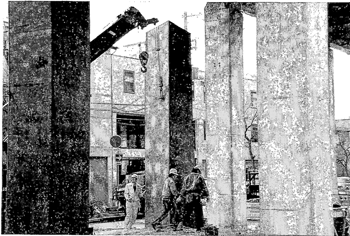
JRS-29. Steel plate jacket installation; note damage at the top of column.
