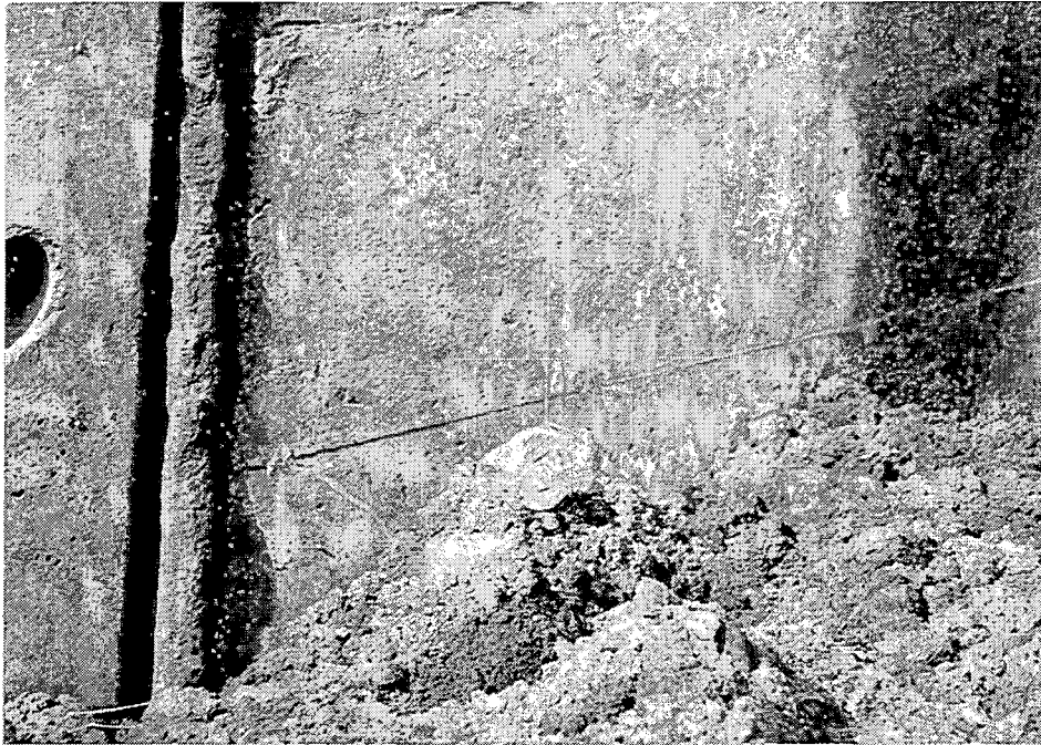
JRT-3. This concrete plumb bob indicates a 400mm lean in the retaining wall.
