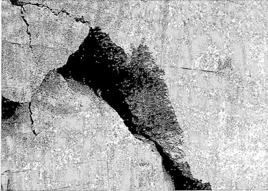
HER-9. The crack in the retaining wall shows that the wall is unreinforced concrete.
