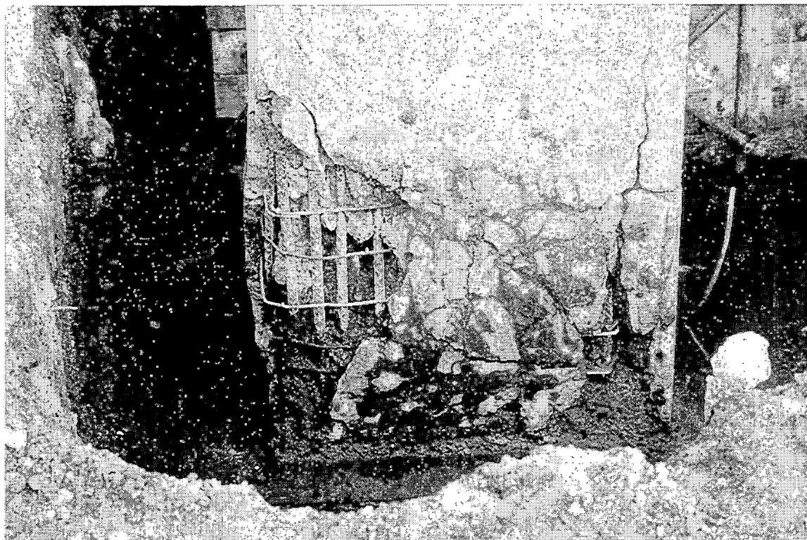
JRS-18. Some spalling is evident at the bottom of this column. Note the tie size and spacing.
