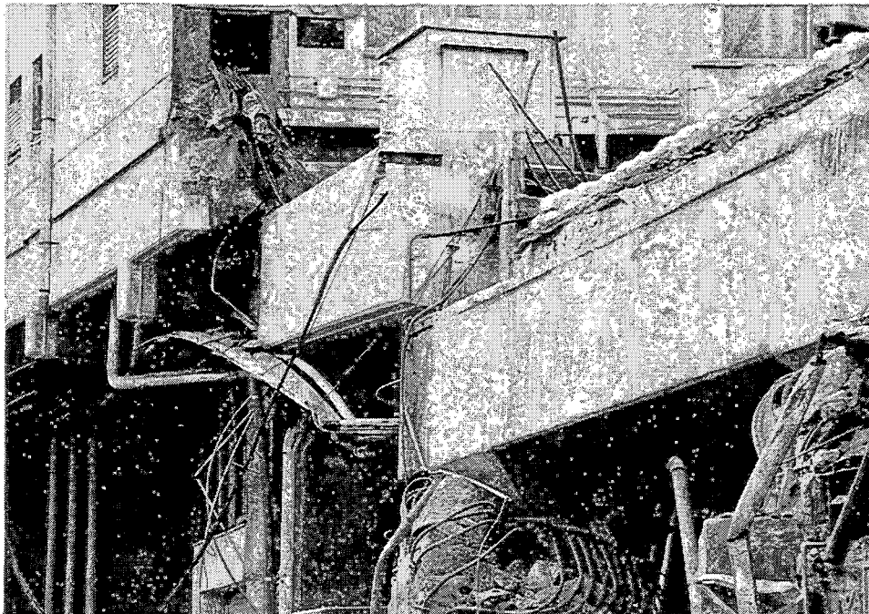
HER-18. The progressive collapse here is unusual.
