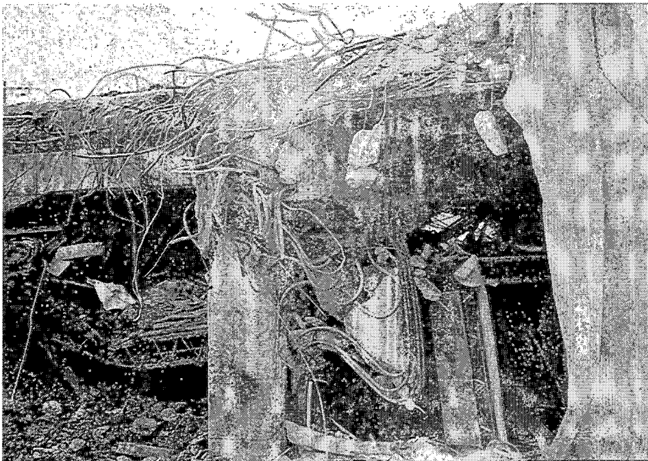
HER-10. Beginning of the failed viaduct; the steel members were used for residential and commercial buildings constructed under the viaduct.
