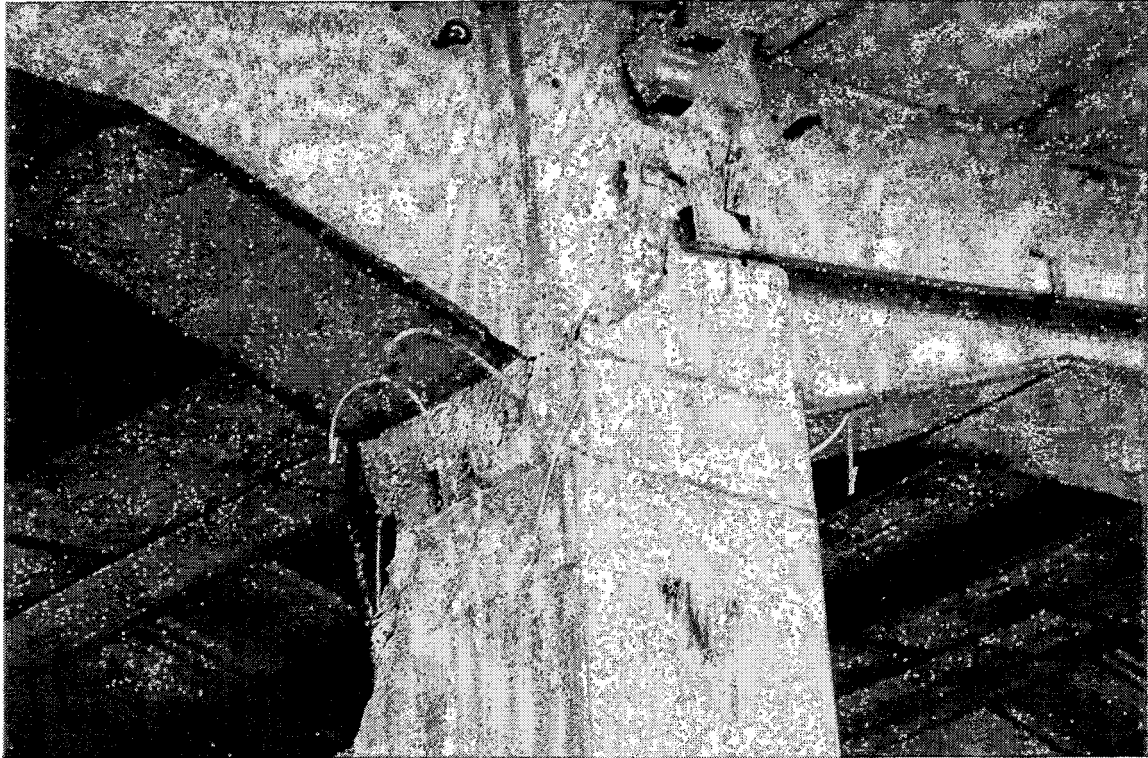
JRS-25. The cracks have been epoxy grouted. The external spalling still needs repair.
