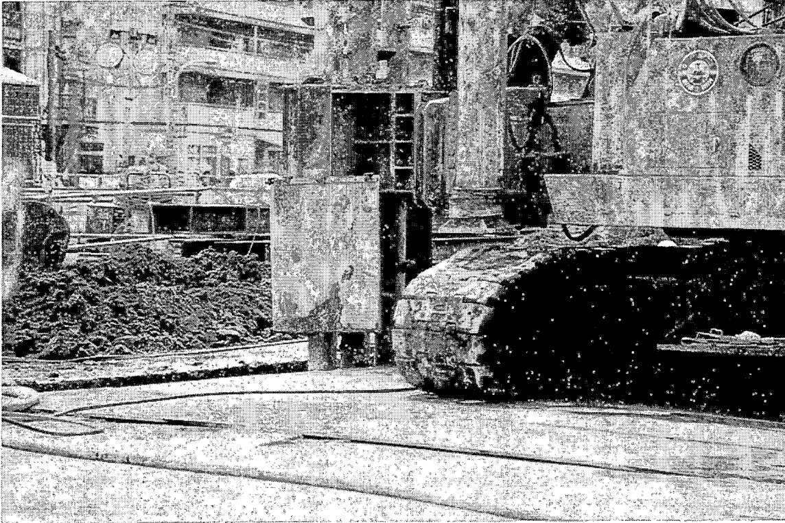
KMS-5. The contractor is constructing a soil cement wall with soldier piles to support the excavation of the station.
