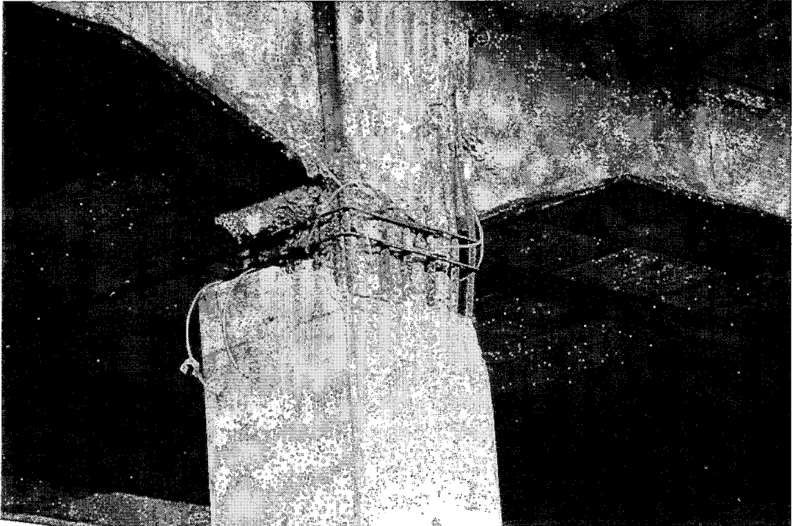
JRS-2. Another column damaged and grouted
