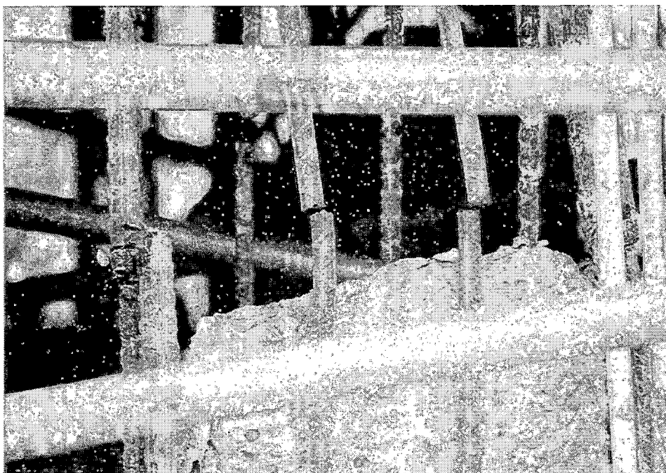
JRT-26. The center two column bars (transverse) appear ruptured while the left side (longitudinal) bars appear to have been flame cut.
