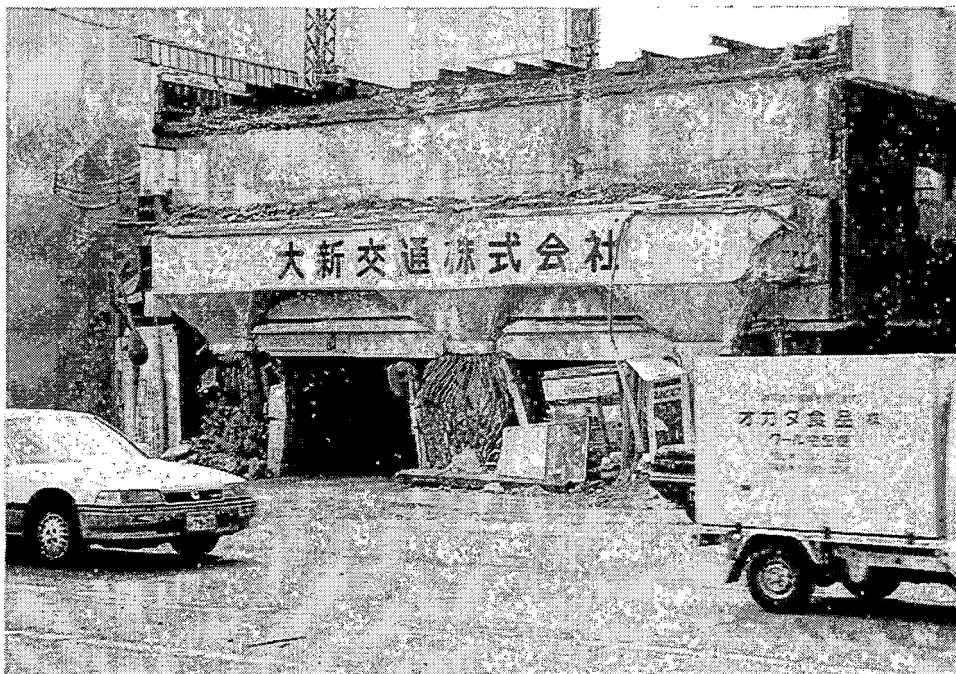
HER-12. This pier supported a steel plate girder span across the four lane street. The plate girder dropped to the street and was removed. The rails are still on the ballast on top.
