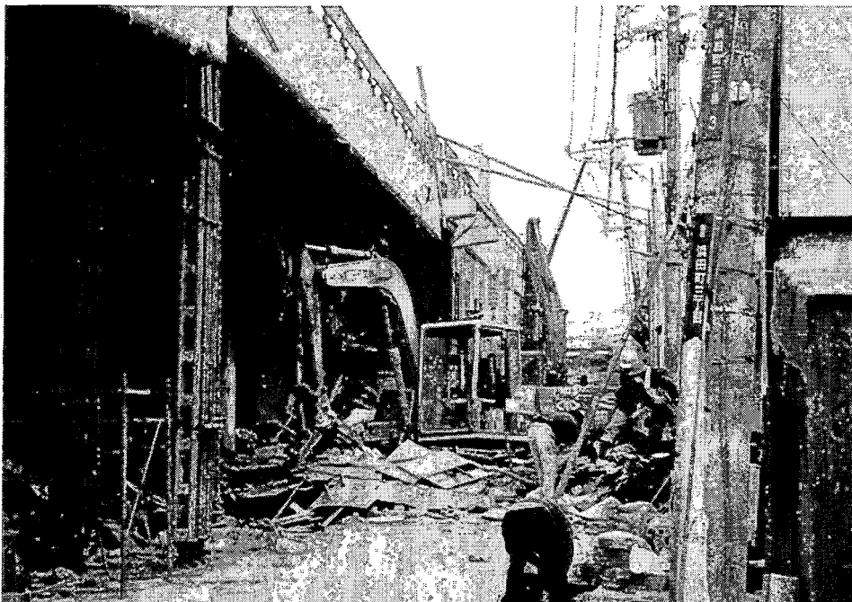
HER-27. More damage and debris is adjacent to the viaduct.
