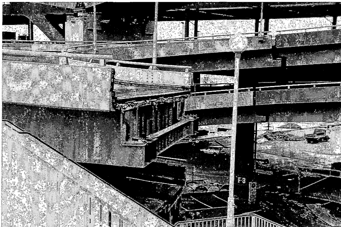
PI-14. These spans of the double deck highway bridge fell from the short span bridge seats. The arch bridge pier is at the top.
