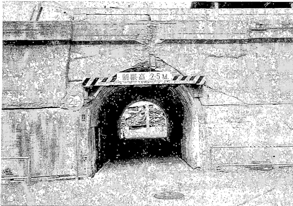
HER-6. The crown of this arch culvert shows some distress.
