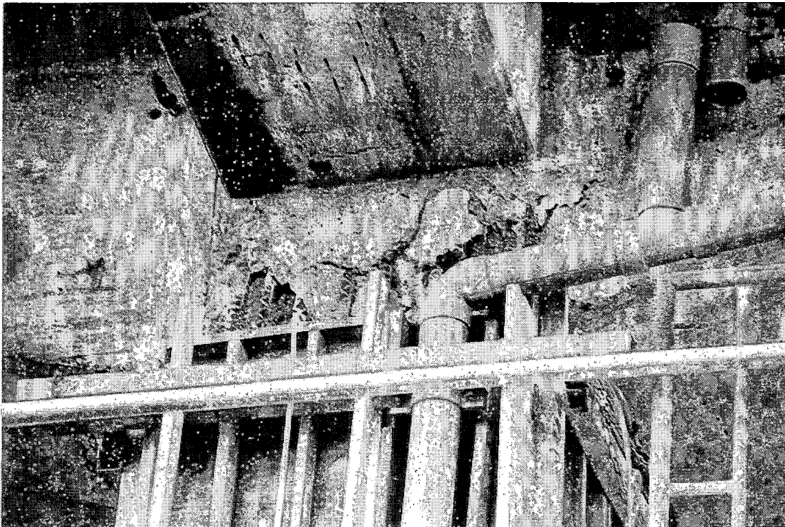
JRS-8. The cracking in this joint is limited to the zone below the confining catenary support beam at the top of the photo and the top of the column.
