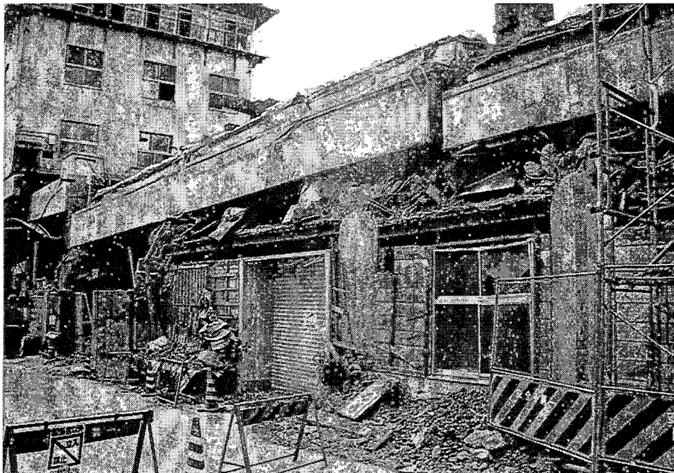
HER-16. This section is completely destroyed above the steel beams. The steel beams were installed for secondary uses of this facility. The beams seem to have concentrated the damage at the tops of the columns. This section was some sort of siding ending at the building.
