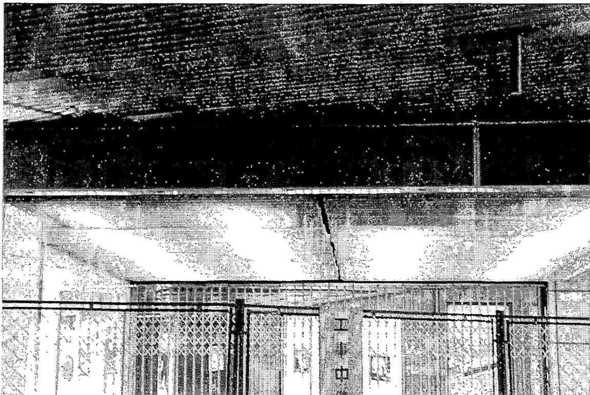
SS-6. This access to Kobe Municipal Subway Sannomiya Station is closed.
