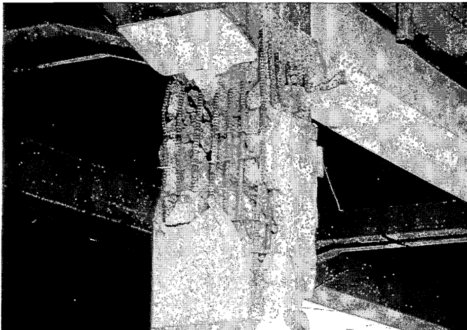
HER-32. Damage to a column west of Shinzaike Station; major transverse shear cracking and longitudinal spalling are evident.
