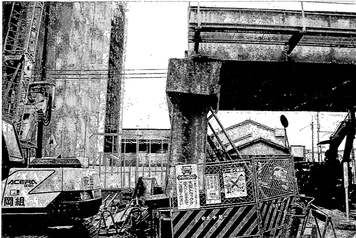
HC-9. The pier wall supporting this steel through girder is leaning significantly only at this end indicating the bearings slipped. The adjoining concrete structure was removed entirely.
