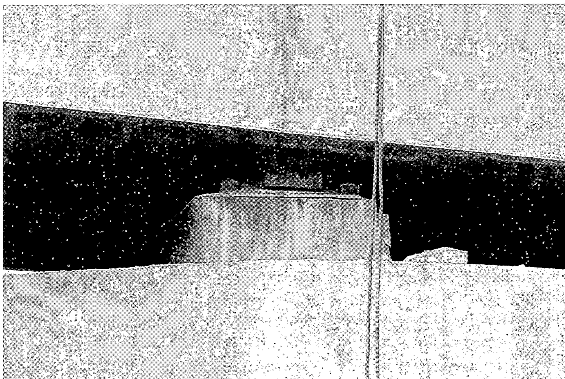
PI-18. A close-up of the the isolation bearing
