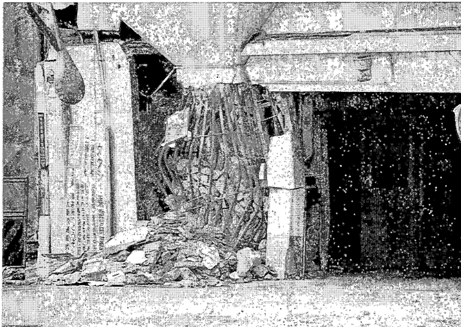
HER-14. Close up of the left column of the pier. The structure has not settled much with respect to the door inside the garage. The glass in the door appears intact. This column shows a few ties were present.
