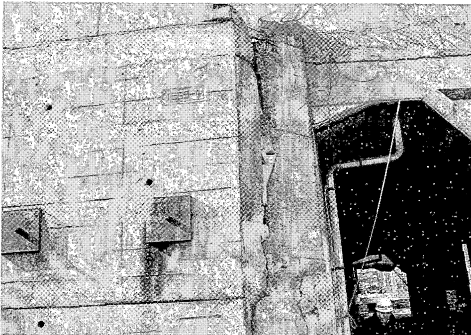
JRT-2. The failed retaining wall opened at this abutment.
