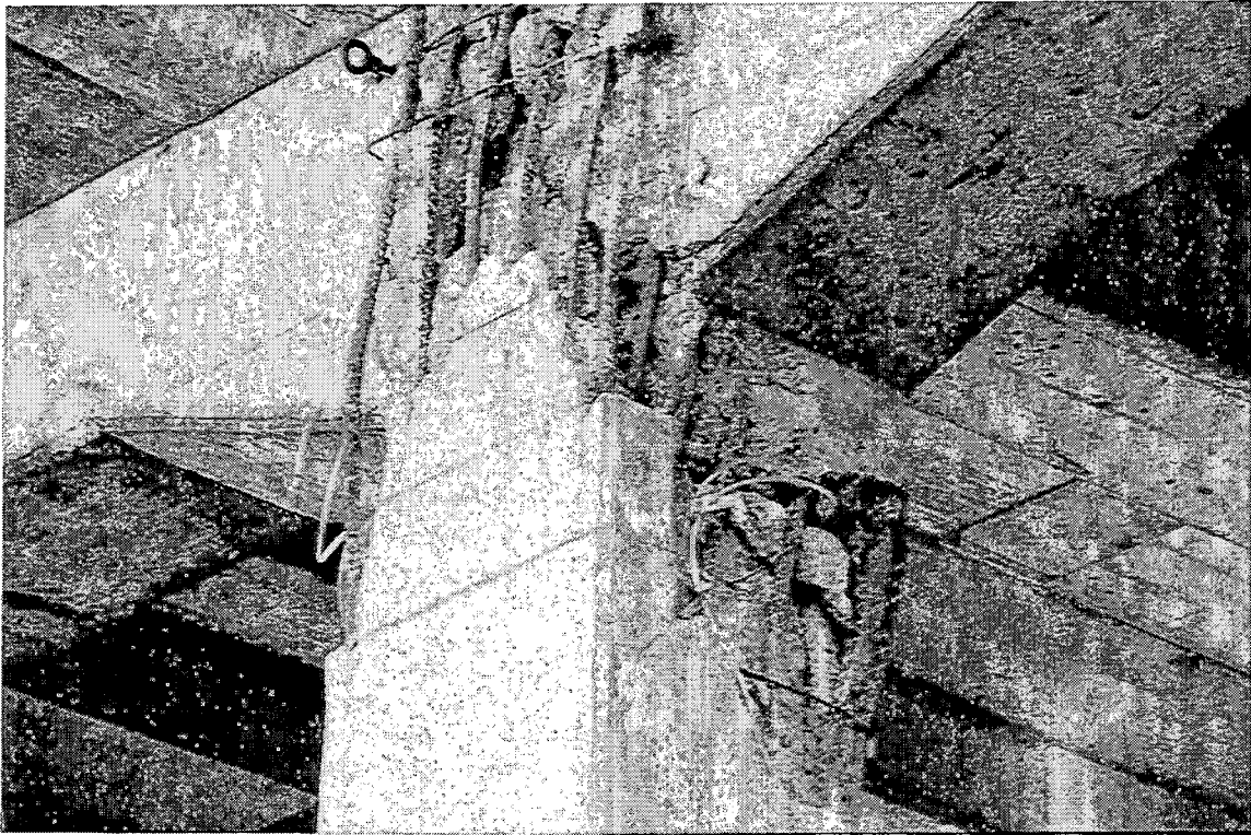
JRS-5. Column very close to collapse with diagonal cracks through the joint zone and ties ruptured; the joint is badly deteriorated.
