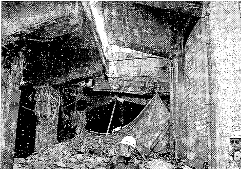
HER-20. The masonry infill wall on the right seems to have helped by increasing shear capacity. Note the expansion joint at mid span and the adjoining parallel structure in the background.
