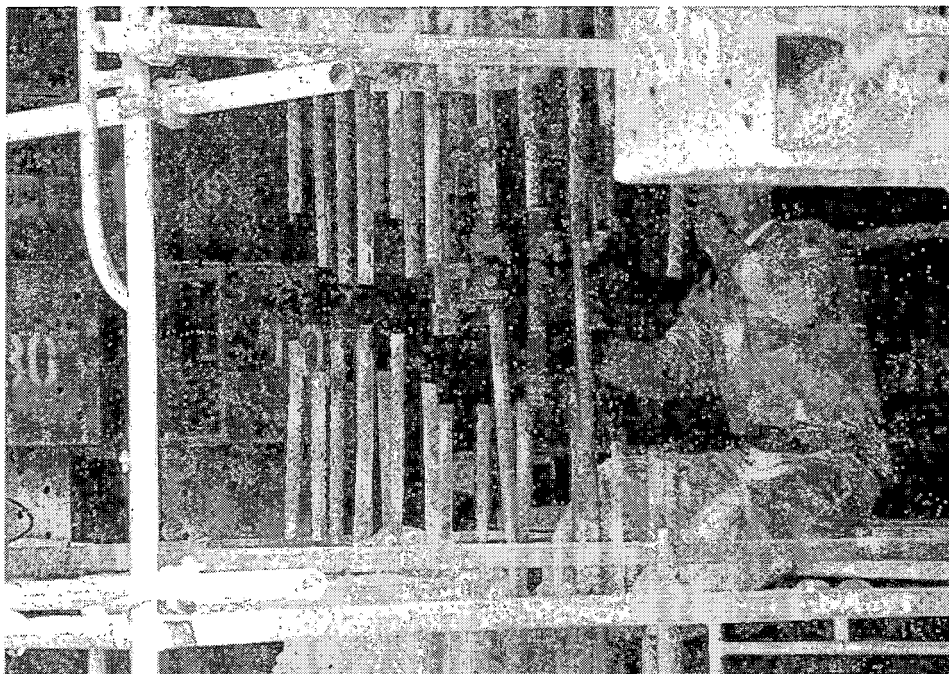
JRT-25. An ironworker is splicing new rebar in this column about 500mm below the top of column.
