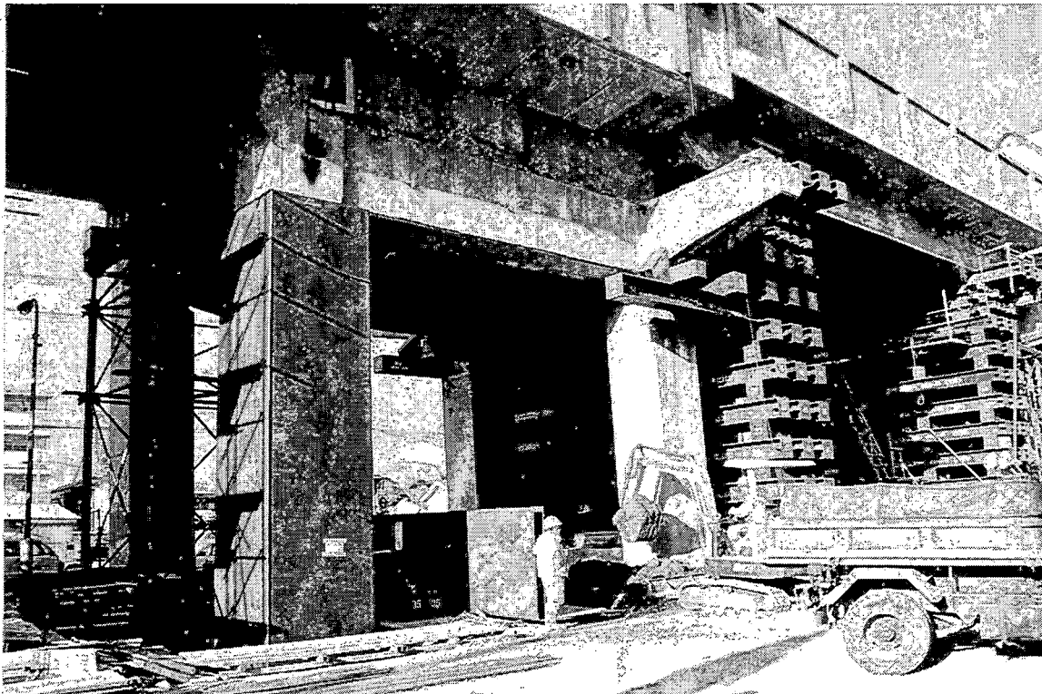
JRS-20. The drop in span on the right was lifted off the ground and relocated on the piers. The adjacent spans were stiffened with the additional girder. Steel jackets were applied to columns.
