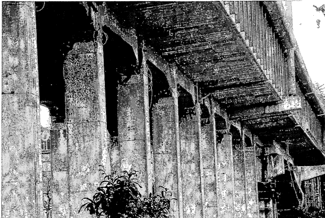
JRS-28. Longitudinal response is shown by the damage in consecutive columns. There is minimal transverse damage.
