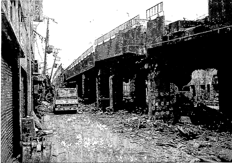
HER-25. Broken columns and disjointed superstructure will require demolition.
