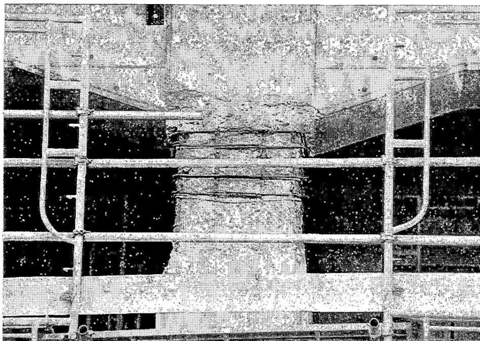
JRT-31. A plastic hinge started to form at the top of this column. Additional ties and a vertical stirrup are being added.
