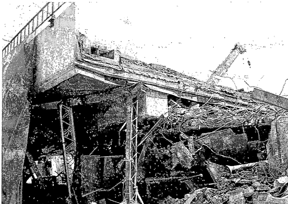
HER-11. The viaduct collapsed to the left of the expansion joint but was destroyed to the right. The joints were located at midspan. The ballasted rail provided no restraint.
