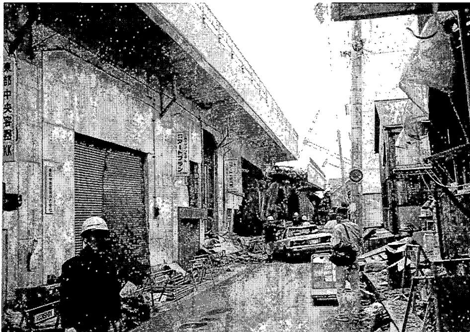
HER-21. The secondary framing and shear walls have had a very positive impact on this frame. The rubble and debris starting up the street prohibited our access and observation for the next three or four blocks.
