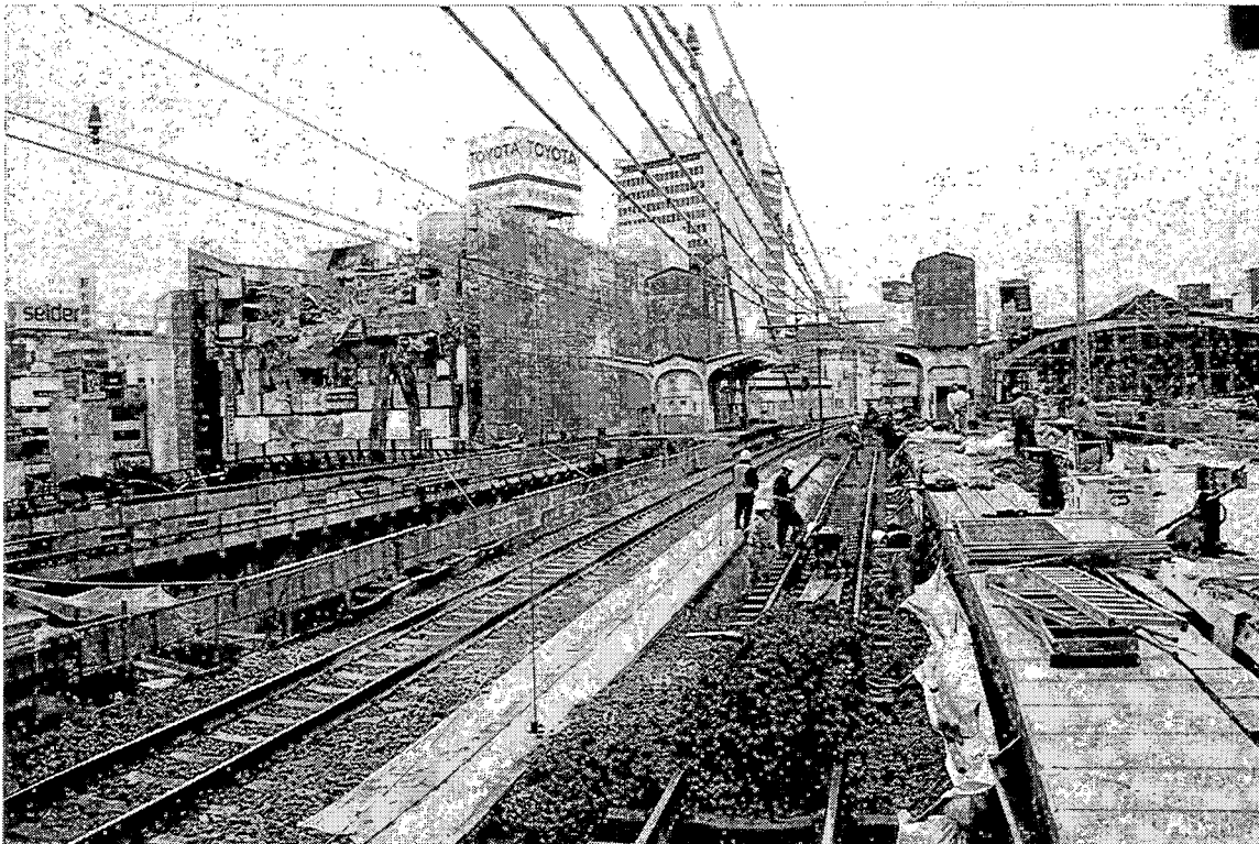
SS-2. The ballast is being replaced and recompactd on the westbound track. Note the damage to the building to the left.
