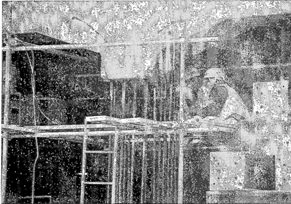
JRT-17. New column reinforcing is being welded to existing bars to repair damaged columns.
