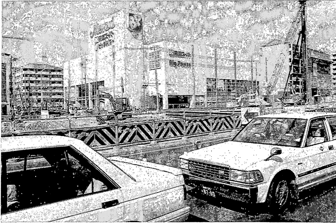
KMS-7. The buildings in the neighborhood of the failed station suffered minimal damage.
