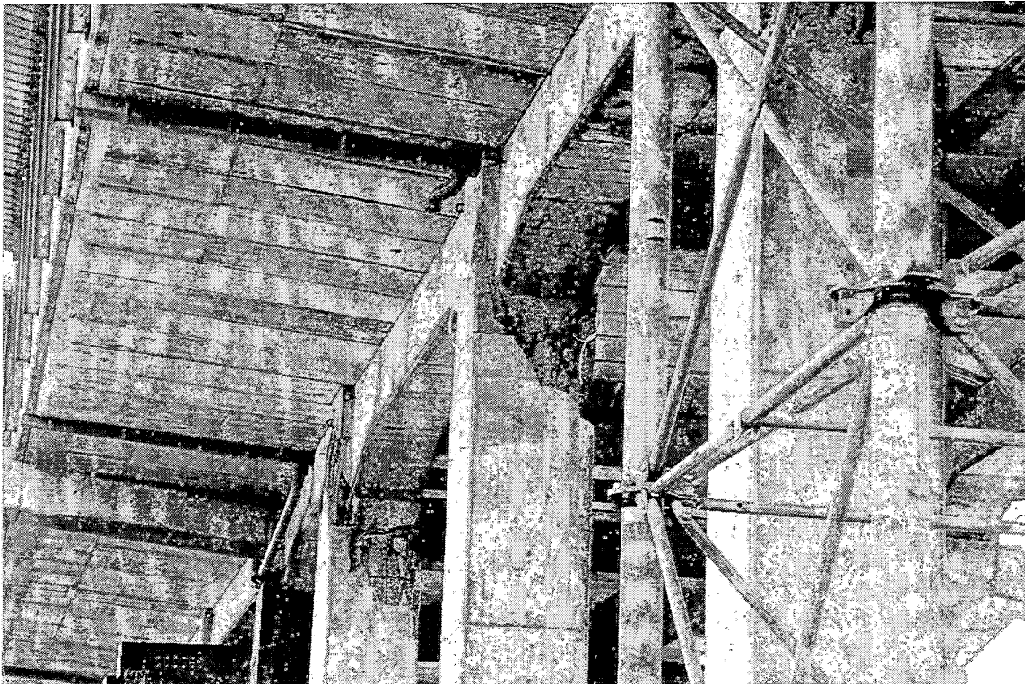
JRS-4. These columns show primarily transverse damage, but also some horizontal spalling.
