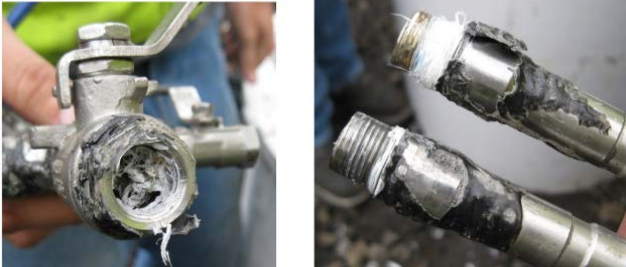
Figure 14. Damaged Tubing Ends
