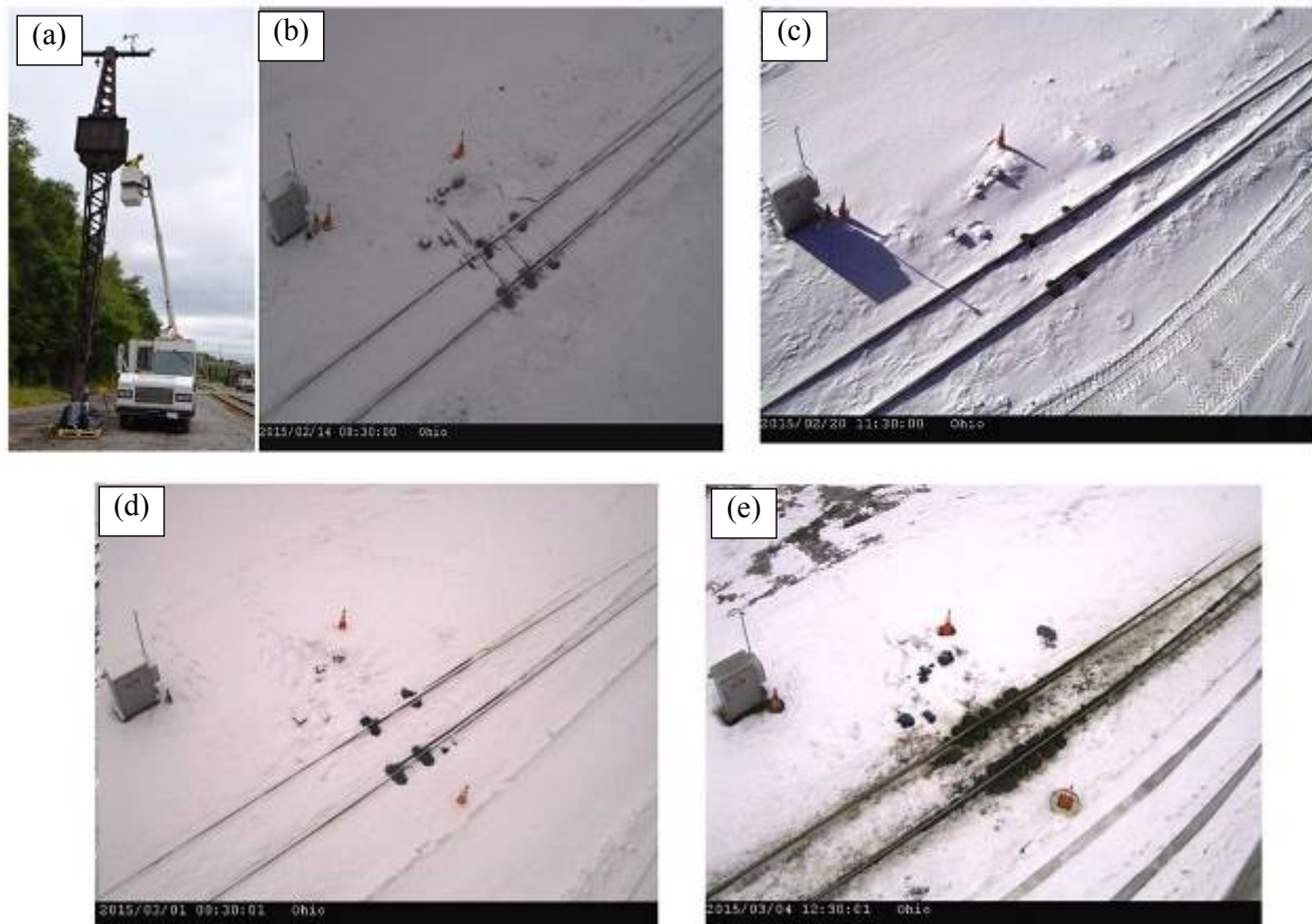
Figure 30. (a) Overhead Camera and Anemometer Setup on Old Catenary Tower (b) Feb. 14, Initial Overhead Photos show five Switch Plate Heating Systems Working (c) Feb. 20 after heavier snow (d) Mar. 1 system still working (e) Mar. 4, switch plates are clear
