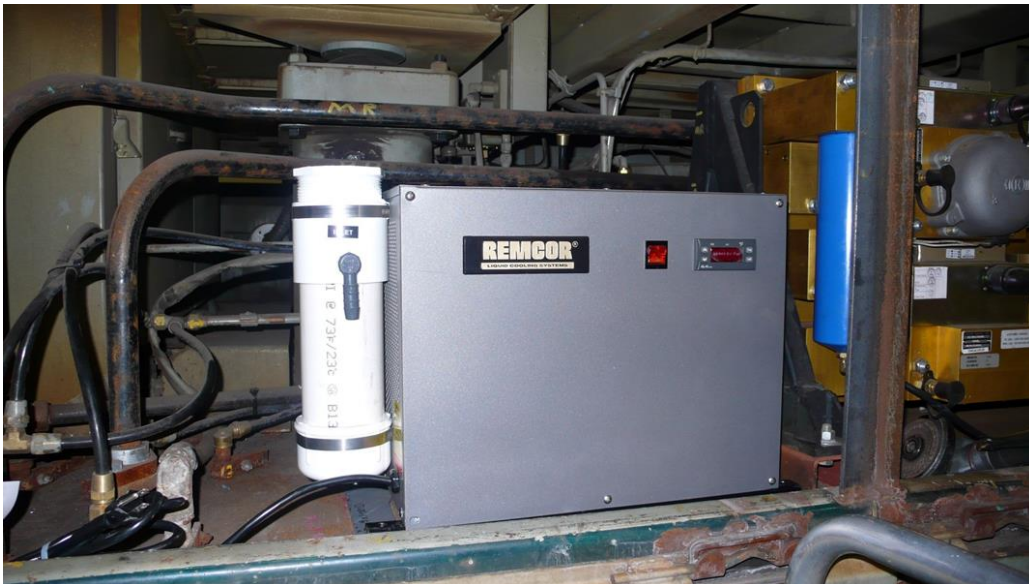
Figure 6. Chiller unit installed in the vestibule below the cab floor
