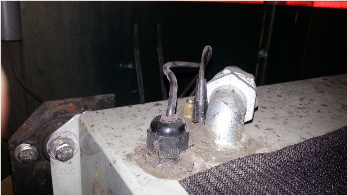
Figure 32. Broken cell phone antenna cable joint found outside the electronics control box
