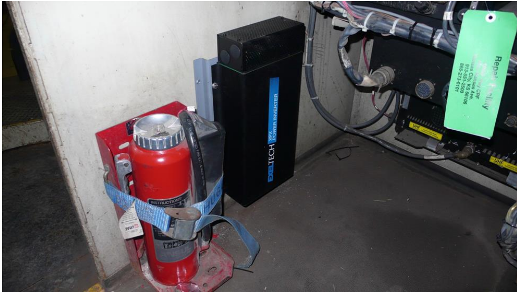
Figure 7. Wall-mounted Power Inverter installed
