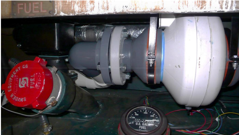
Figure 4. Exhaust pipe attachment to the fan outlet
