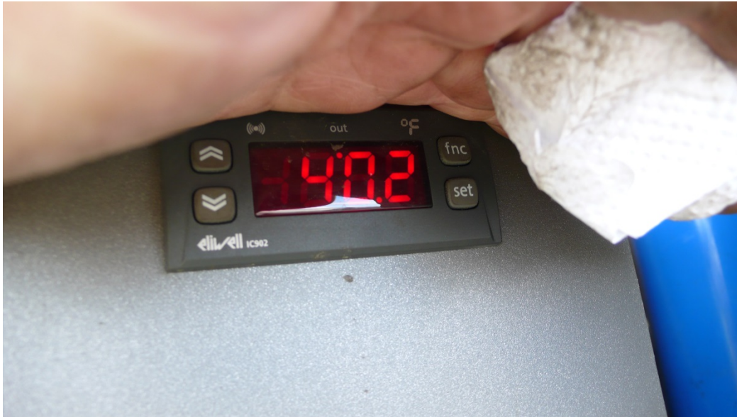
Figure 22. Chiller display showing status of circulating coolant temperature
