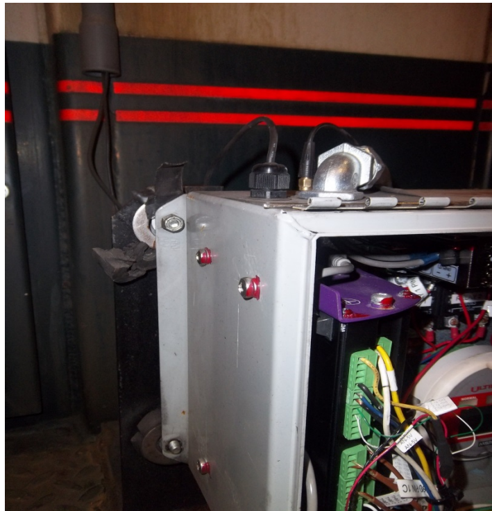
Figure 24. New Data Taker module installed inside the electronics control box
