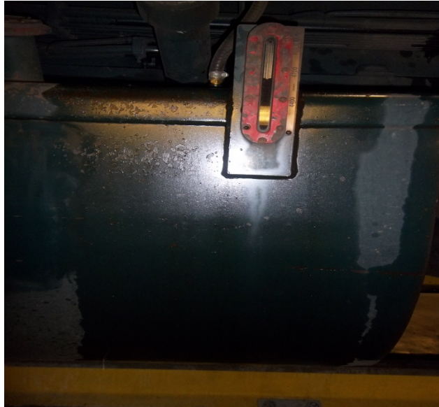
Figure 25. Evidence of fuel overfill during tank refueling
