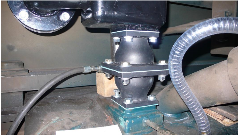
Figure 2. Modified vent pipe with float valve fitting
