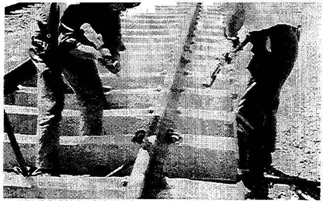
Fig. 6. B-66 ties with Pandrol fasteners at Noble, Illinois.
