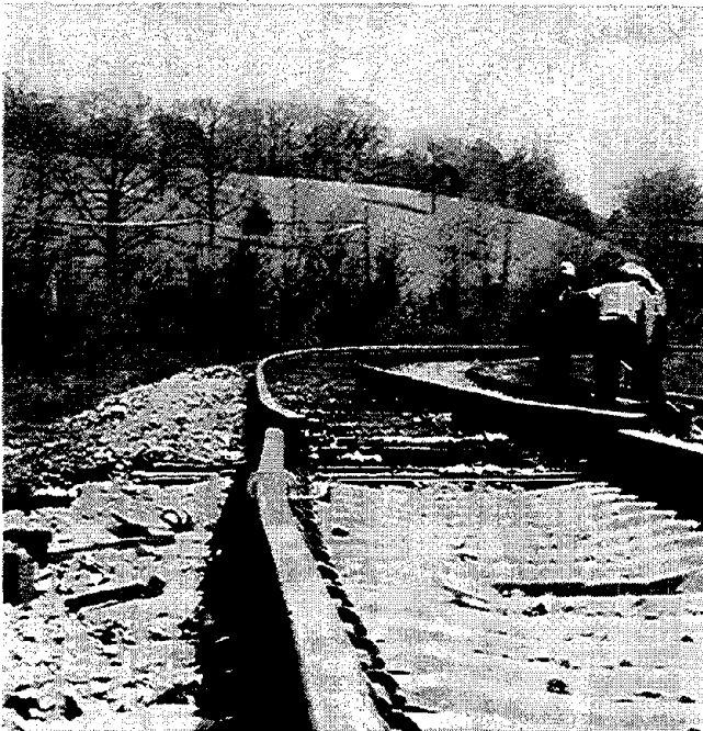
Fig. 18. Displaced concrete tie panel.
