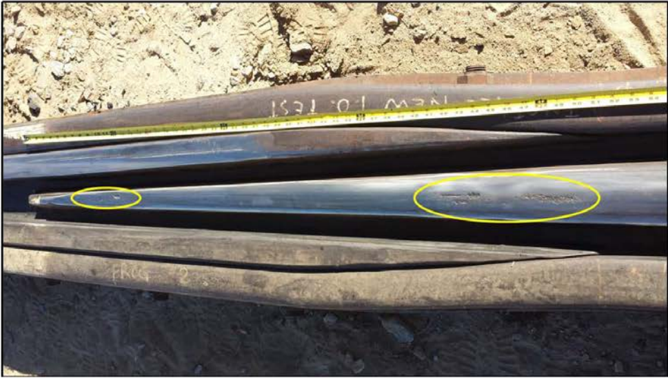
Figure 18. Final inspection: Running surface spalls developing on the frog point
