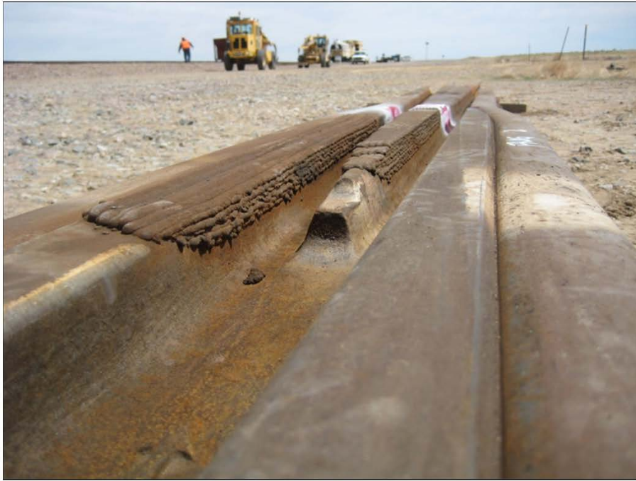
Figure 2. Frog 2: Wing rail repair about 36 inches long; point repair about 43 inches long
