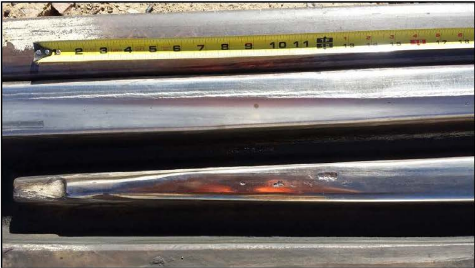
Figure 19. Final inspection: Close-up of running surface spalls developing on the frog point
