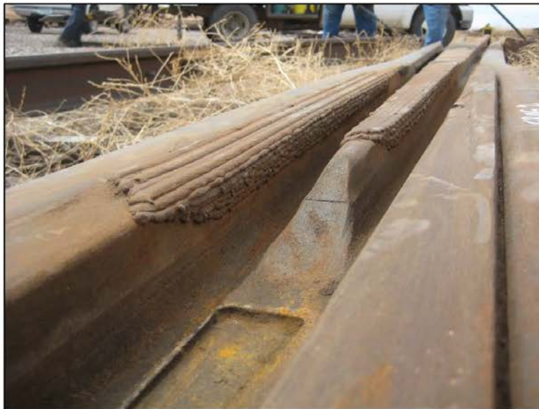
Figure 1. Frog 1: Wing rail repair about 36 inches long; point repair about 48 inches long
