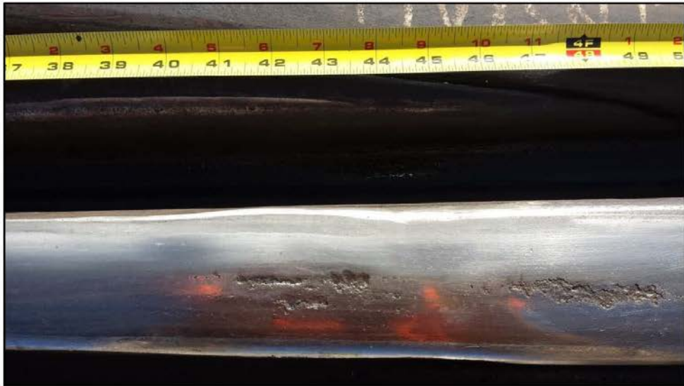
Figure 20. Final inspection: Close-up running surface spalls developing on the frog point
