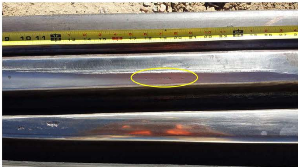
Figure 21. Final inspection: Minor running surface pitting on the wing rail
