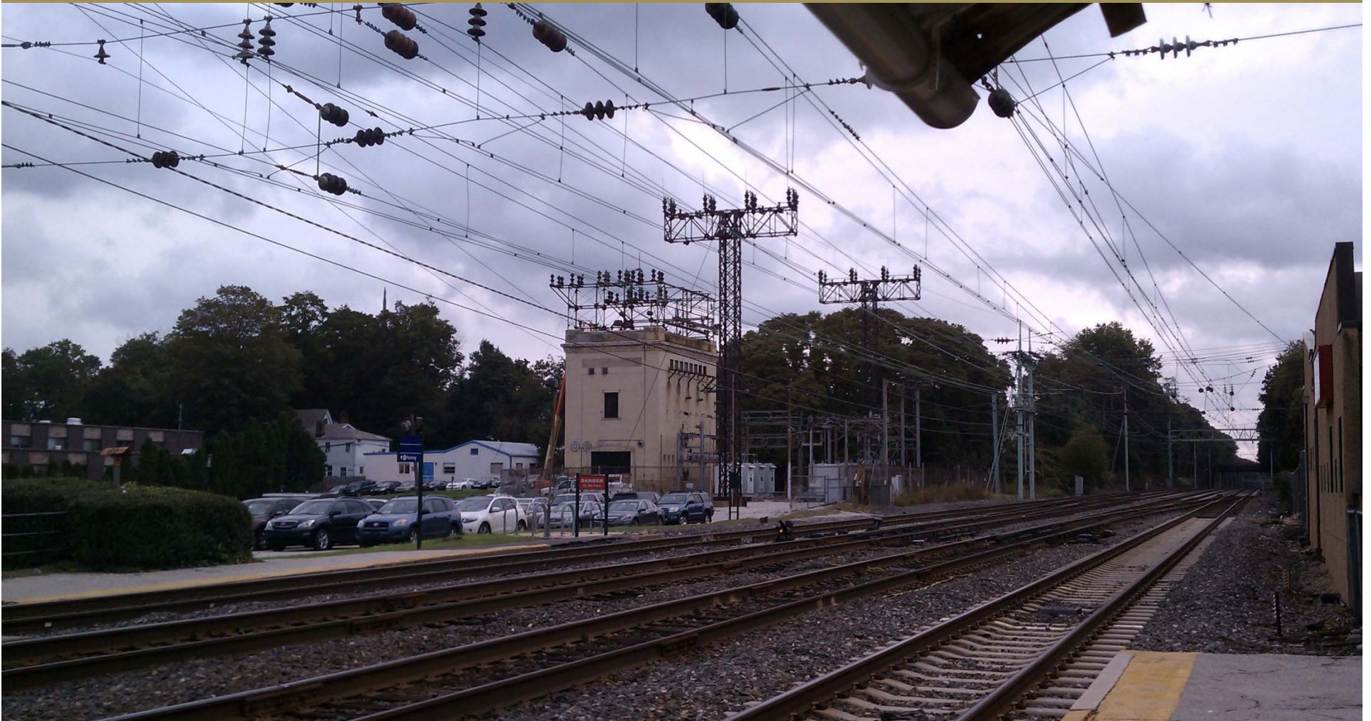
Existing Bryn Mawr Substation
