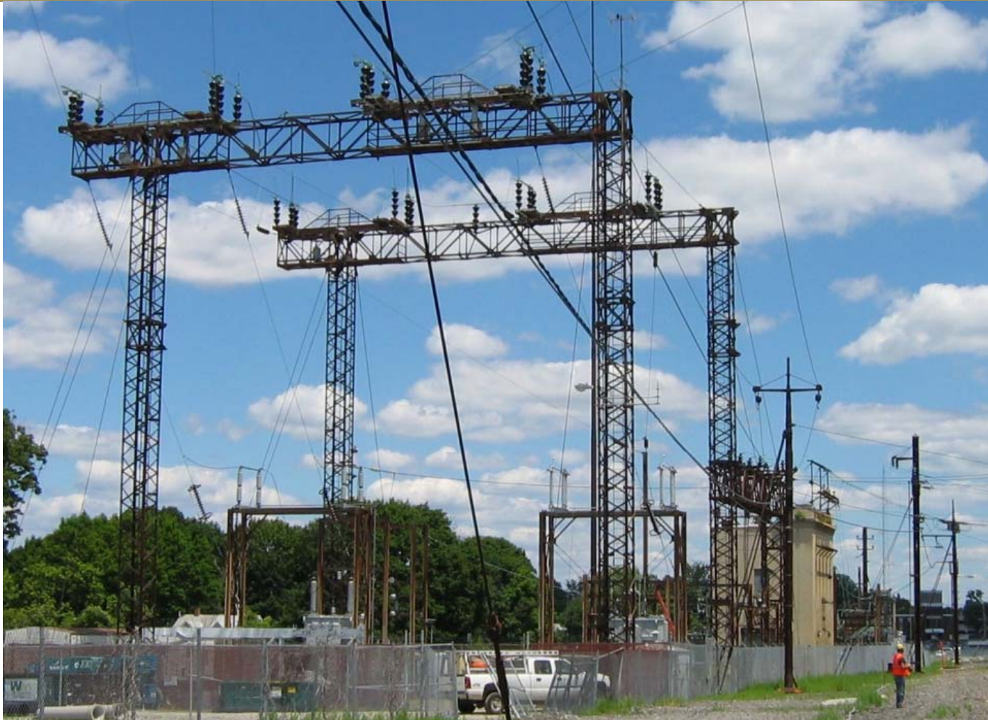
Paoli Substation, 138 kV Structures
