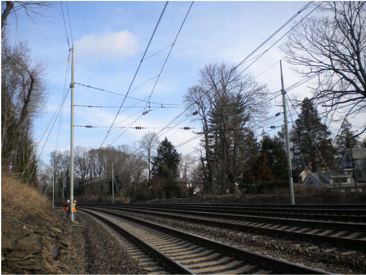
Figure 3 - Existing Catenary Structures
