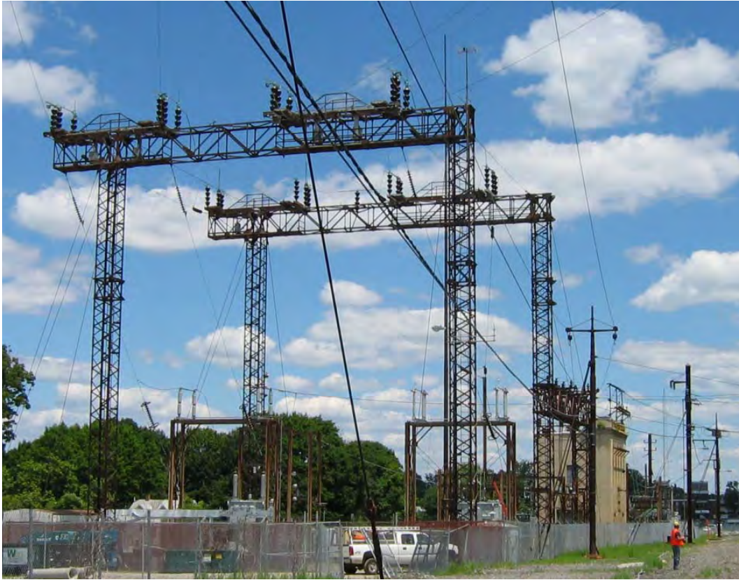
Figure 6 - Paoli Substation, 138 kV Structures
