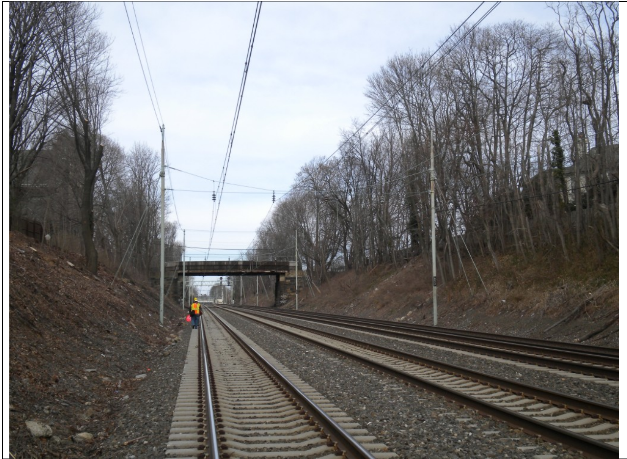
Photograph 1: Harrisburg Line, milepost 9.73, west of Haverford, looking west at existing structure P-87. Pennswood Road Bridge is in the background. HSHD is on the left, the south side of the railroad. Photograph taken 12/5/2012.
