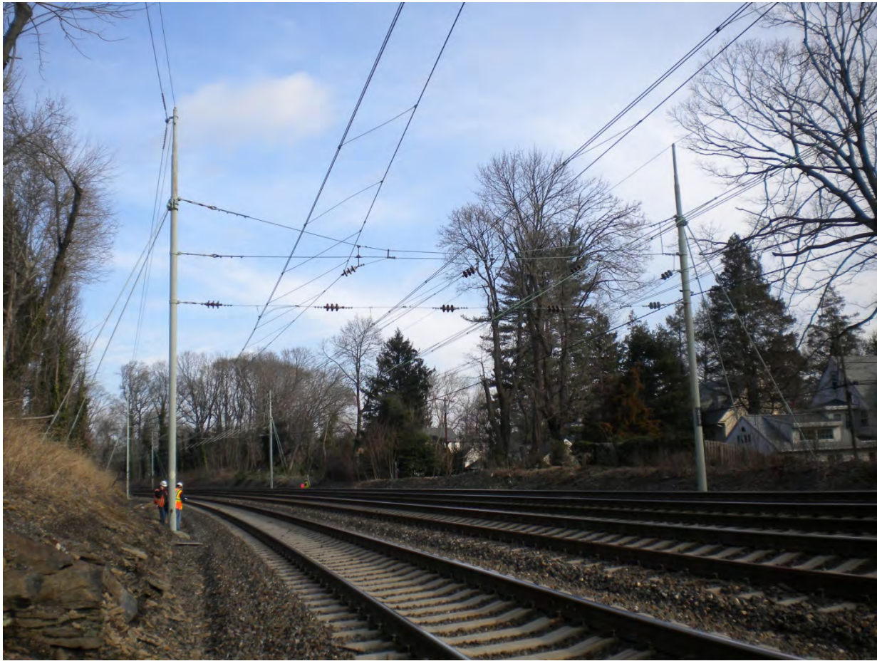
Figure 3 - Existing Catenary Structures
