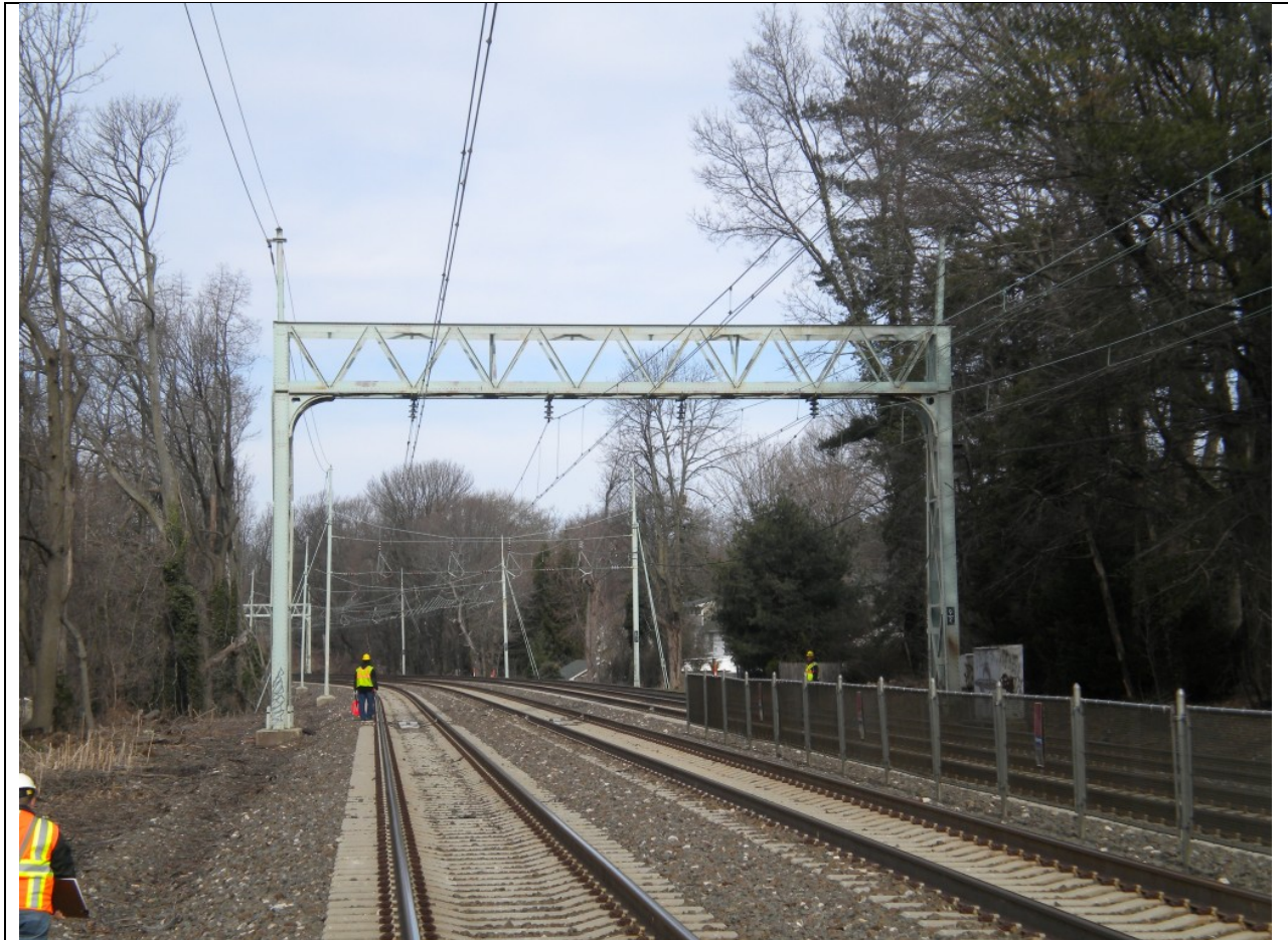
Photograph 9: Harrisburg Line, milepost 9.28, west of Haverford, looking west at existing structure P-79. HSHD is on both sides, north (right) and south (left) of the railroad. Photograph taken 12/5/2012.
