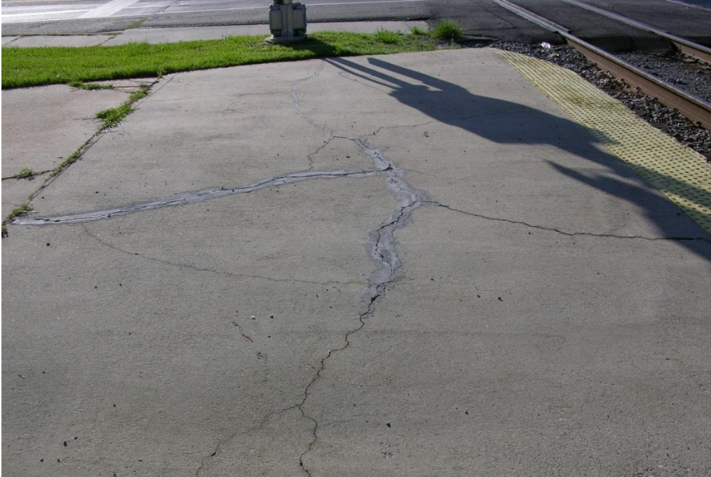
FIG TLH.21 – Cracking at edge of platform adjacent to Railroad Avenue
