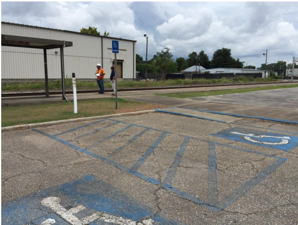
FIG BIX.12 – ADA parking spaces
