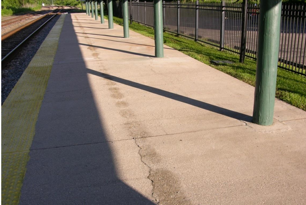
FIG TLH.19 – View of minor cracking on platform surface (looking northwest)
