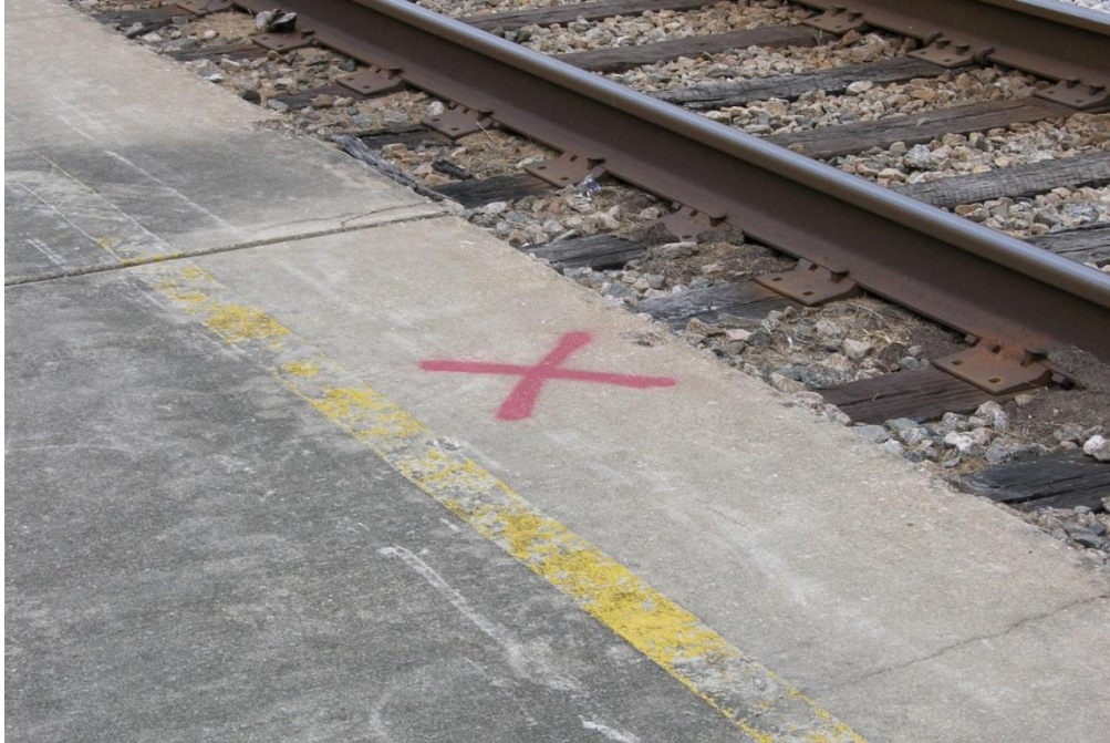
FIG BIX.11 – Tactile edge needs replacement
