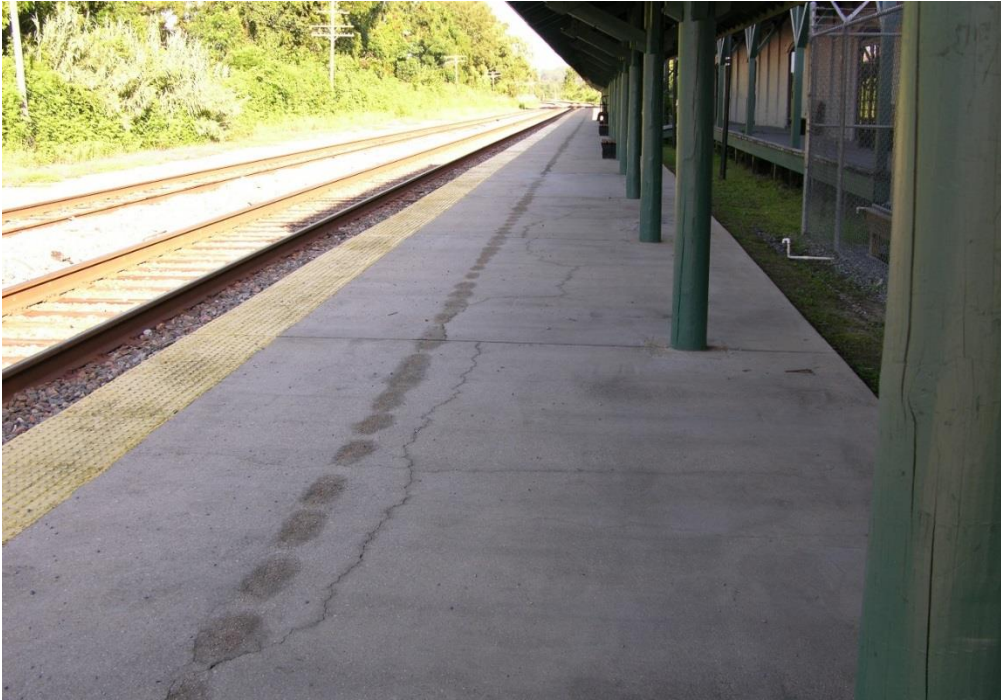
FIG TLH.22 – Minor cracking of platform surface on eastern end of platform
