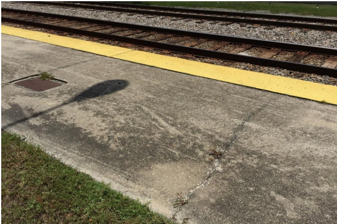
FIG LAC.05 – The platforms walking surface has minor cracks that need to be patched for Lake City FL station
