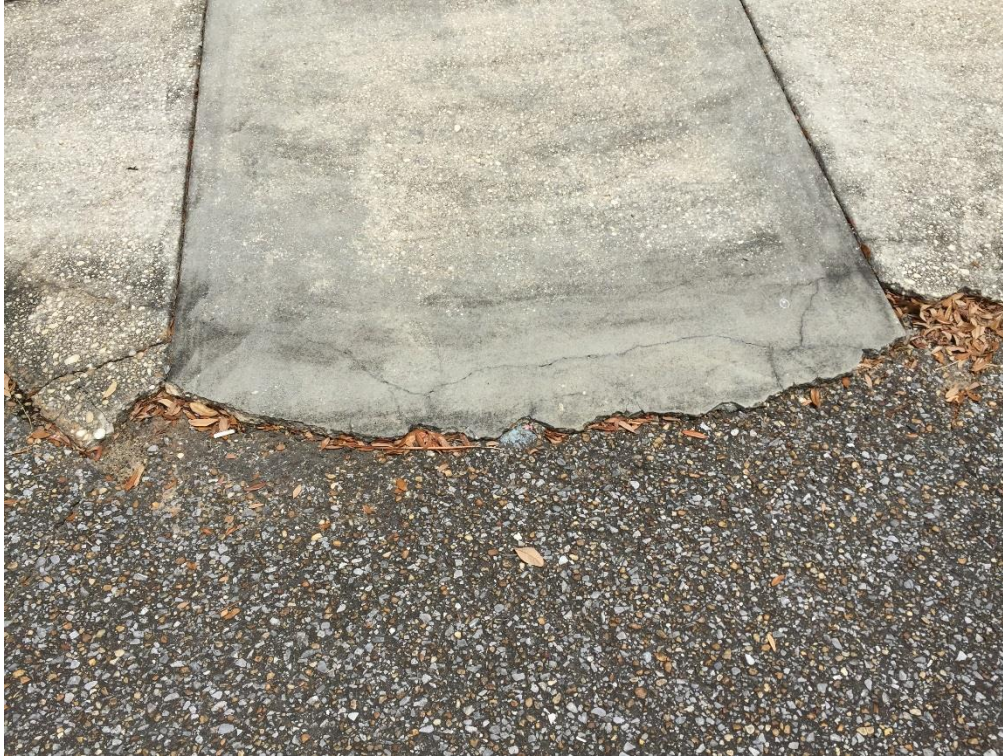
FIG PNS.54 – Second deteriorated access ramp from ADA space to sidewalk immediately in front of station
