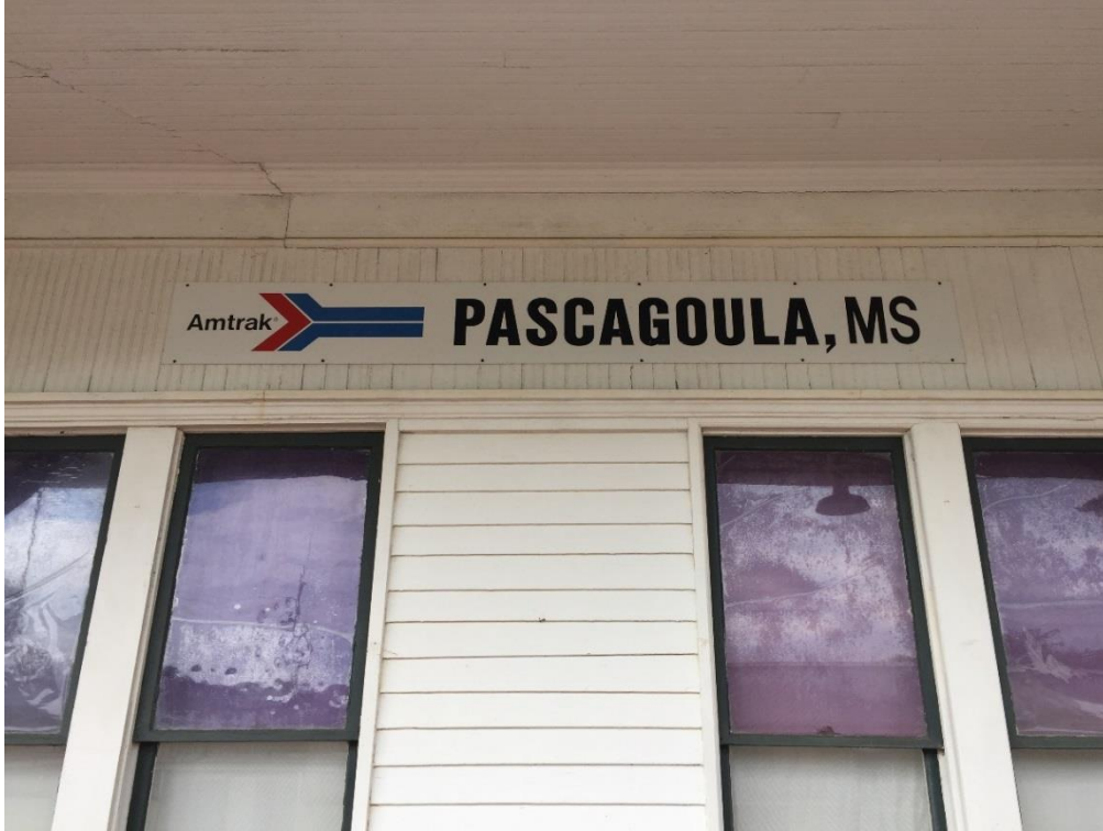
FIG PAG.07 – Outdated signage on station exterior
