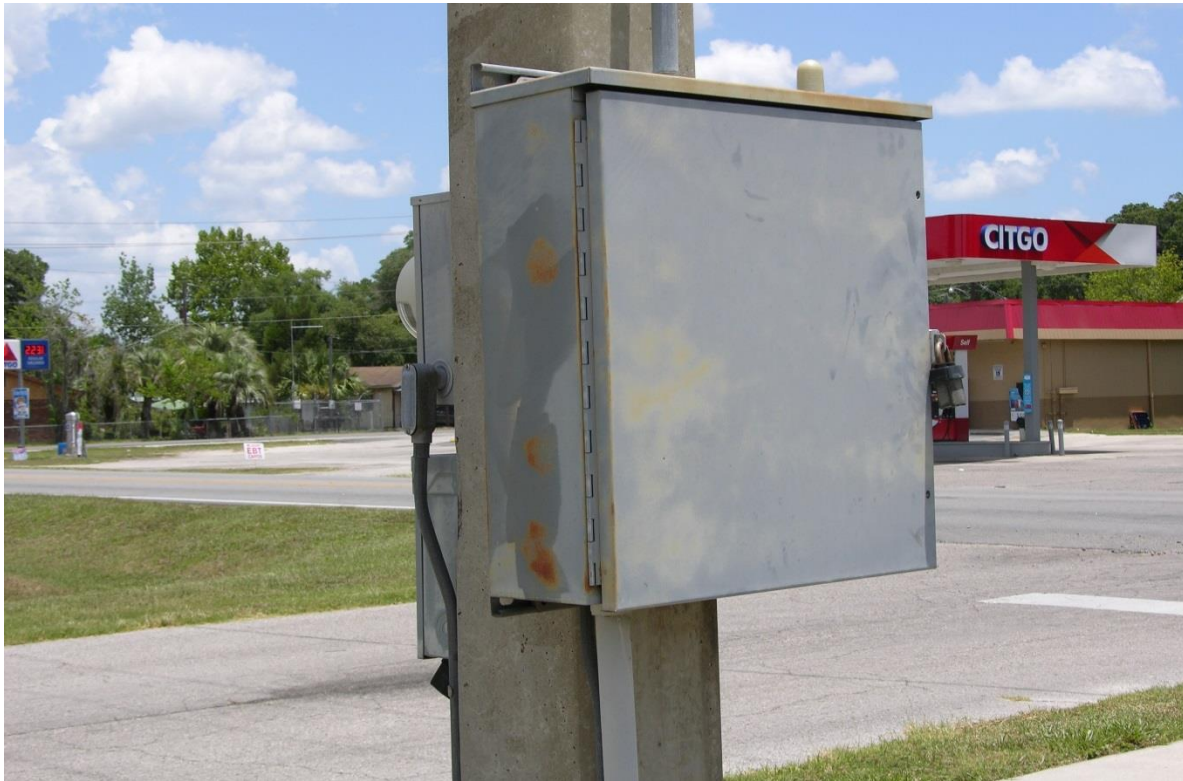
FIG LAC.16 – Distribution panel at Lake City FL station
