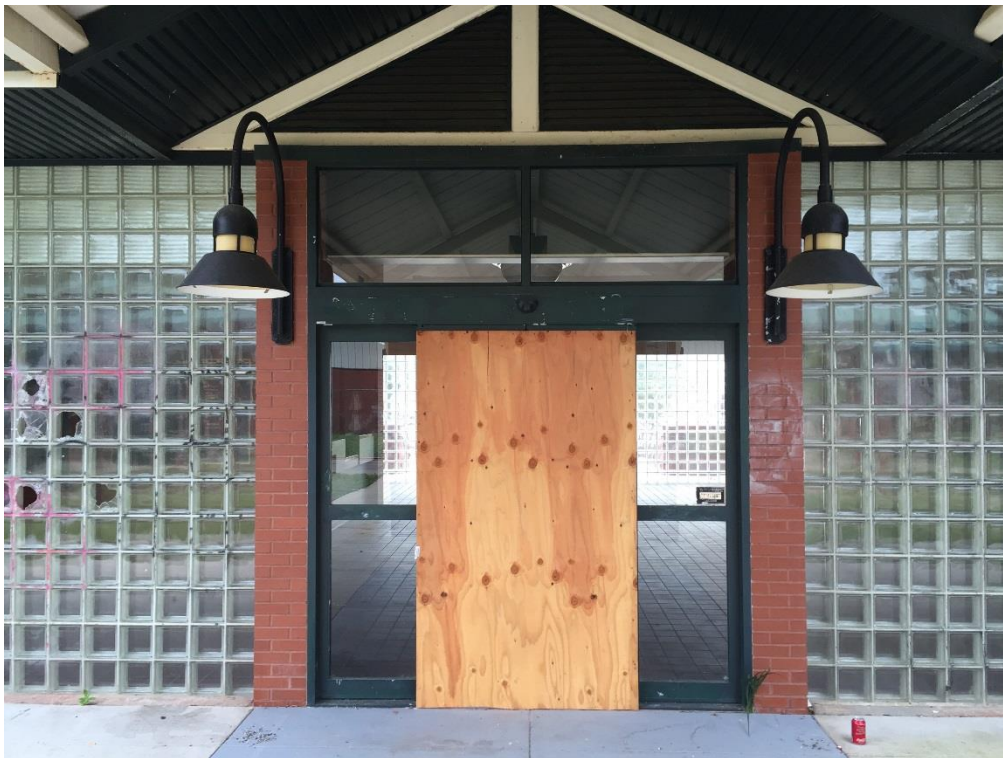
FIG PNS.38 – Boarded up sliding door at rear of station building; the bottom glass panes were broken by vandals
