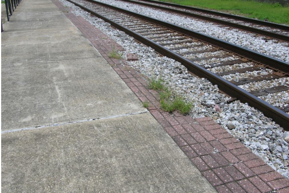
FIG MOE.13 – Further tactile strip deterioration
