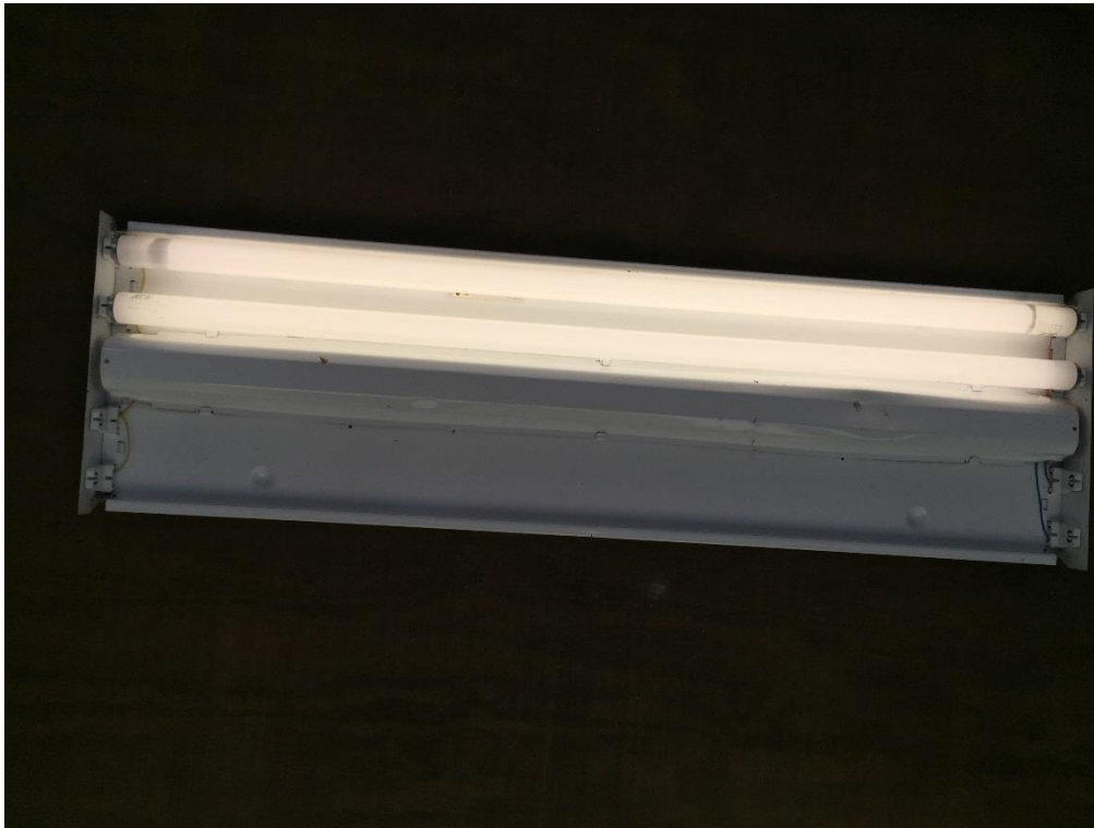
FIG CSV.18 – Fluorescent lighting on interior of station building
