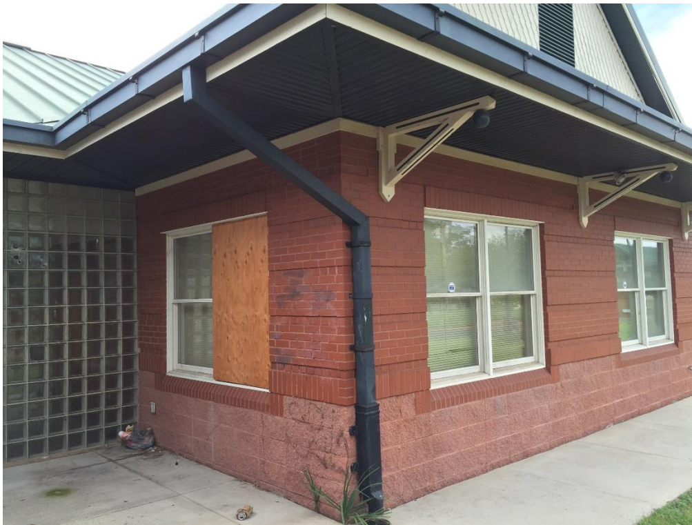
FIG PNS.42 – Boarded up office window on west side of building
