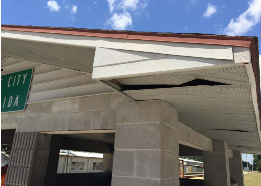
FIG LAC.12 – The shelter roof structure below the eaves require repairs for Lake City FL station
