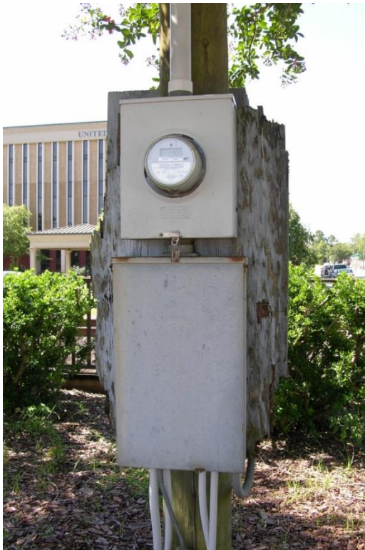
FIG ATR.16 – Electrical Service and Panel
