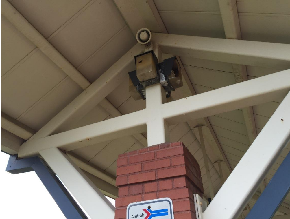
FIG PNS.52 – Canopy column wall pack
