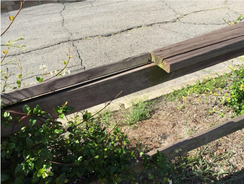
FIG GUF.12 – Section of broken platform railing
