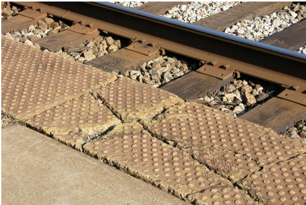
FIG GUF.10 – Tactile Surface experiencing significant cracking
