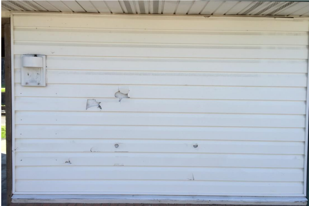
FIG CSV.11 – Exterior siding and non-functioning wall pack (roadside)
