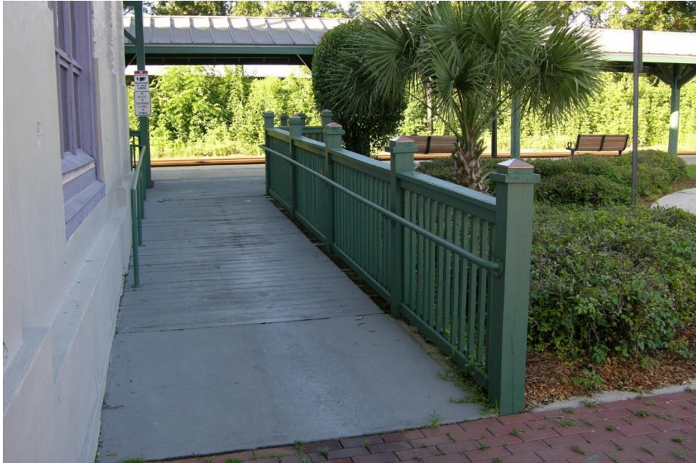
FIG TLH.23 – Walkway to station building/platform needs paint
