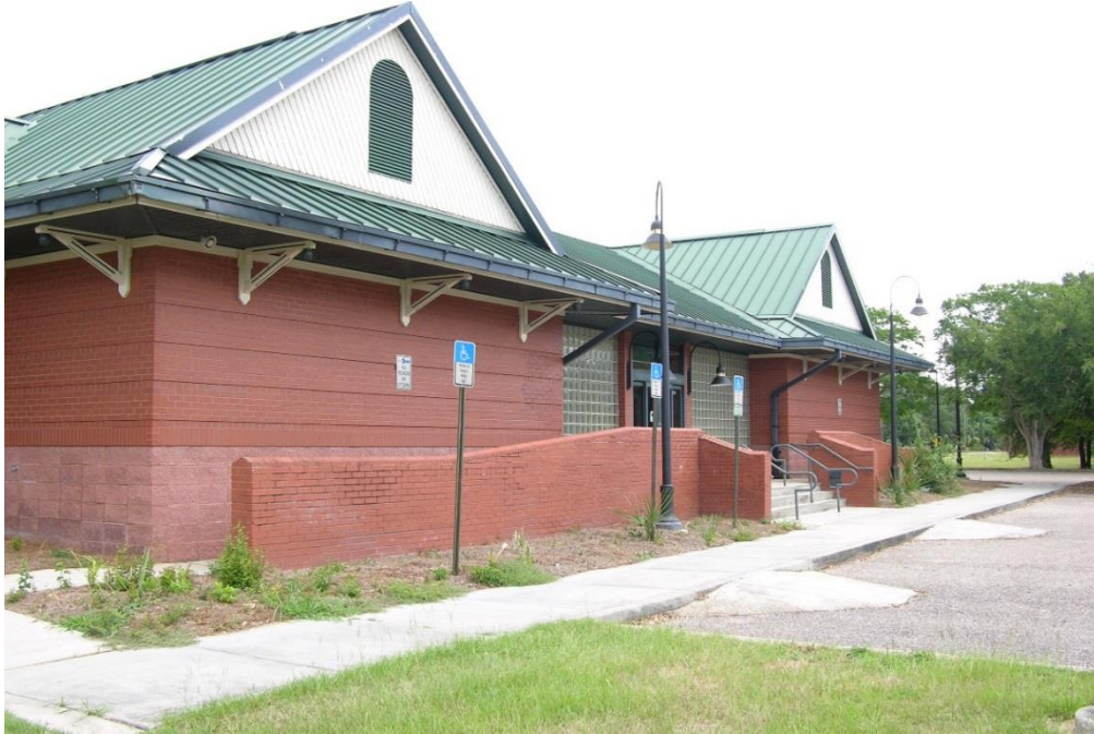
FIG PNS.45 – Rainwater conductor west side front corner damage
