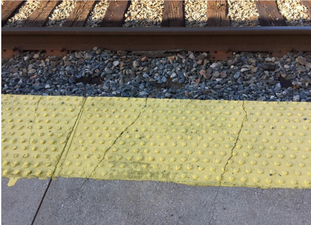
FIG TLH.61 – Worn and crack tactile at the edge of the platform
