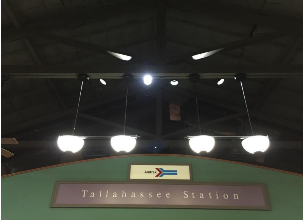
FIG TLH.37 – Lighting fixtures in station waiting room
