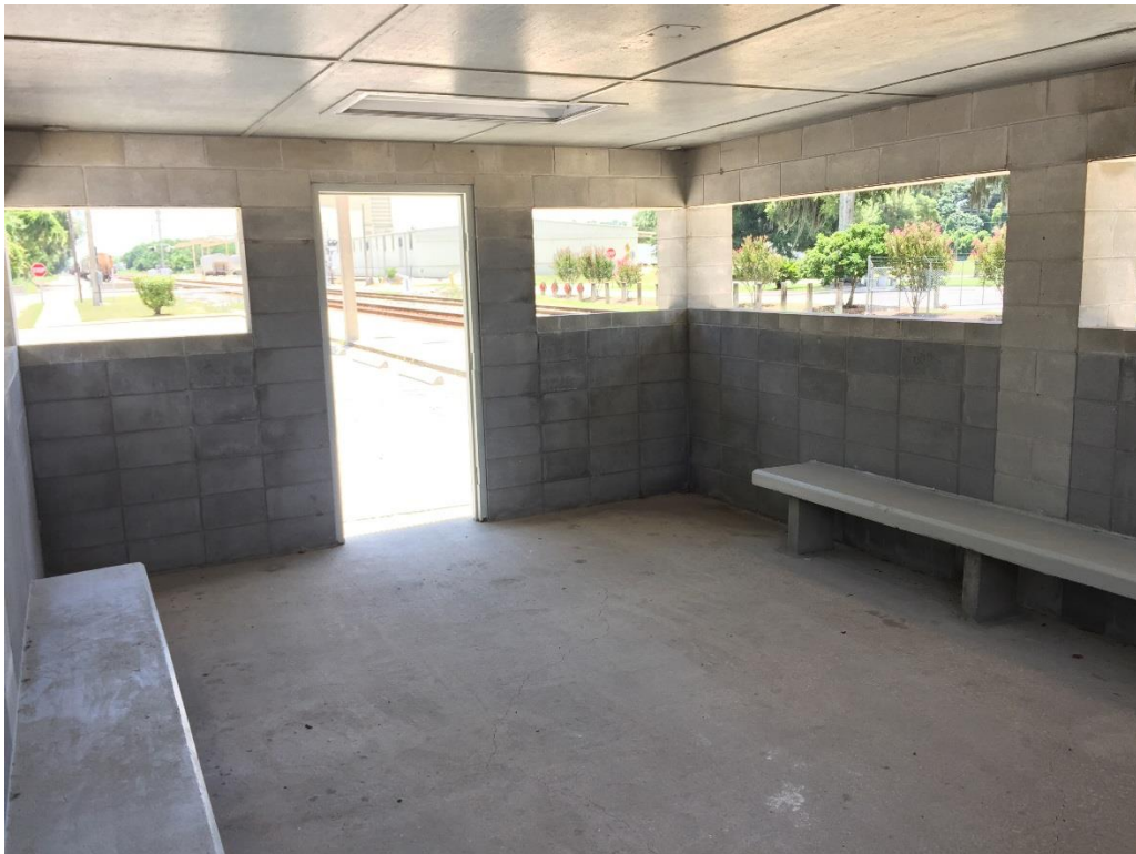
FIG LAC.20 – Shelter station interior (minor cracking visible on floor)
