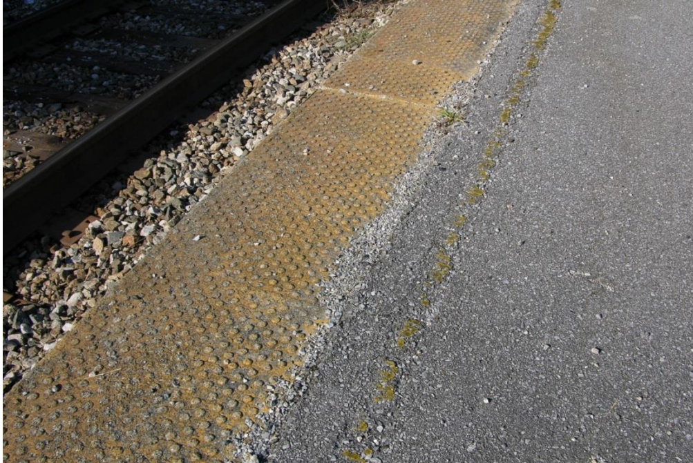
FIG CSV.13 – Condition of tactile surface at platform
