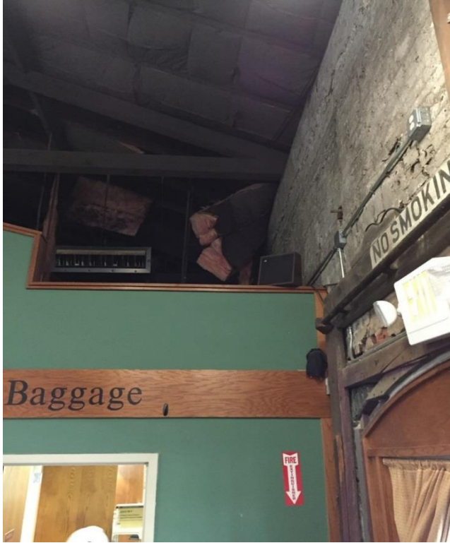
FIG TLG.35 – Insulation that has come free from rafters
