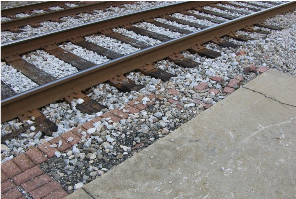
FIG MOE.12 – Tactile strip deterioration at southern end of platform
