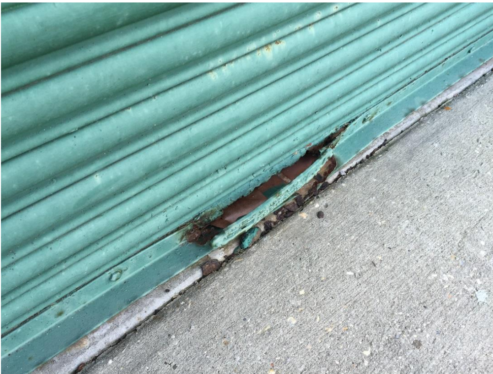
FIG BAS.12 – Deteriorated handle of roll up door located on east side of historic station building
