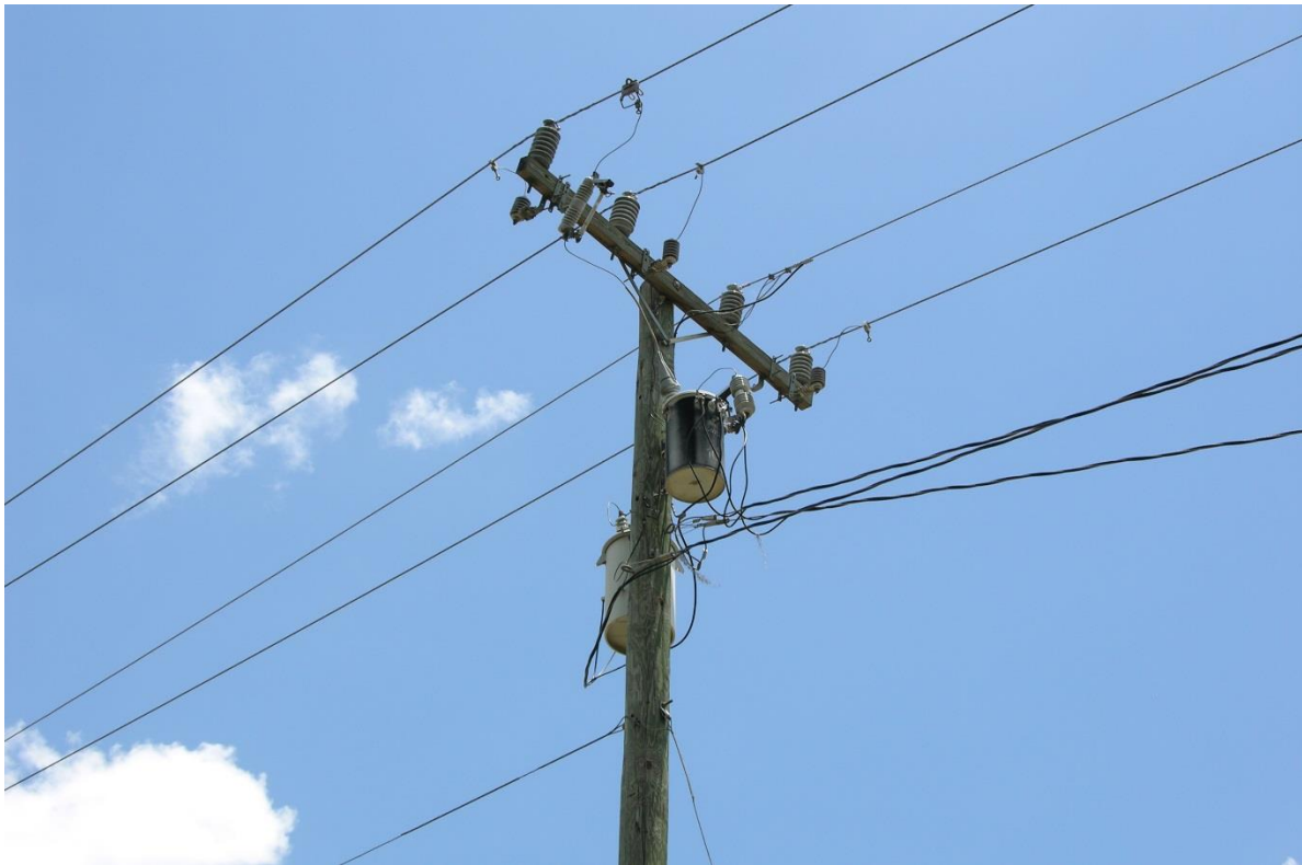
FIG LAC.14 – The service entrance and transformers for Lake City FL station
