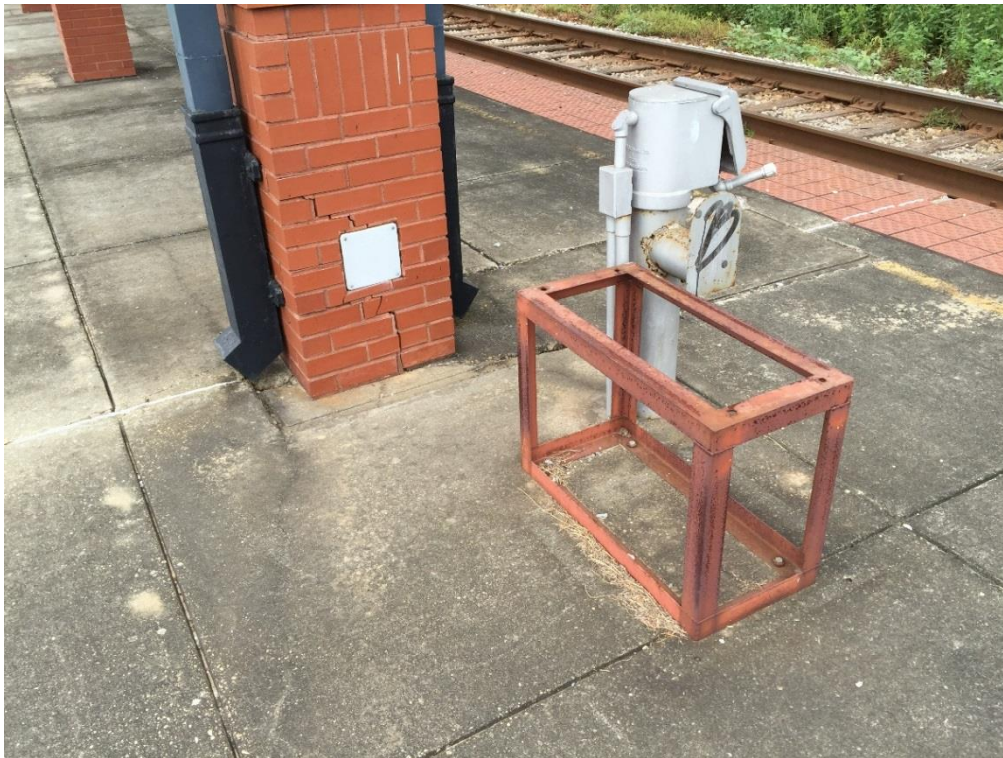
FIG PNS.16 – Cracks in canopy structural-support column
