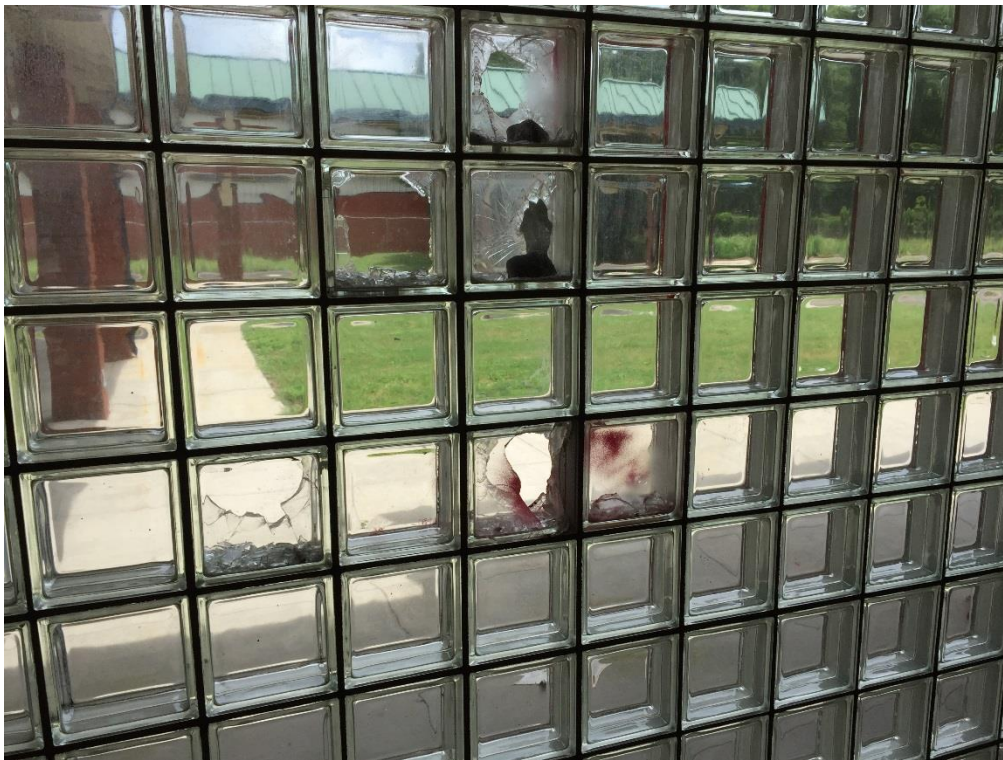
FIG PNS.24 – Eastern glass block infill window in waiting room looking out towards platform—a few of the blocks have been broken by vandals
