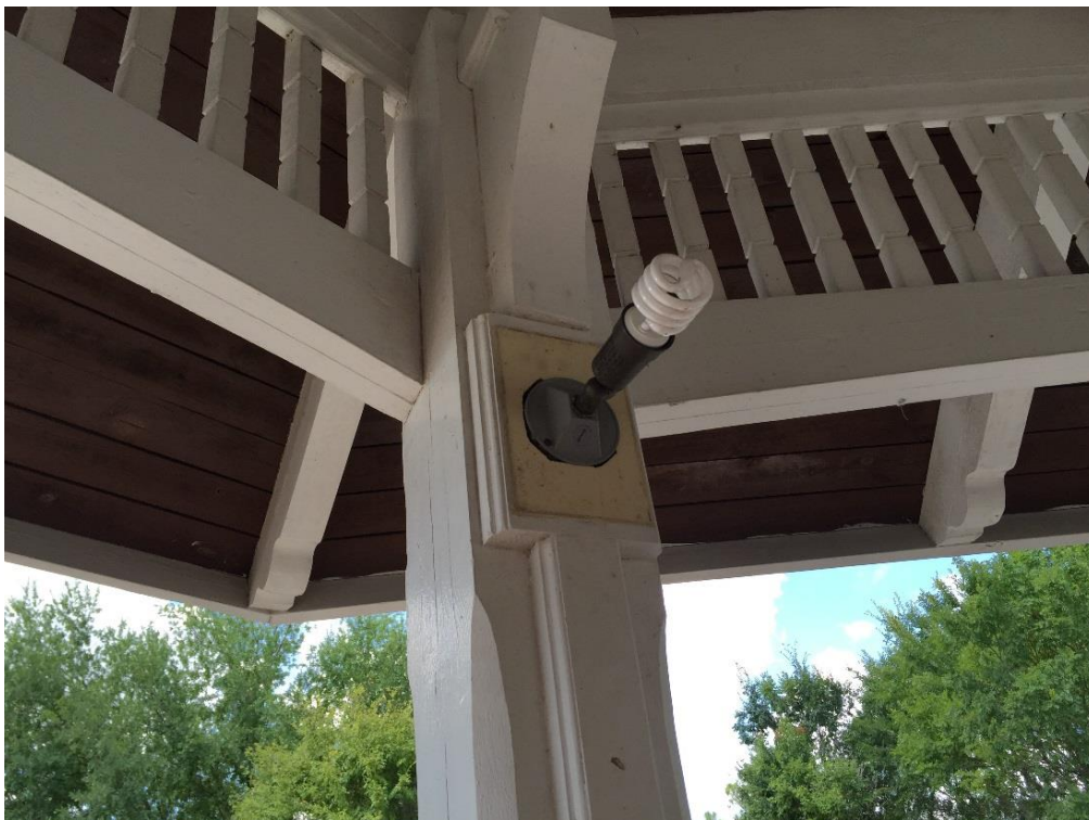
FIG MDO.23 – “In-tact” lighting fixture that appears to have been retrofitted with different fixture
