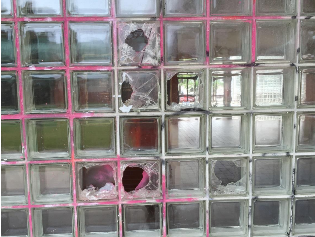
FIG PNS.41 – Exterior view of broken glass blocks and graffiti
