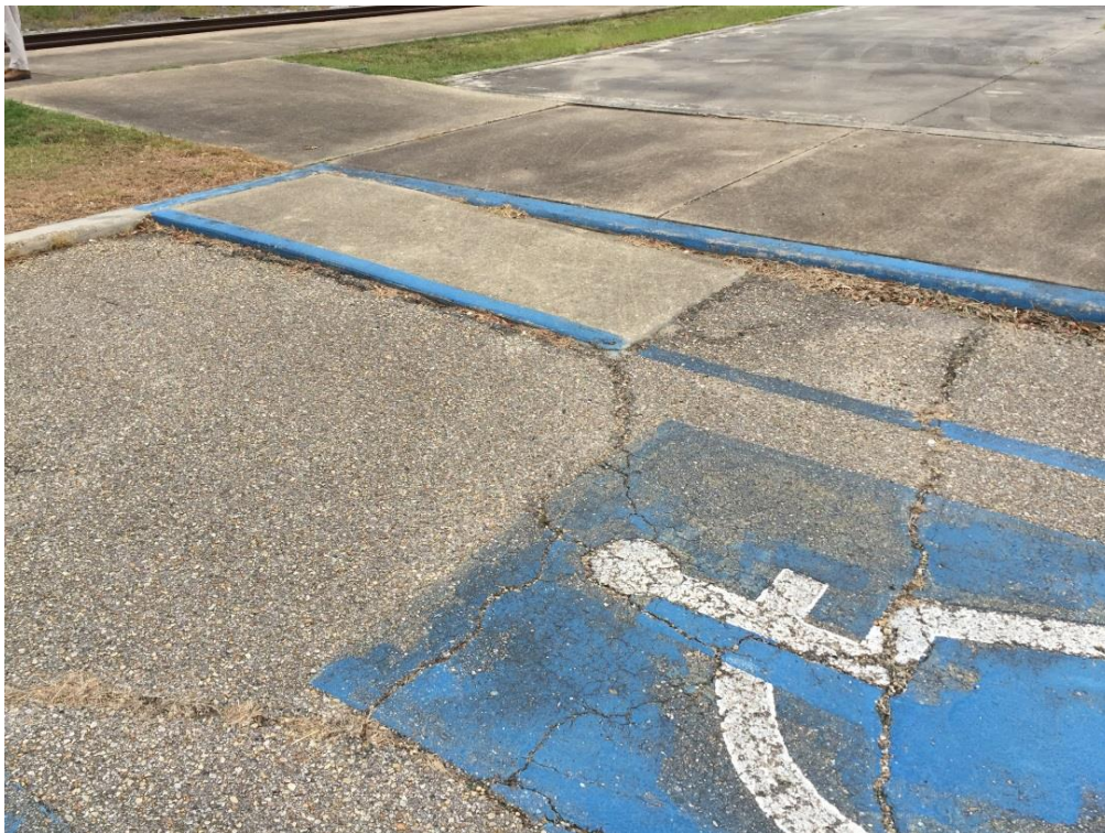
FIG BIX.10 – Intended accessible path from ADA parking requiring remediation
