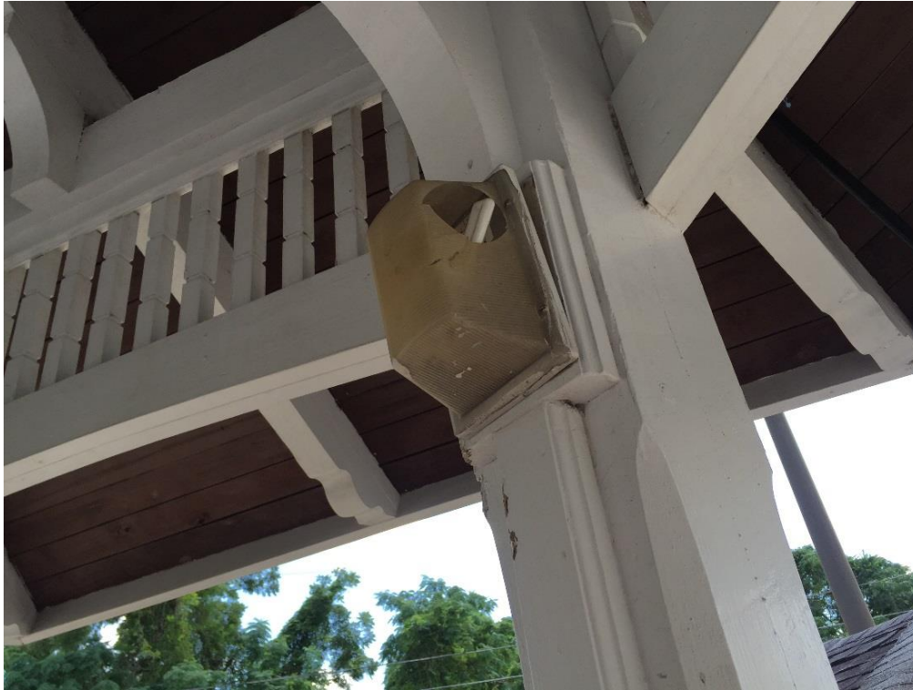
FIG MDO.22 – Typical wall-pack lighting fixture in poor condition
