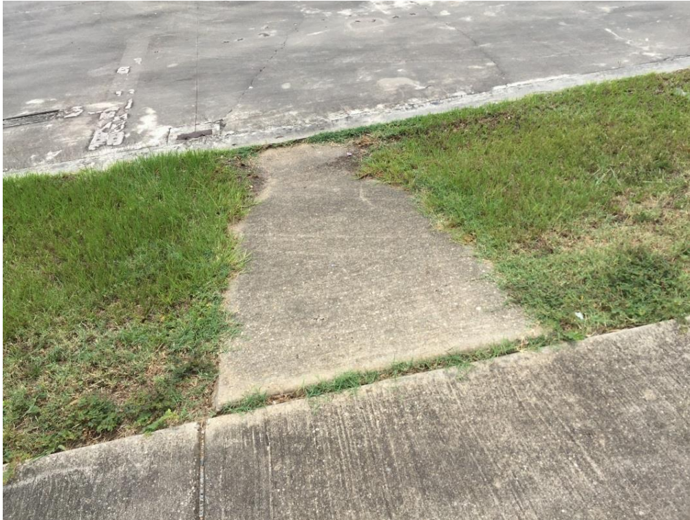
FIG BIX.09 – Access from concrete slab from demolished station building to platform with vegetation in cracks
