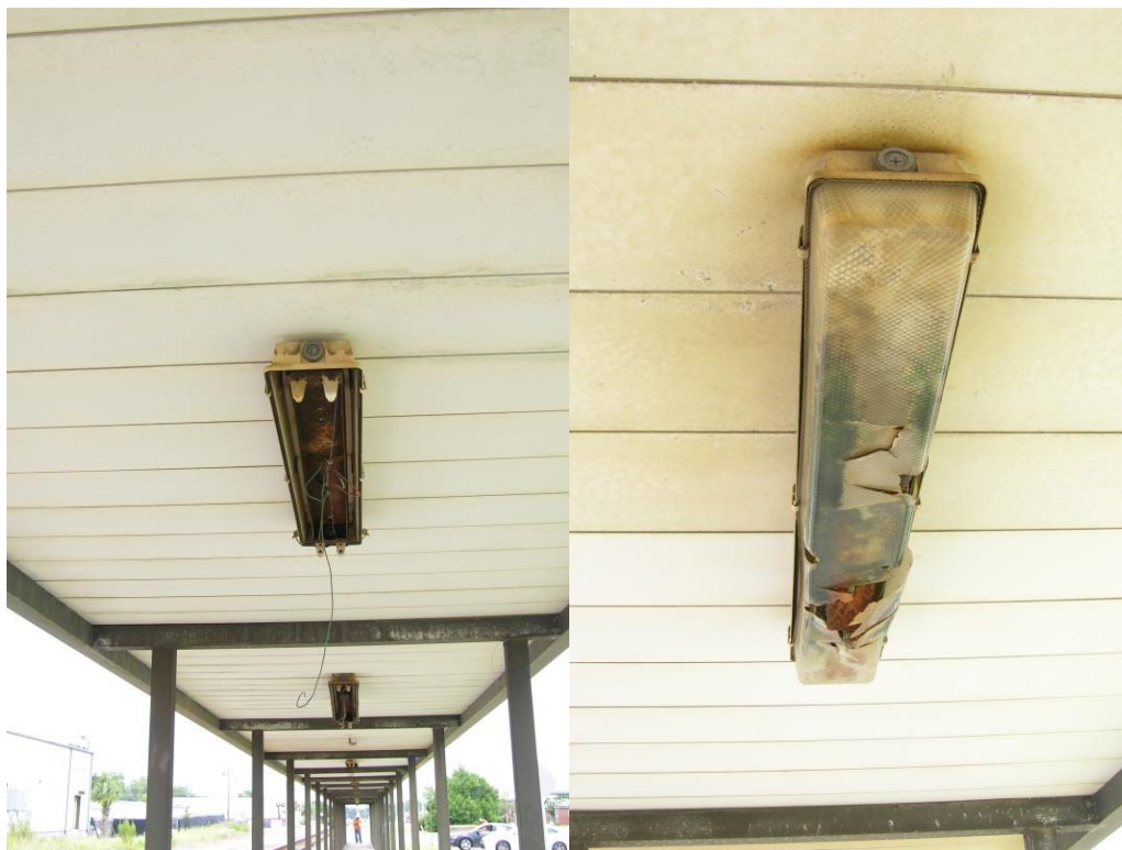
FIG BIX.08 – Platform Lighting Fixtures
