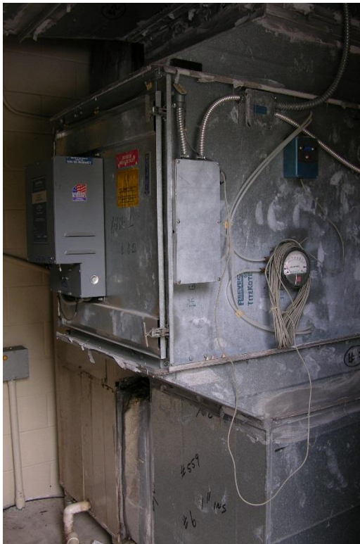
FIG PNS.46 – Air handler
