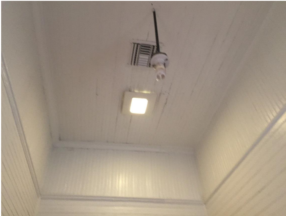
FIG PAG.22 – Lighting in Women's restroom requiring replacement
