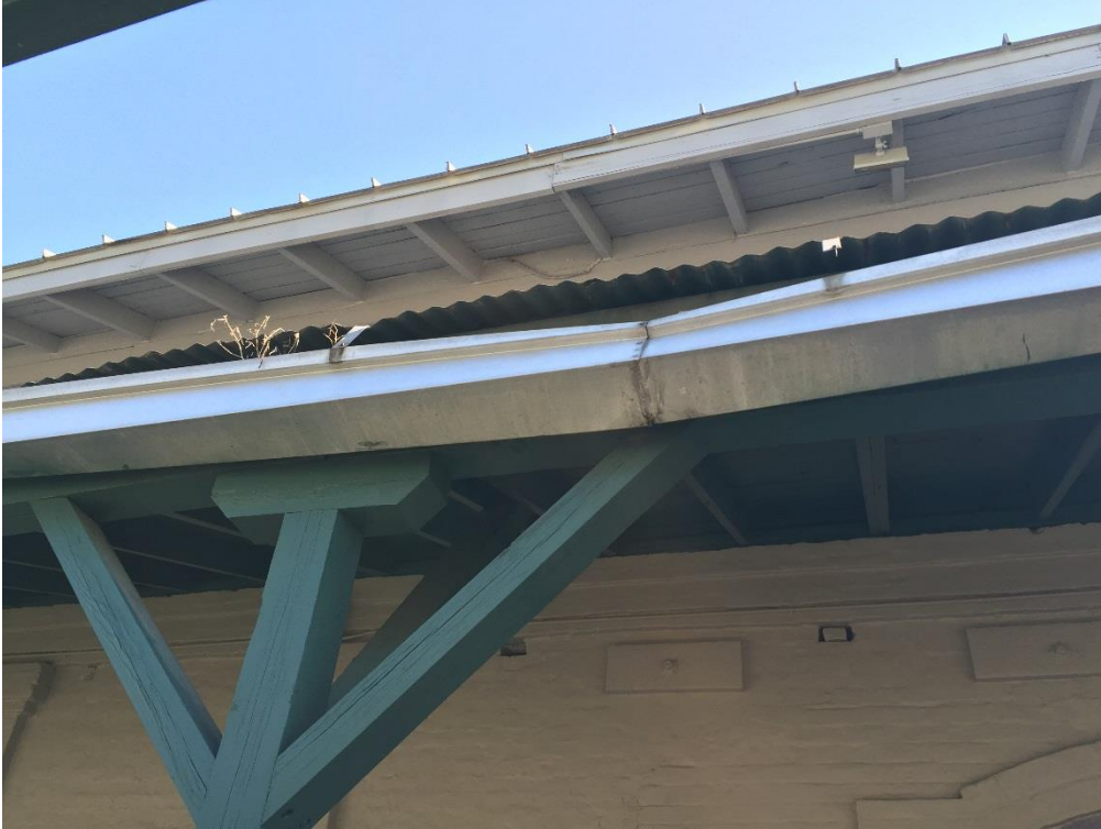
FIG TLH.63 – Dented gutter located on back of station
