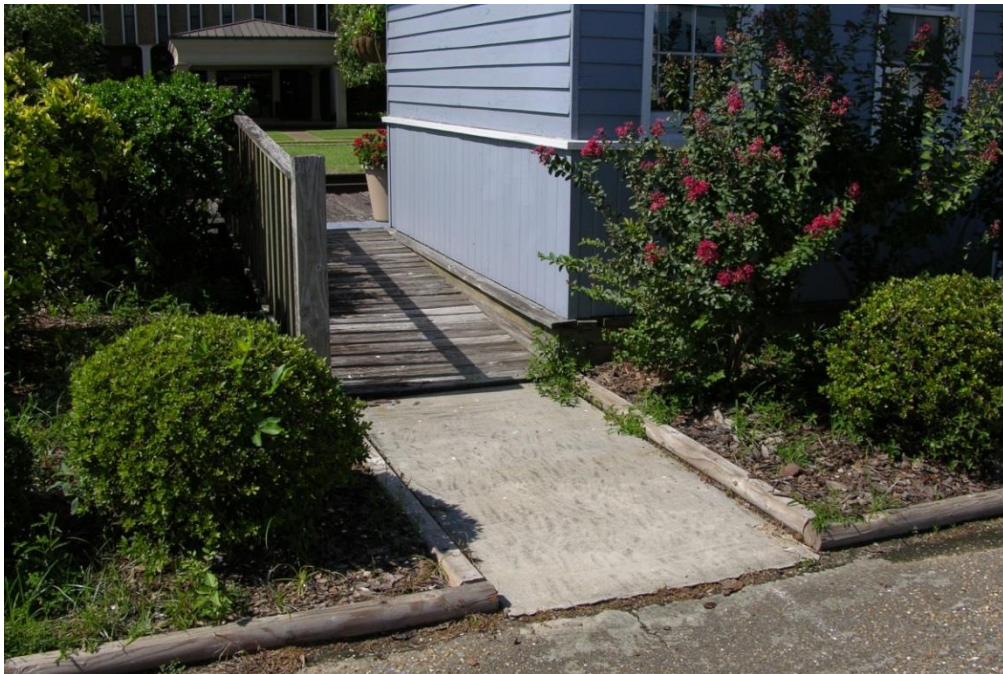
FIG ATR.18 – Non ADA compliant access (immediately adjacent to station structure) to deteriorated platform
