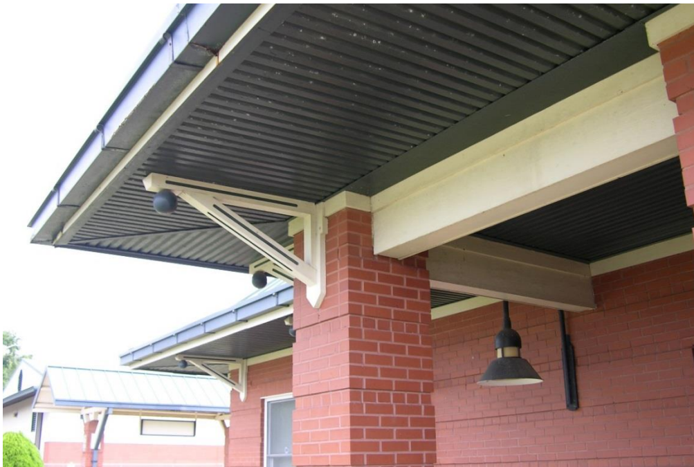
FIG PNS.44 – Minor rust on rainwater conductor on west side of building
