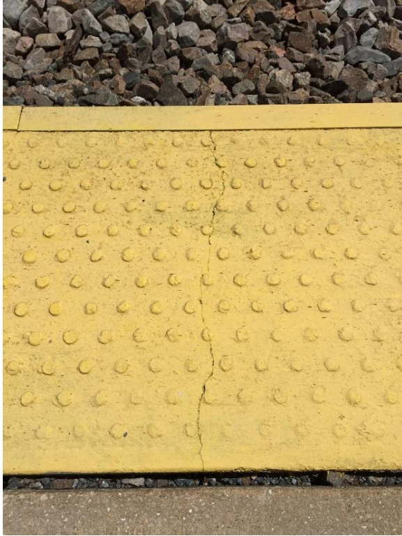
FIG MDO.15 – Small crack that has propagated across tactile strip.
