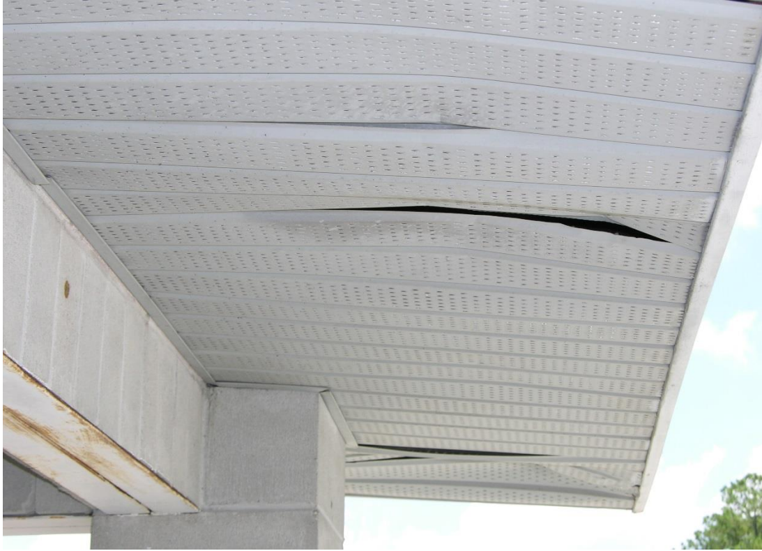
FIG LAC.13 – The shelter roof structure below the eaves require repairs for Lake City FL station
