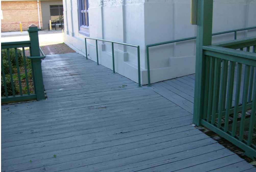
FIG TLH.25 – Walkway to station building/platform needs paint
