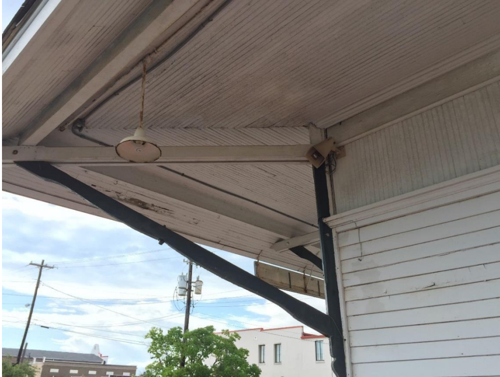
FIG PAG.09 – Building awning / canopy in need of paint
