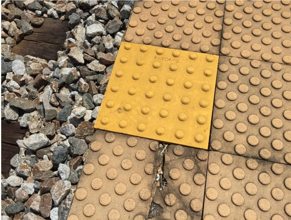
FIG BAS.09 – Tactile surface failure
