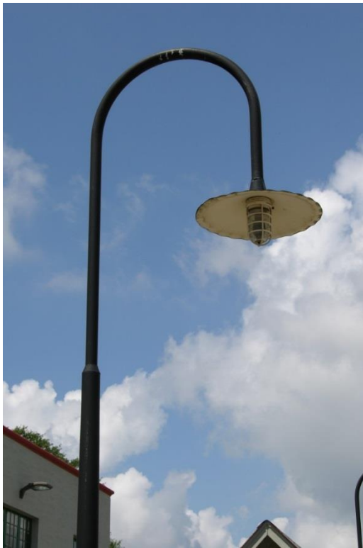
FIG BAS.08 – Platform mounted lighting fixture example
