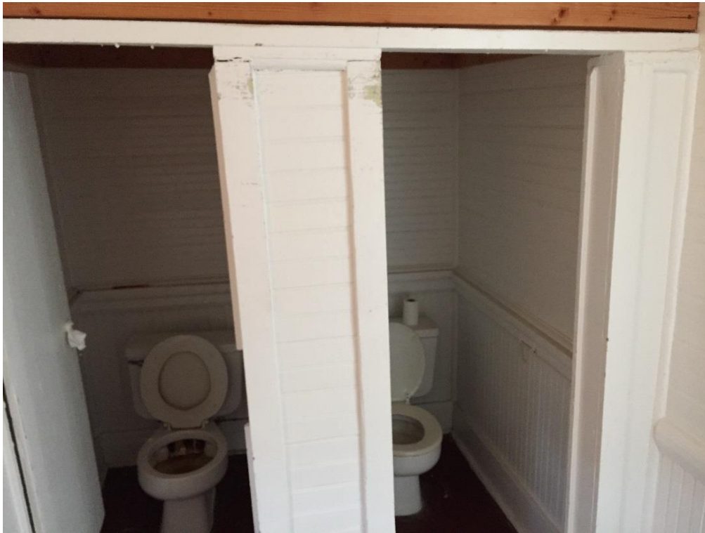
FIG PAG.16 – Toilets in Women’s restroom
