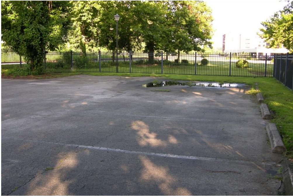
FIG TLH.07 – Potholes and standing water evidence in Parking Lot for Tallahassee FL station
