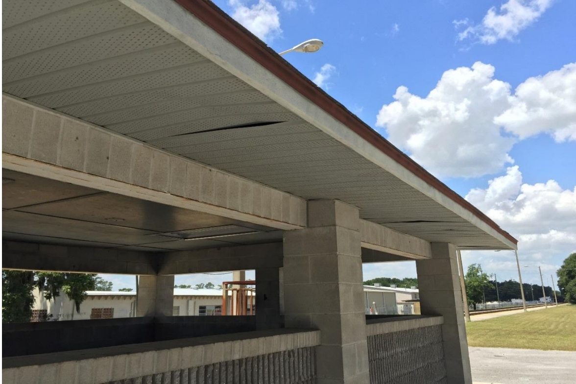
FIG LAC.11 – The shelter roof structure below the eaves require repairs for Lake City FL station
