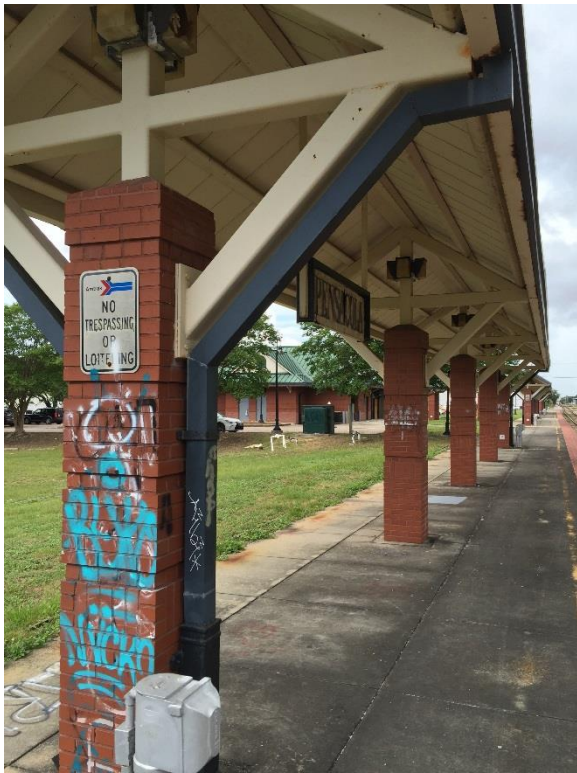
FIG PNS.18 – Close up view of gutters / graffiti seen in FIG PNS.17; rust can be seen on the gutter at ninety degree angle joint, and along the canopy edge
