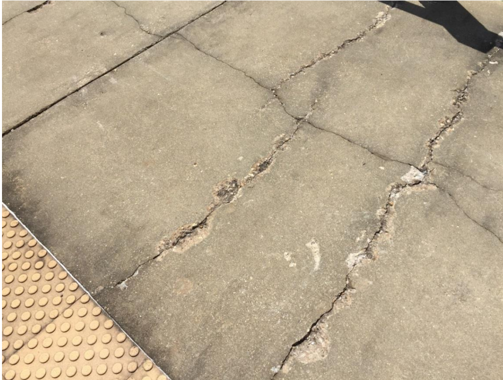
FIG BAS.03 – Concrete platform surface is spalled and cracked and requires replacement
