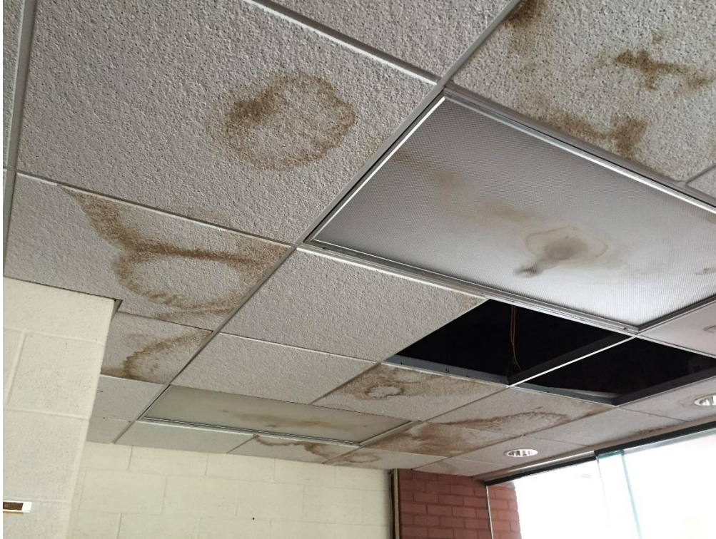
FIG PNS.29 – Ticket office acoustical tile ceiling in need of replacement
