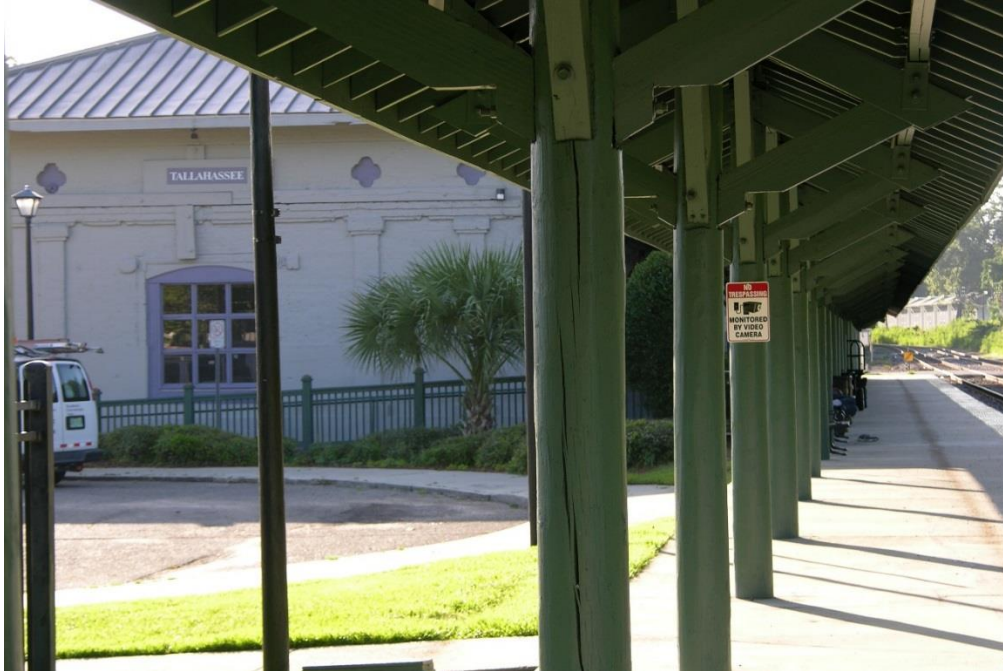
FIG TLH.27 – Minor cracking of canopy’s wooden support columns
