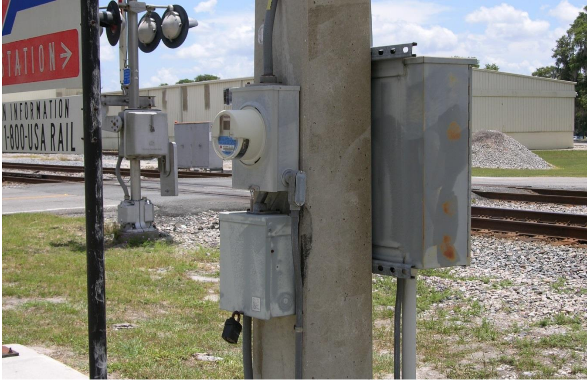
FIG LAC.15 – The service entrance and transformers for Lake City FL station
