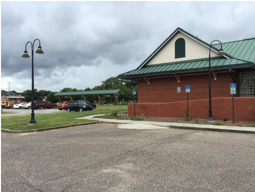
FIG PNS.04 – ADA spaces in front of station with missing striping
