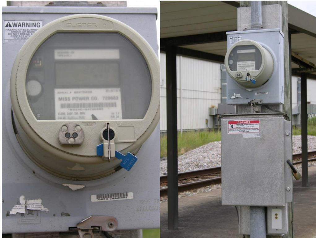
FIG BIX.07 – Electric Service Entrance / Panel
