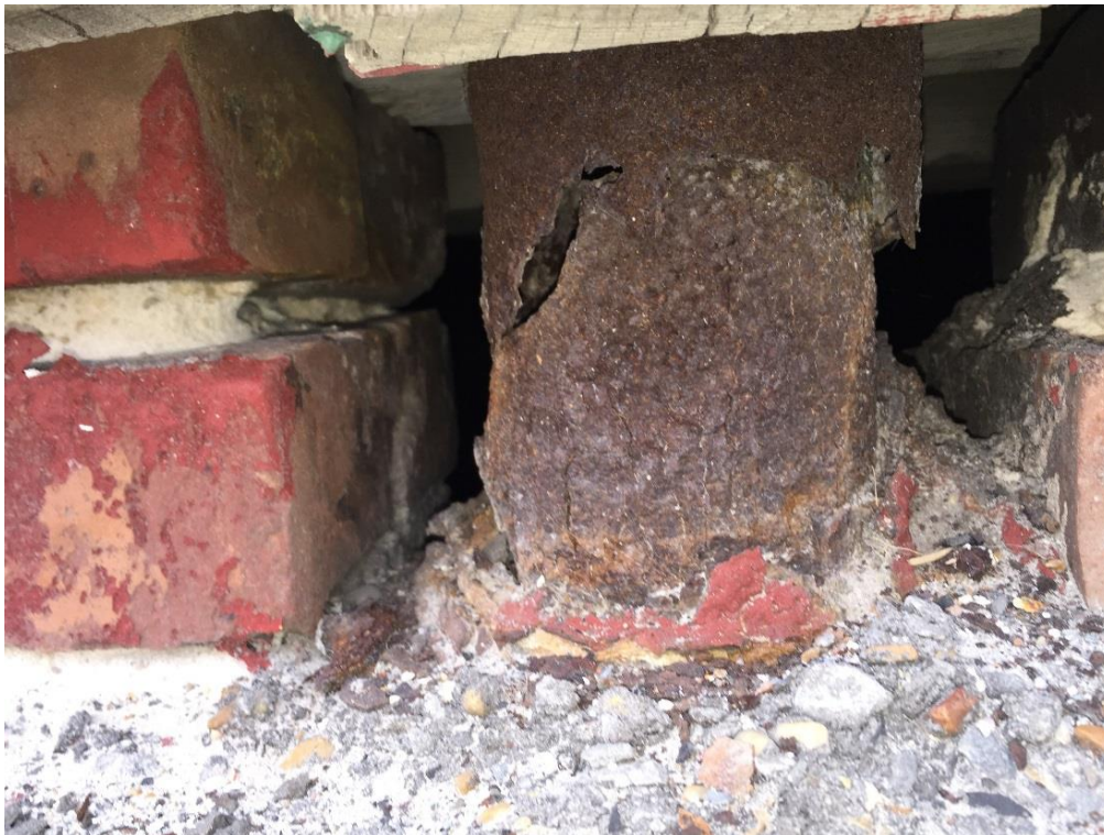
FIG PAG.24 – Deteriorated pipe located in brick foundation immediately adjacent to Railroad Avenue.
