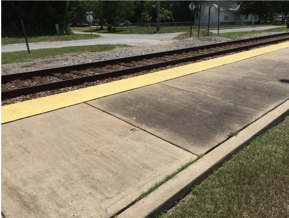
FIG MDO.13 – Section of platform northwest of the station, near the edge of the parking lot. The side closest to the station seems to have been power washed.
