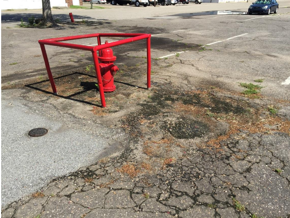
FIG ATR.15 – Fire hydrant in parking lot area
