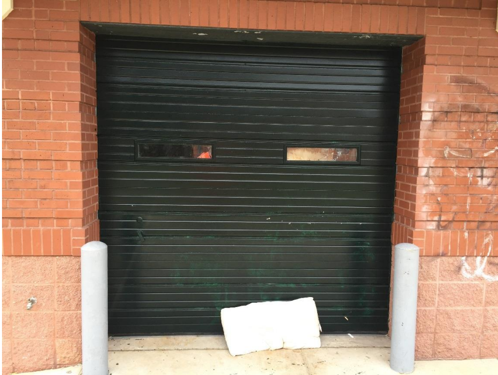
FIG PNS.37 – Automatic roll-up door on back of station building
