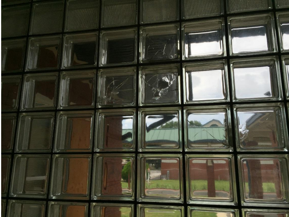
FIG PNS.25 – Western glass black infill window in waiting room looking out towards platform—a few of the blocks have been broken by vandals
