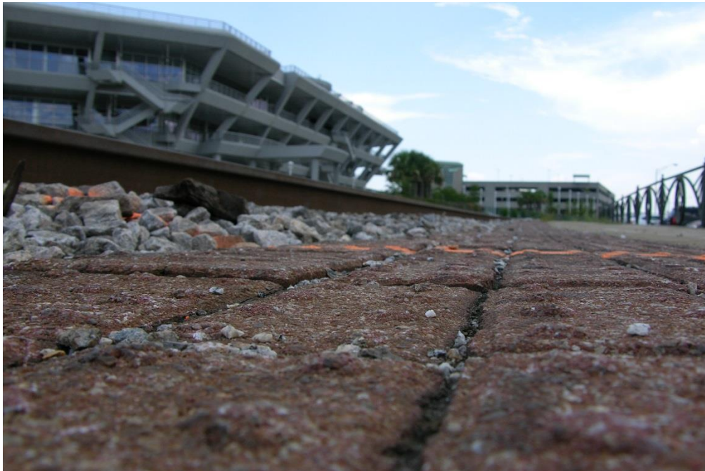
FIG MOE.10 – Platform level view at section experiencing excessive cracking
