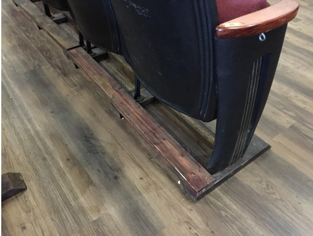
FIG TLH.29 – Base of theater seats – not fixed to wood floor
