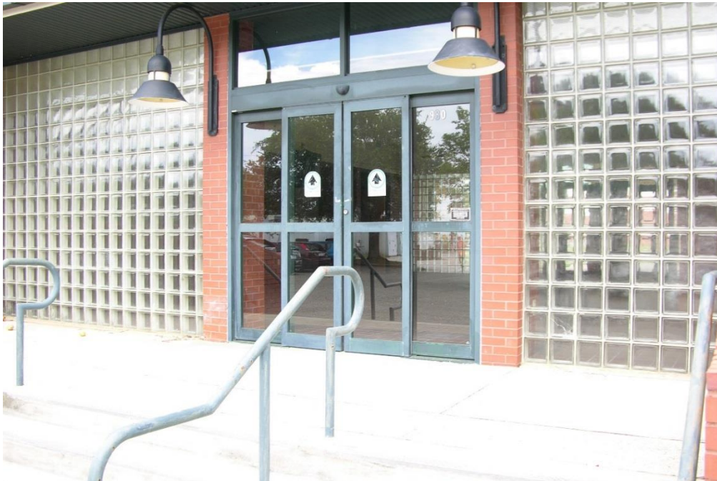
FIG PNS.08 – Entrance-way handrails with rust / chipped paint
