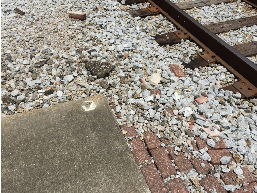
FIG MOE.15 – Deteriorating tactile at northern end of the platform
