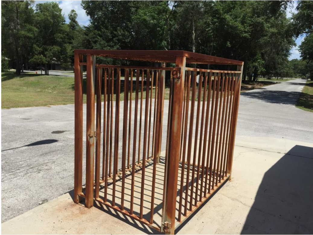
FIG LAC.17 – Wheelchair Lift enclosure
