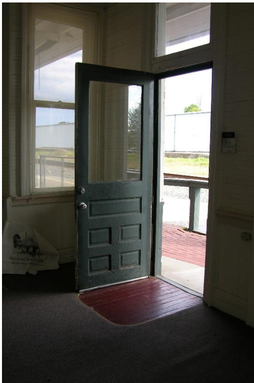
FIG PAG.20 – Exterior door in need of scraping & paint
