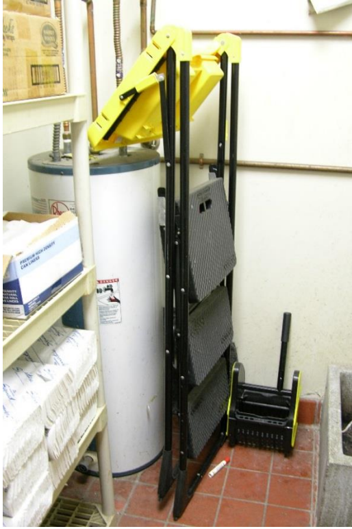
FIG TLH.55 – Water heater in utility closet
