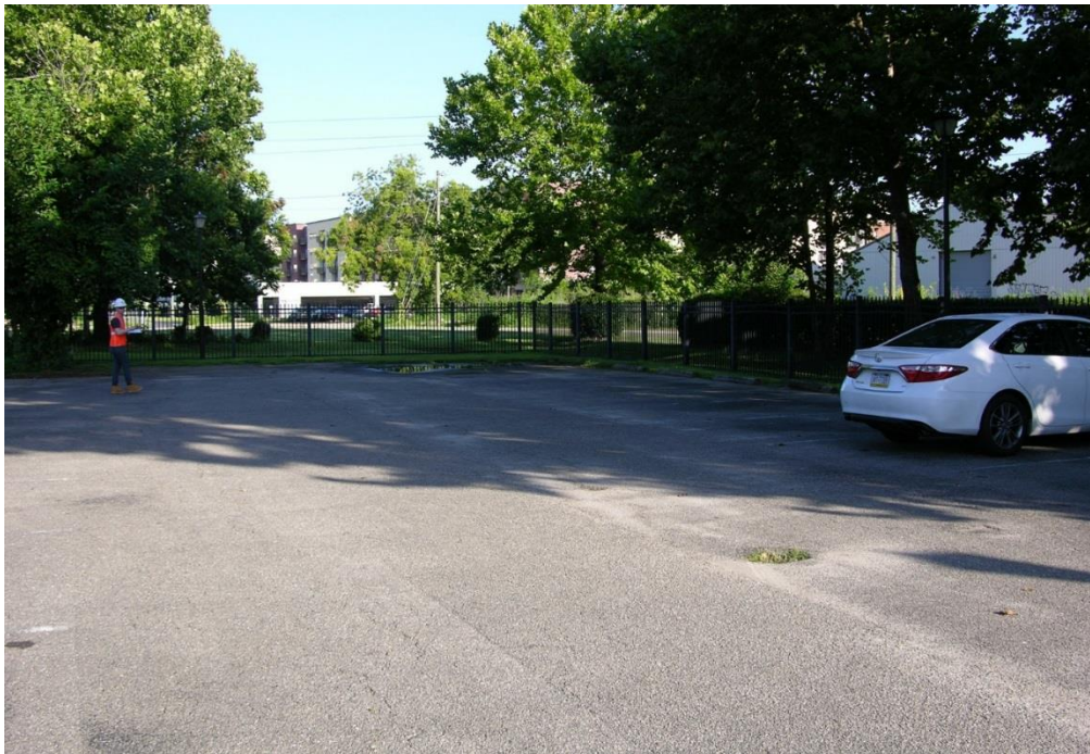
FIG TLH.06 – Potholes and standing water evidence in Parking Lot for Tallahassee FL station
