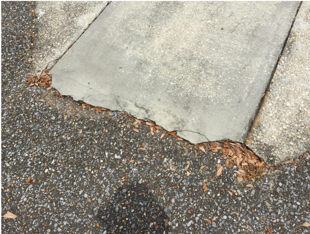
FIG PNS.53 – First deteriorated access ramp from ADA space to sidewalk immediately in front of station
