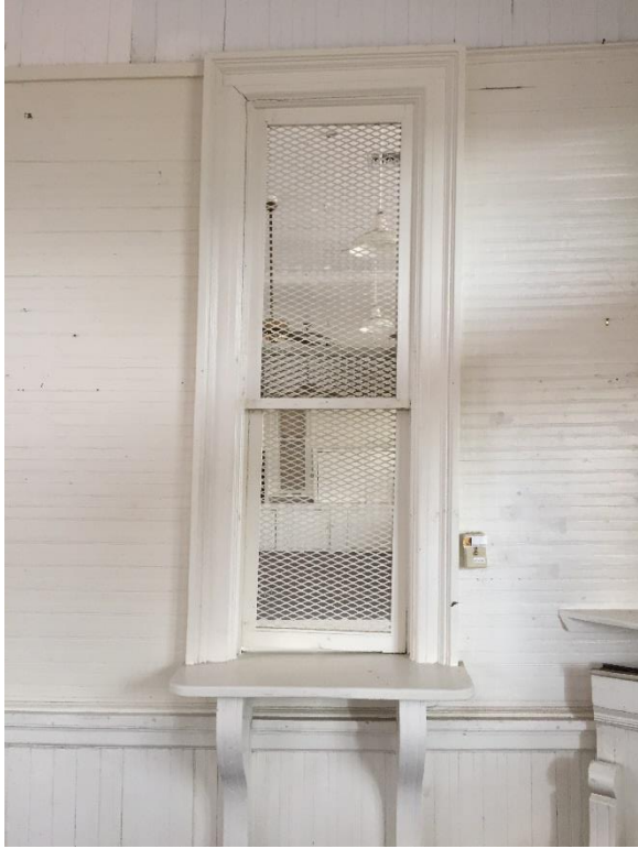
FIG PAG.13 – Close-up view of ticket window (the settling of the building’s foundation is evidenced by the fact that the window does not sit flush with the counter)
