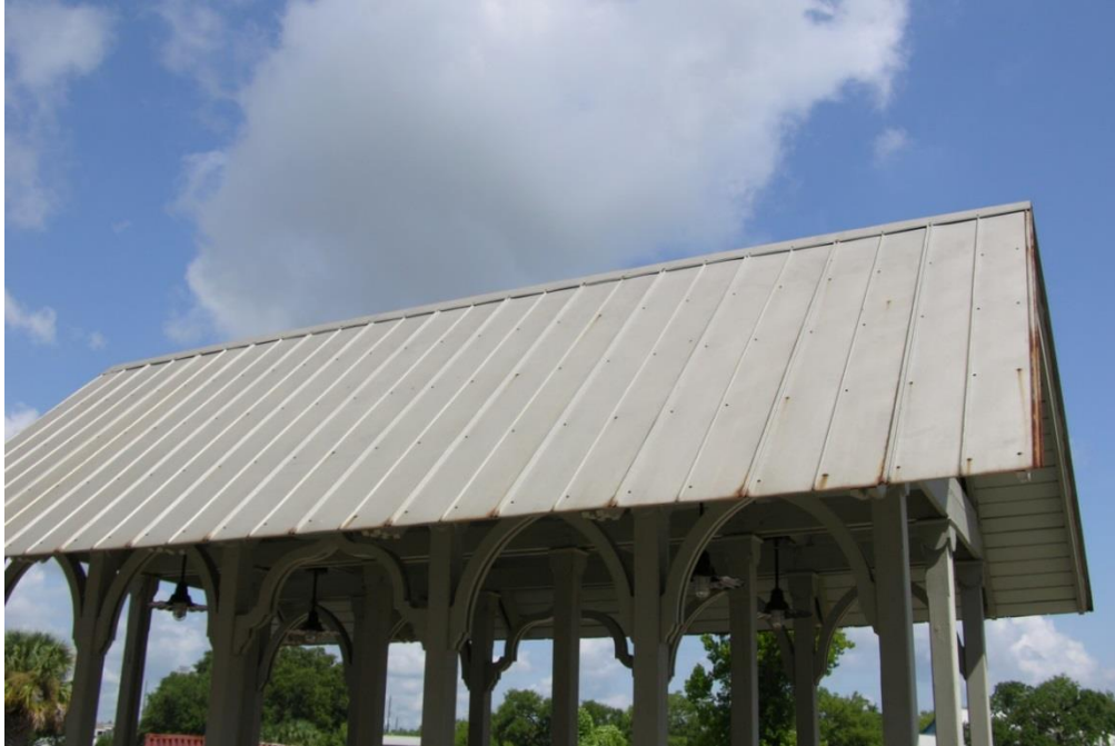
FIG BAS.05 – Platform Canopy structure roof rust
