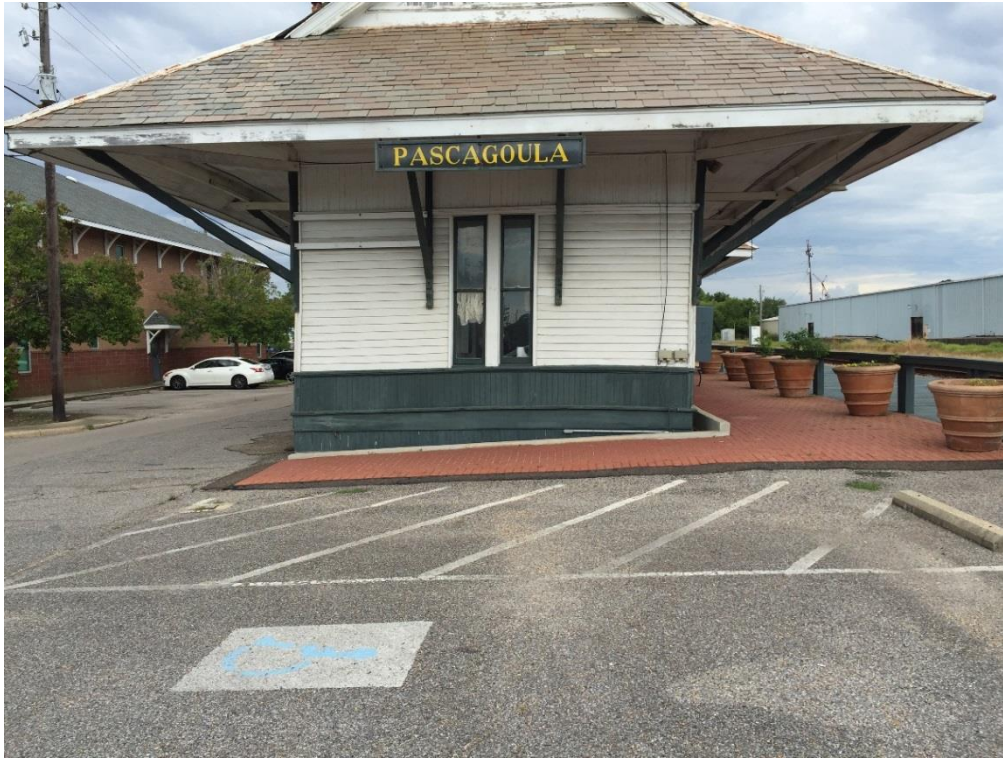
FIG PAG.19 – Evidence of settling
