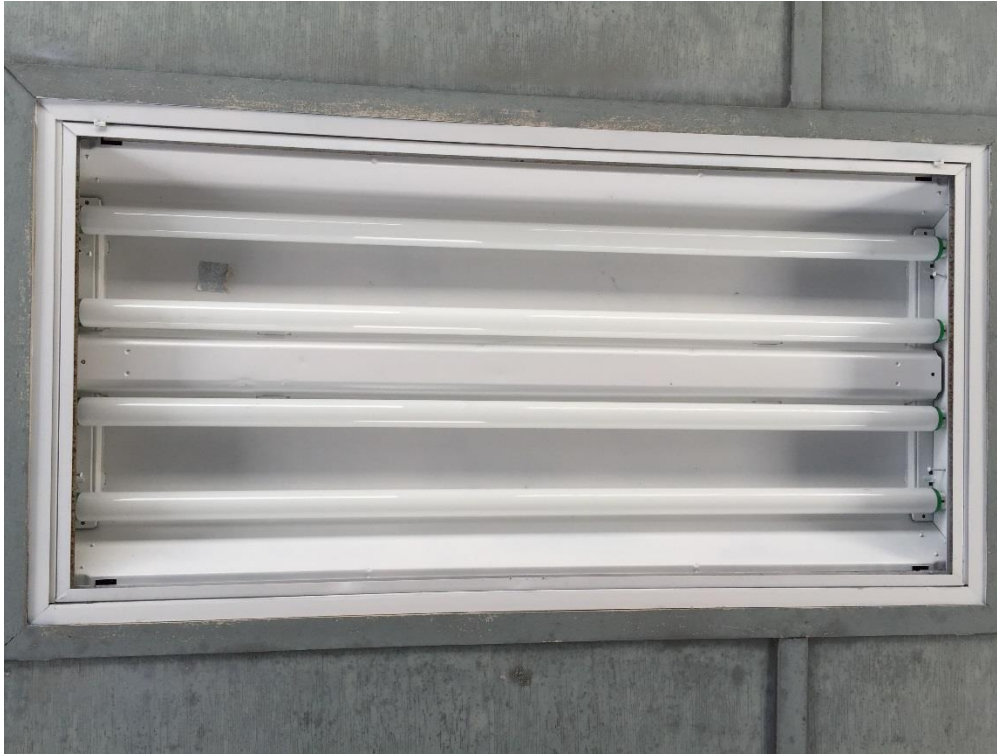
FIG LAC 23 – One (1) of two (2) fluorescent lights located inside the shelter
