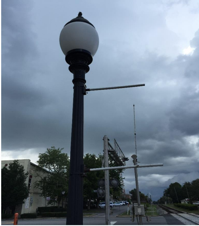
FIG CIP.17 – Black platform-mounted lighting fixtures for the Chipley FL station
