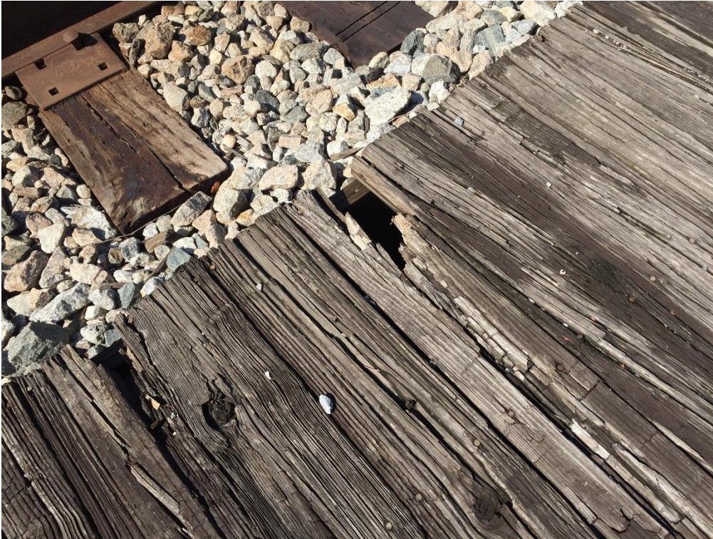
FIG ATR.10 – Example of platform deterioration
