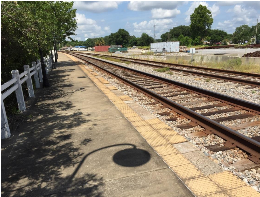
FIG BAS.10 – Tactile surface failure
