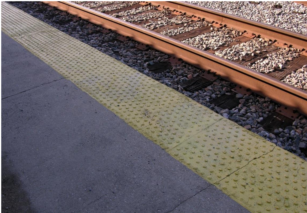
FIG TLH.60 – Worn-down tactile nubs & cracking
