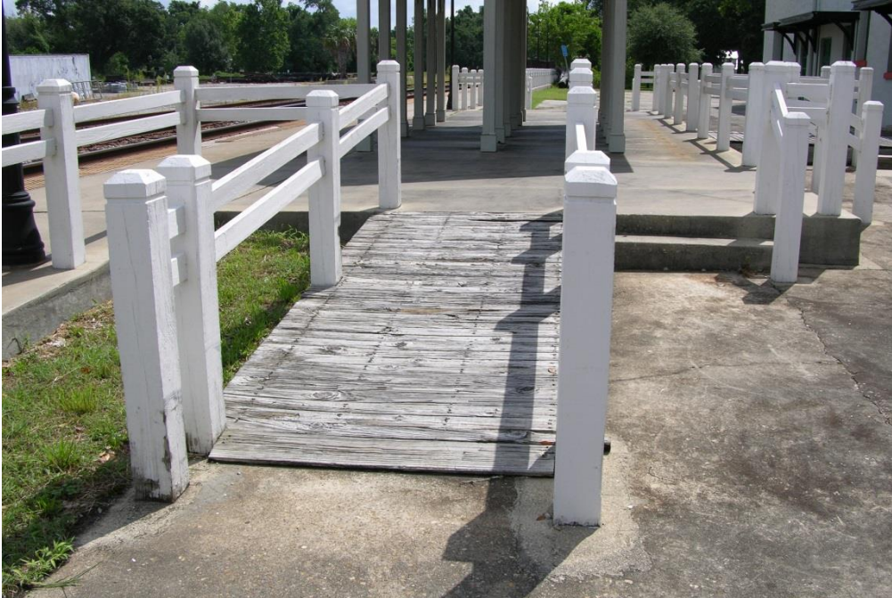
FIG BAS.11 – Non compliant and deteriorating ramps
