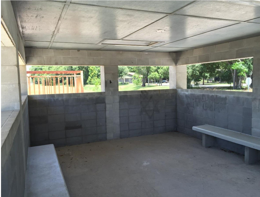
FIG LAC.21 – Graffiti on station interior walls
