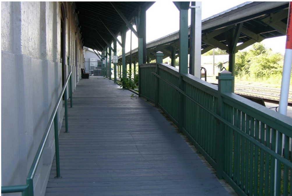
FIG TLH.24 – Walkway to station building/platform needs paint
