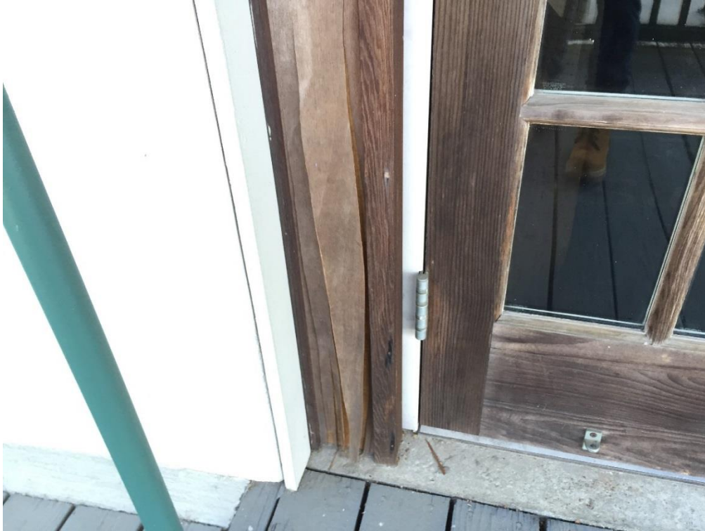
FIG TLH.53 – Close-up view of double door seen in FIG TLH.52 with peeling siding
