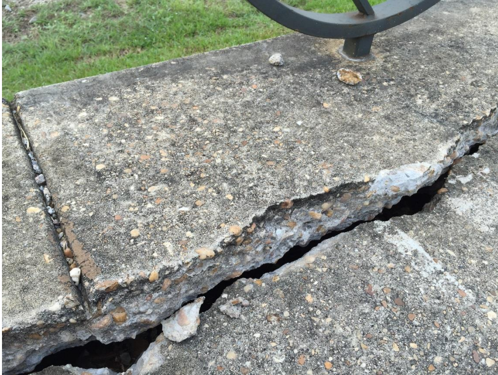
FIG MOE.09 – Close-up view of platform cracking seen in FIG MOE.08
