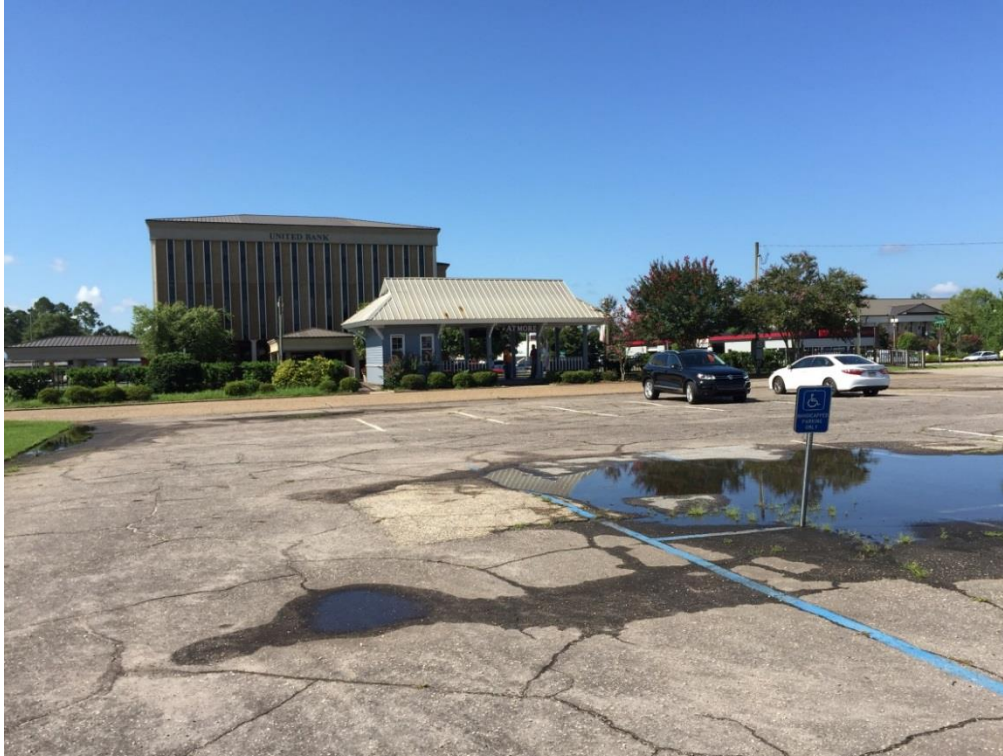
FIG ATR.03 – Parking showing standing water and cracking
