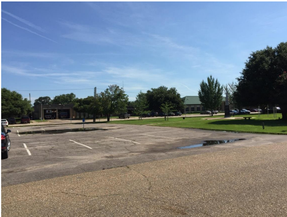
FIG ATR.02 – Parking showing standing water and cracking
