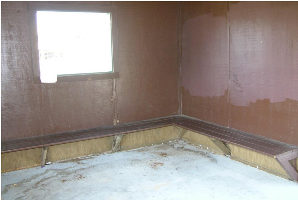
FIG CSV.06 – View of interior of structure showing water stains
