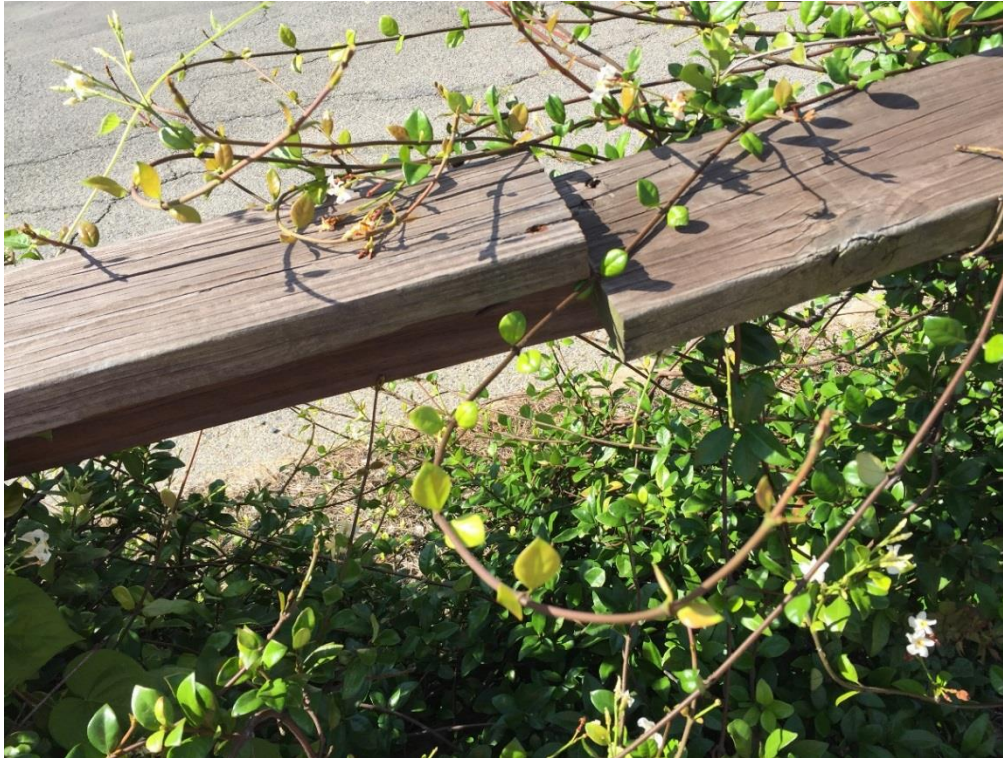
FIG GUF.13 – Section of deteriorating platform fencing
