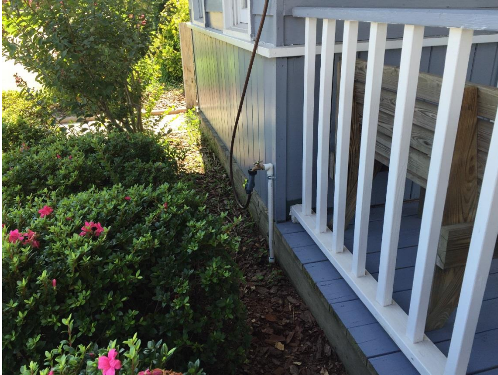
FIG ATR.17 – Hose bibb with flexible tubing connected—the tubing branches off and feeds in the various plant pots around the station structure
