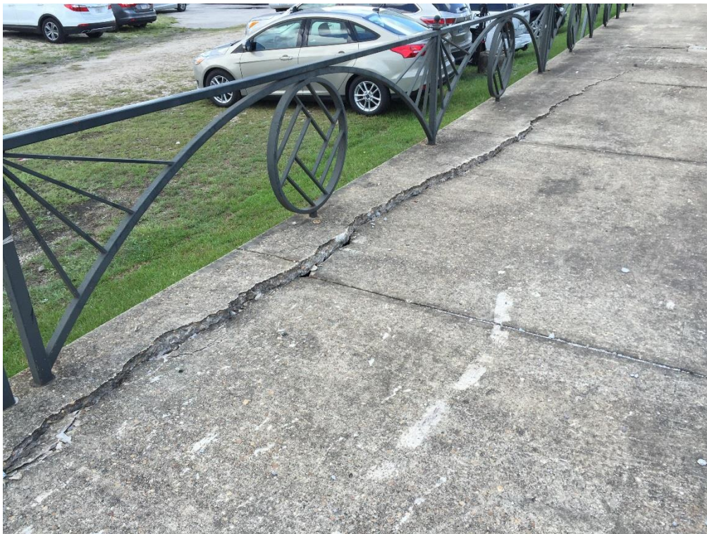
FIG MOE.08 – “Middle section” of platform experiencing excessive deterioration, see plan (“EX-2, Mobile AL” and “EX-3, Mobile AL”) for more precise location
