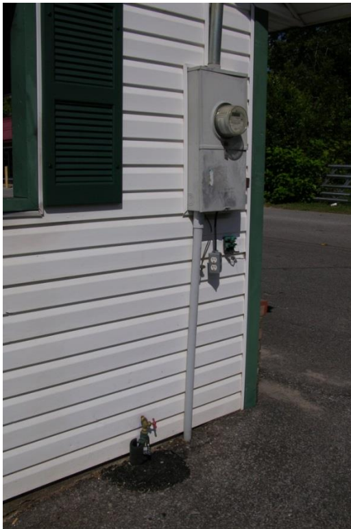
FIG CSV.12 – Electrical service on northeast exterior wall
