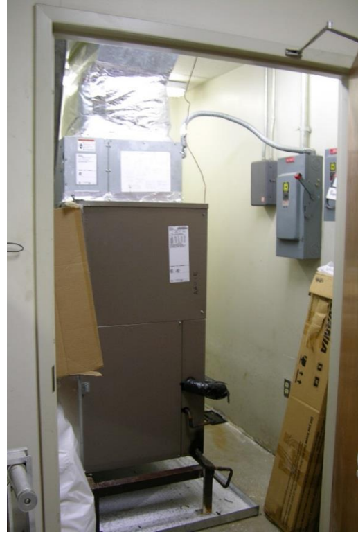
FIG TLH.56 – Air handler in separate utility closet
