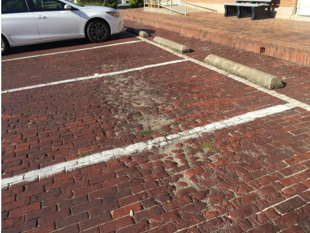
FIG GUF.03 – Cracked brick at parking lot
