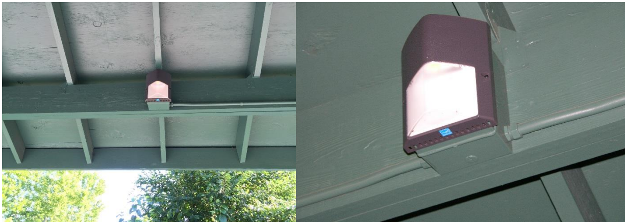
FIG TLH.57 & 58 – LED wall packs located on platform canopy
