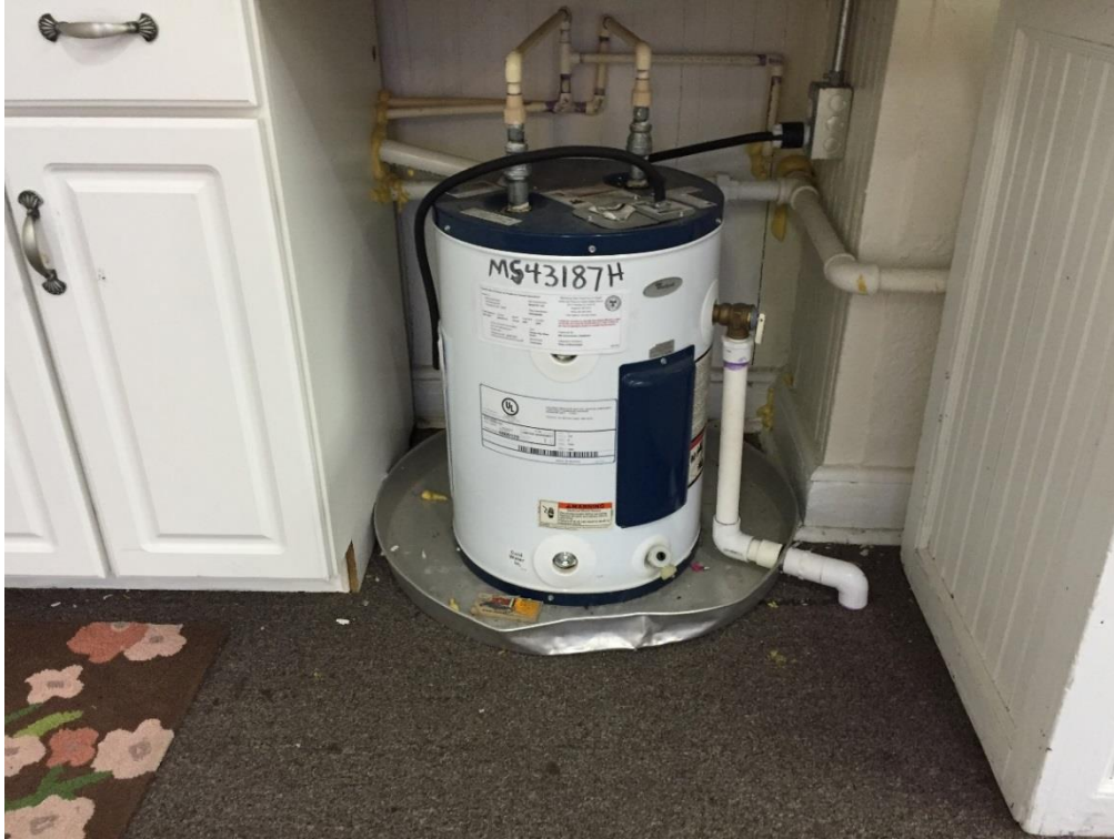
FIG PAG.23 – Water heater located in western wing of building (originally utilized as segregated waiting room for African American passengers)
