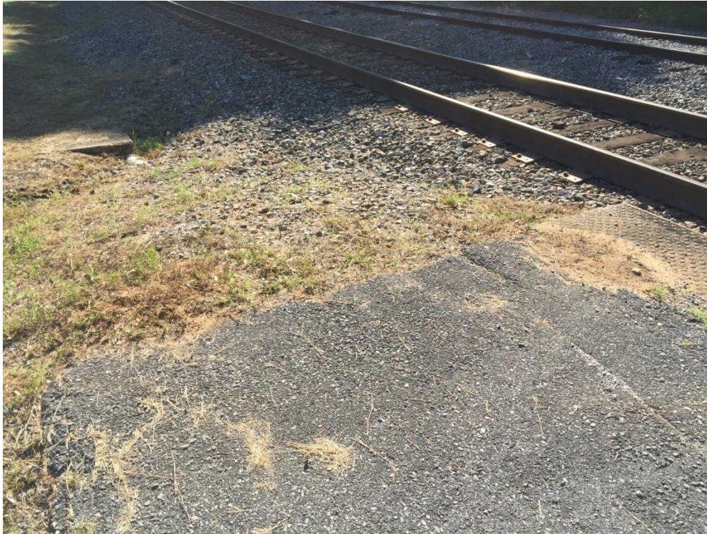
FIG CSV.15 – Portion of platform (15 LF, 150 SF total) on northeast end of platform that has deteriorated and must be replaced or removed & taken out of service.
