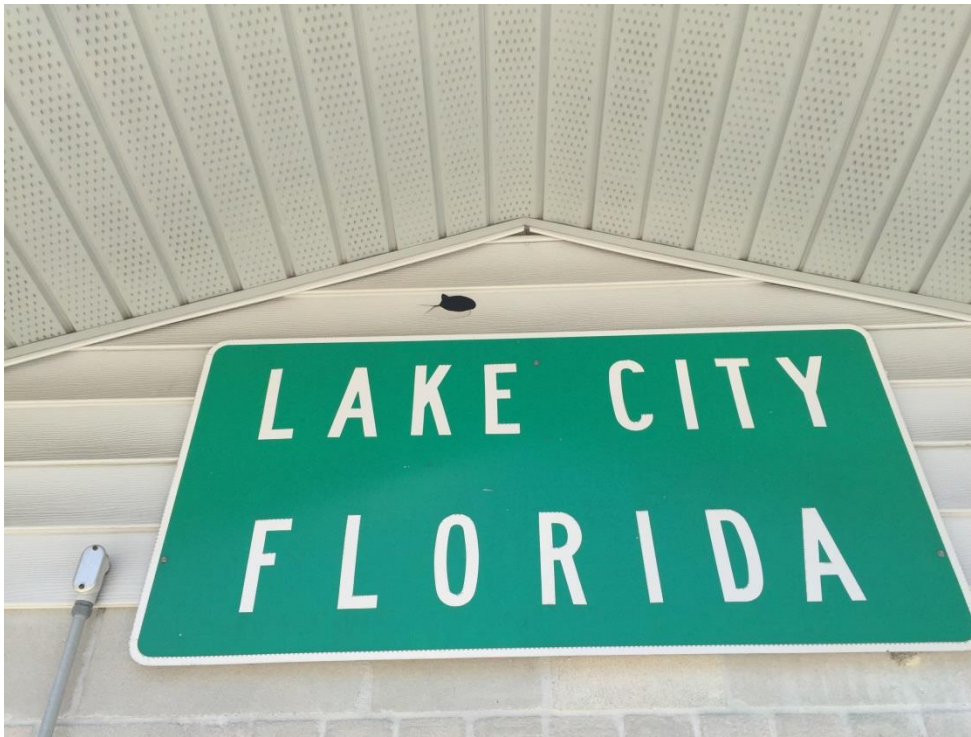
FIG LAC.10 – The signage at the shelter for Lake City FL station. Hole in siding visible above. Venting in side eaves visible.
