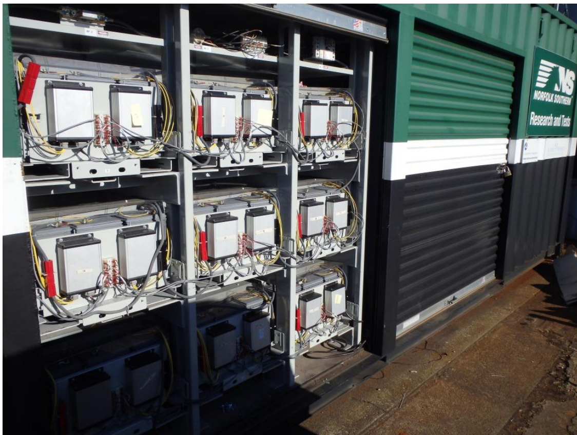
Figure 9. HLS outfitted with East Penn UltraBattery string
