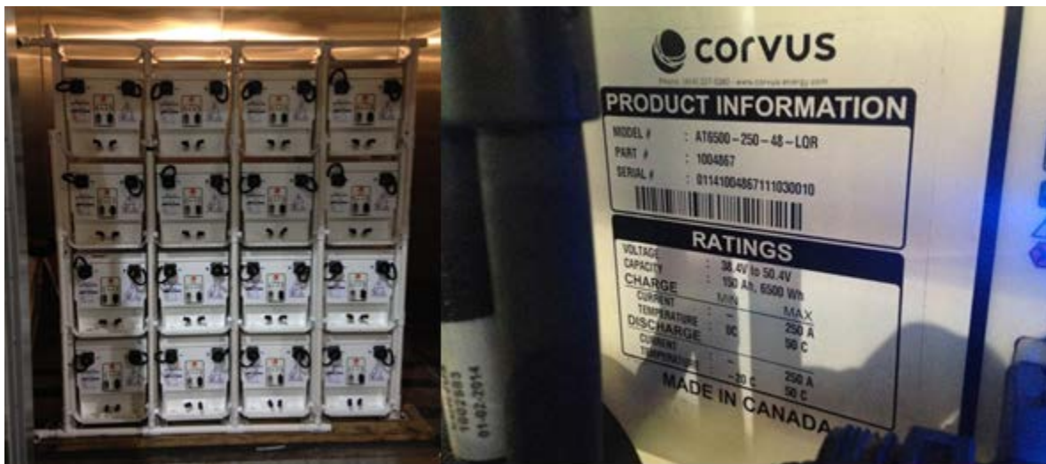
Figure 18. Corvus battery system enclosed in ESPEC chiller
