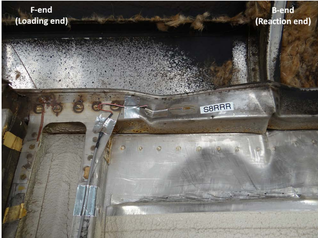
Figure B23. Post-test — Right Roof Rail Buckle at Section 8
