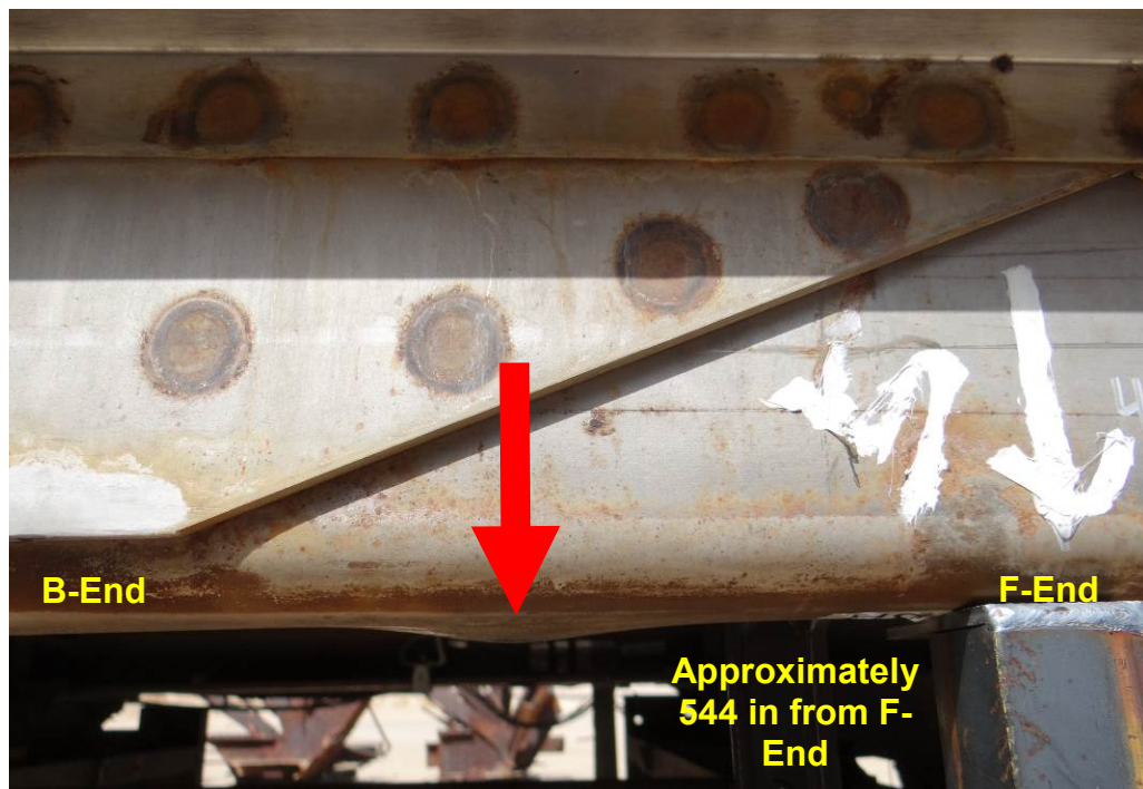
Figure 26. Damage on Right Side Sill Following 800,000-pound Load Test
