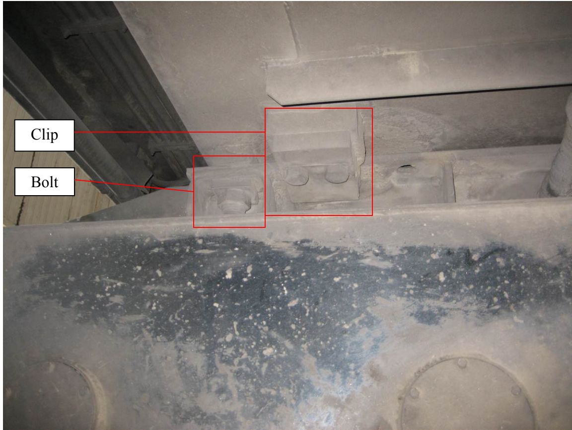
Figure A.3-2. Fuel Tank Attachment to Underframe
