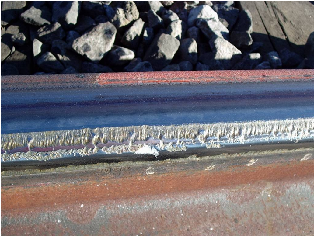
Figure 8. Typical Chip Noted on Gage Corner of Laser-Treated Trail After 1.2 MGT
