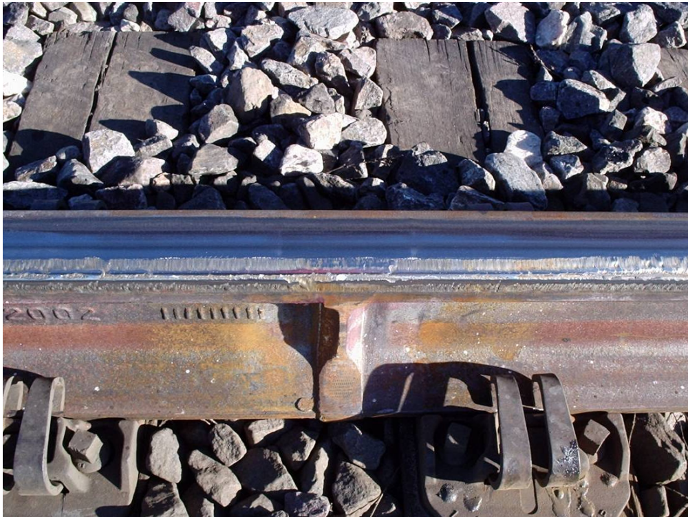
Figure 11. Overall View of Thermite Weld in Laser-Treated Section After 1.2 MGT. Compare with Figure 19 at the Same Location After 5.6 MGT
