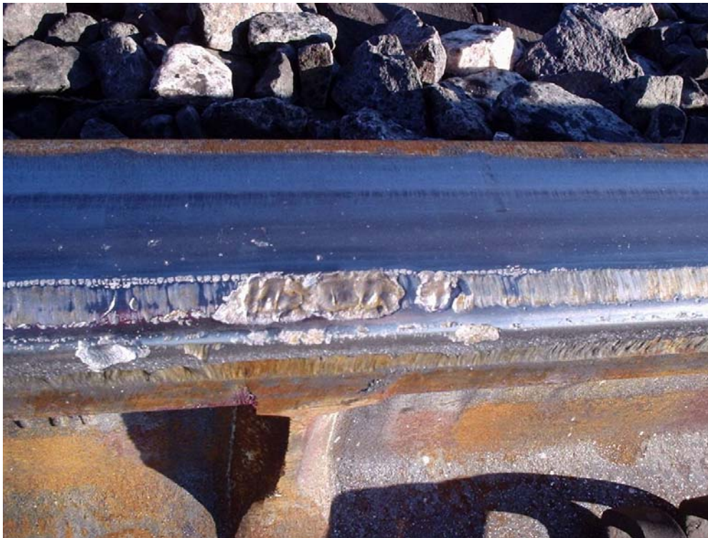
Figure 20. Close View of Spalls At and Near Thermite Weld After 5.6 MGT. Compare with Same Location as Shown in Figure 12 After 1.2 MGT
