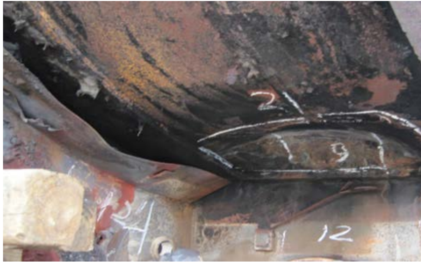
Figure 7: Burn through of tank shell on the outboard A-end, left side of draft sill.
