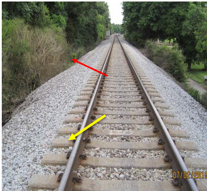
Figure 1: POD (yellow arrow) and location of failed roller bearing (red arrow).
