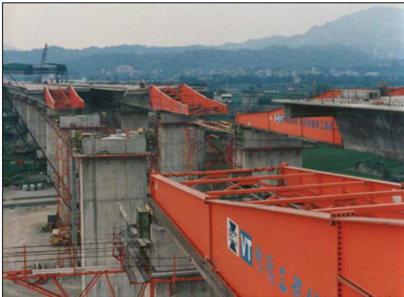
Figure 4: Incremental Launching Method Equipment Used on the Tou Chien Bridge Second Freeway, Taiwan (Photo courtesy of Wiecon)
