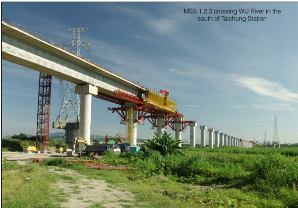
Figure 9: MSS Moving Forward to the Next Span, Bent Construction Well Advanced of the Girder Placement, Taiwan High-Speed Rail, ROC (Photo courtesy of THSRC)
