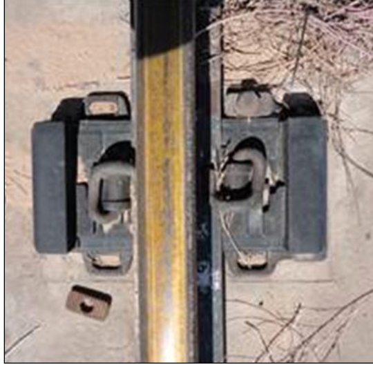
Figure 20. DFST Fastener with Three Missing Bolts
