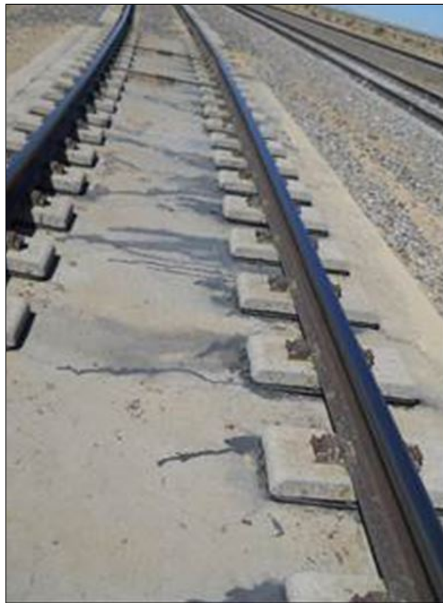
Figure 16. Staining of the Concrete Slab from Rubber Boot Abrasion
