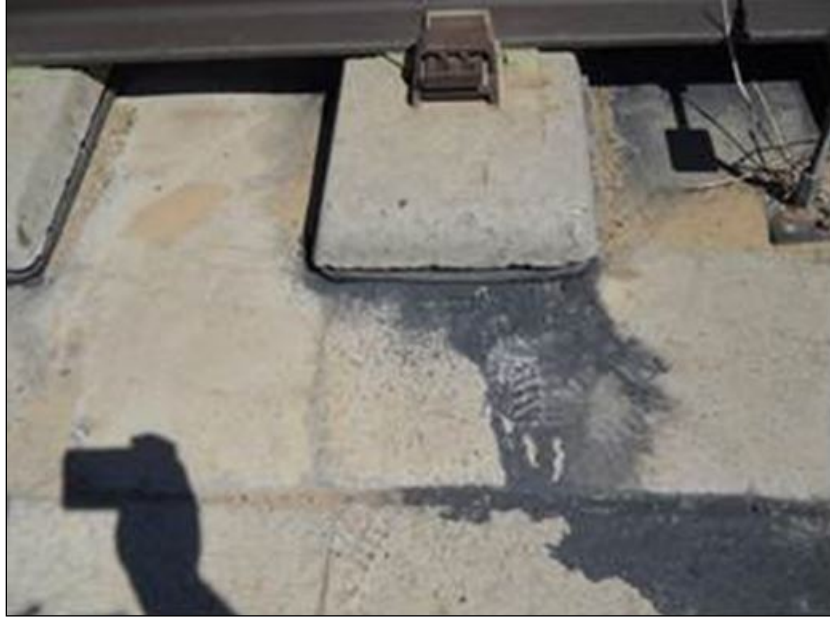
Figure 17. Close-up of Rubber Boot Deterioration and Staining
