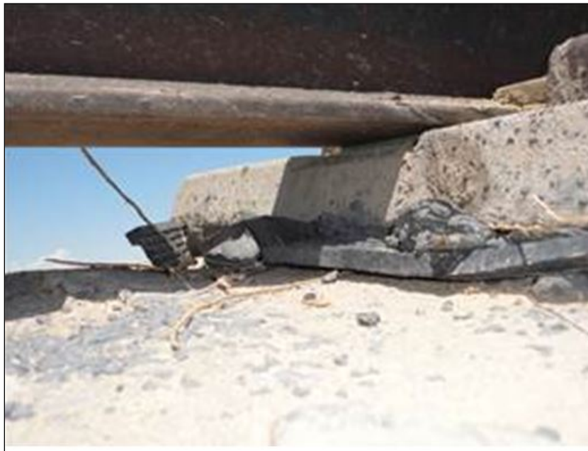
Figure 18. Close-up of Rubber Boot Abrasion and Deterioration
