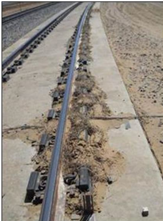
Figure 1. Sand and Debris Accumulation on the Slab Track
