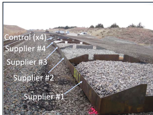
Figure 1. Ballast Box Installation in 2010. Ballast Type Number, Box Number, and Supplier Number Corresponds to the Same Box
