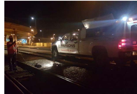
Integrated testing on PTC territory at turnout.
