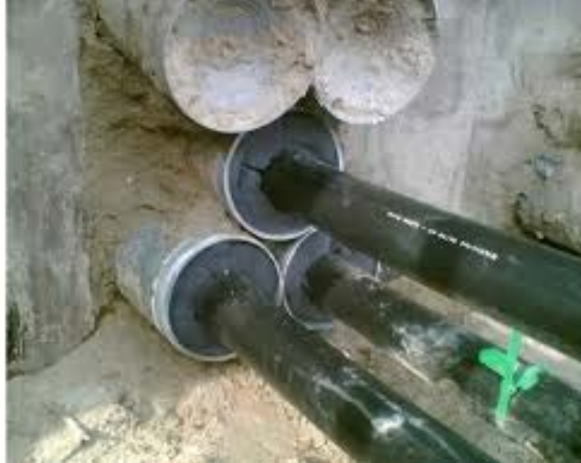
Figure 15. Concrete-Encased Fiber Conduit
