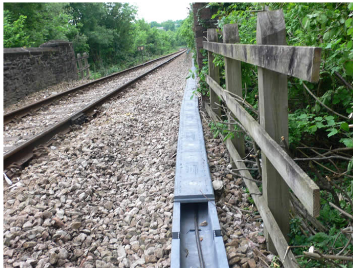
Figure 16. Fiber Optic Cable Wayside Enclosure
