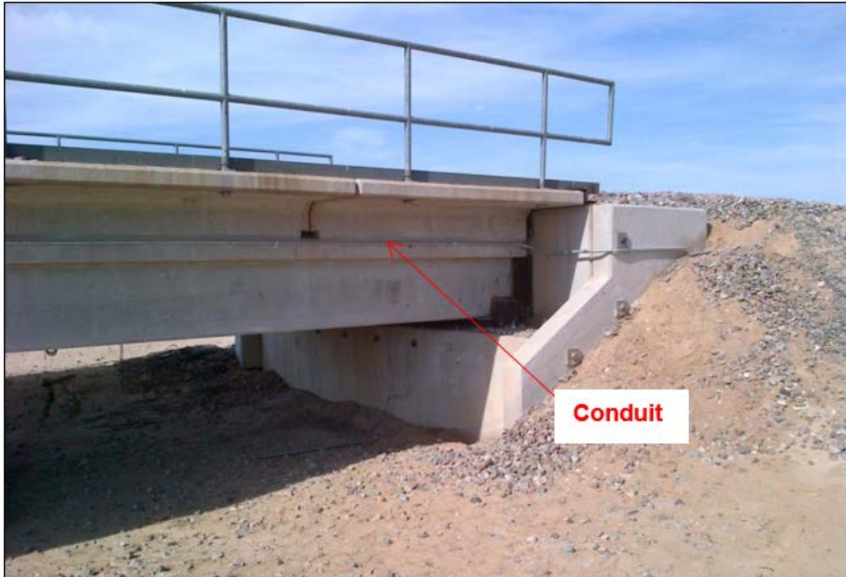
Figure 4. HTL Bridge with Fiber Optic Conduit
