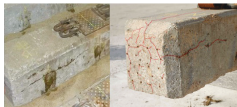
Figure 1. Splitting (left) and bursting cracks (right) observed in pretensioned concrete ties.
