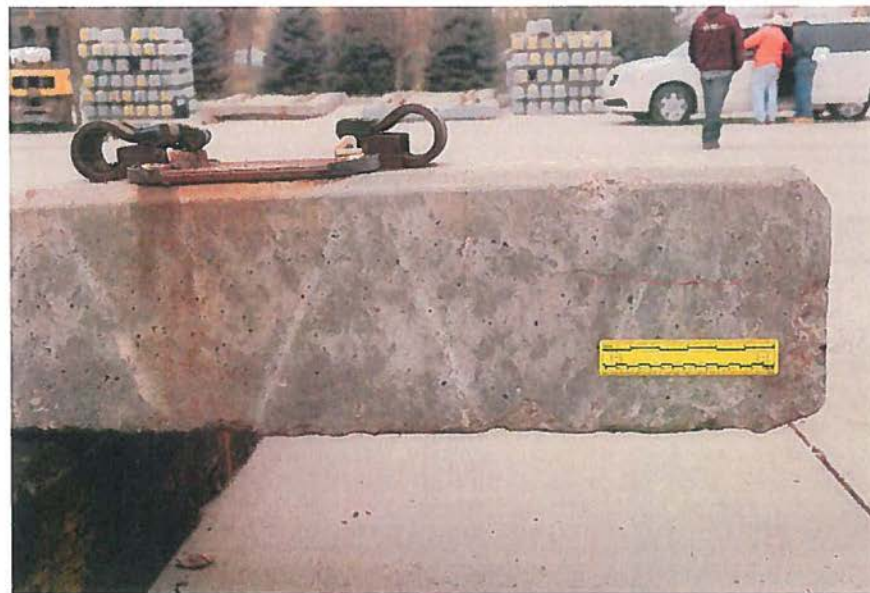
Figure 20. Opposite side of south end of tie NDT #7. L3672 102312 14
