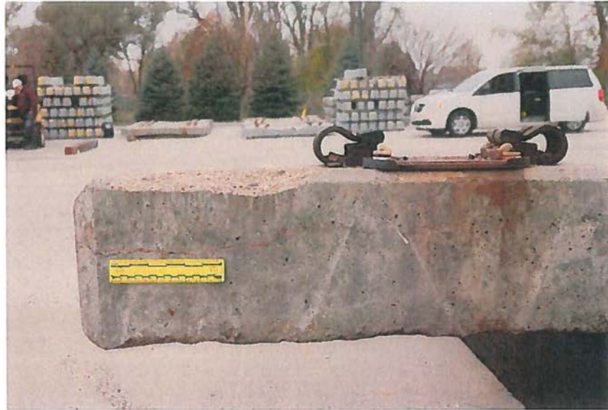
Figure 7. Side view of north end of the NDT #7, visible crack outlined in red.
