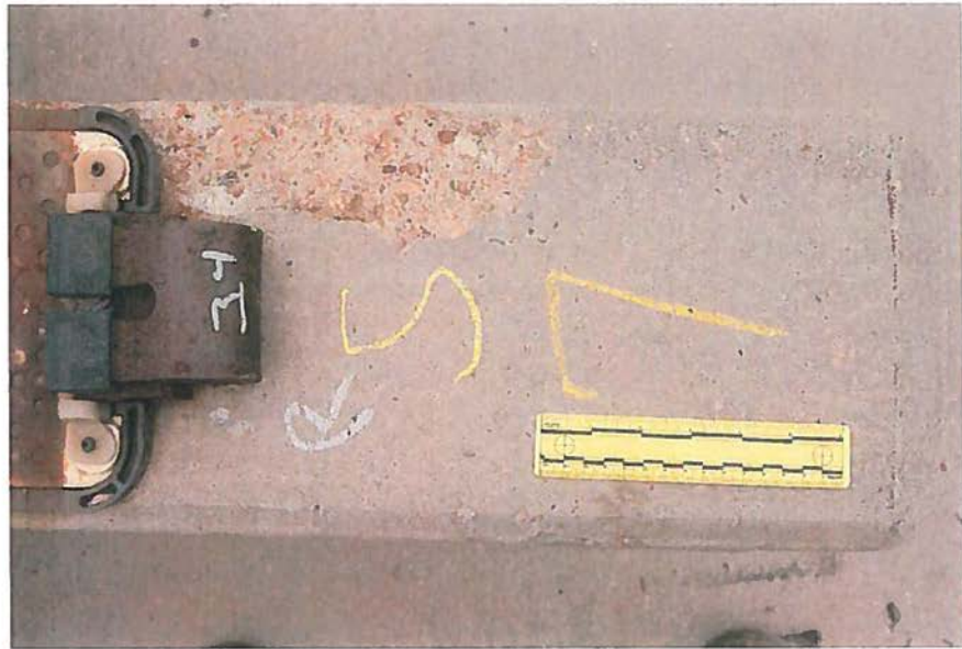
Figure 15. Top surface at south end of tie NDT #7 rated by NDT as "1" condition. L3672 102312 09
