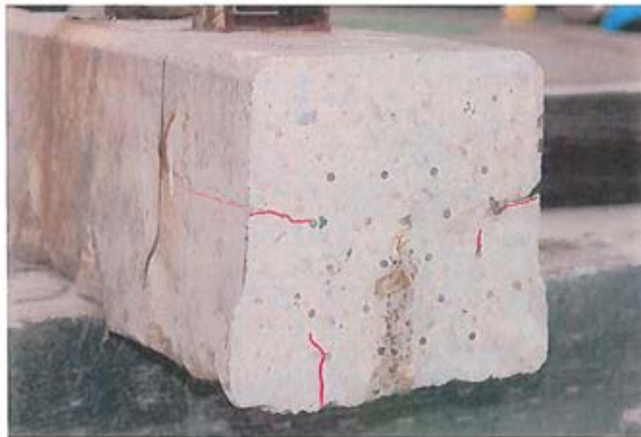
Figure 62. Oblique view of south end of tie NDT #1 after removal of 8 inches from end. L3672 103312 84
