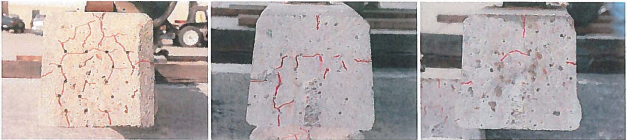
Figure 30. North end cross-sections of tie NDT #69 at exposed end (left), saw cut at 4 inches (center) and saw cut at 8 inches (right), all visible cracks outlined in red.
