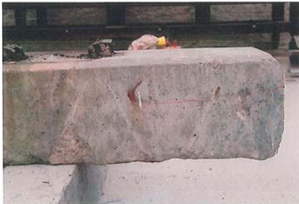
Figure 58. Opposite side view of south end of tie NDT #1 with horizontal crack 13 inches long outlined in red. L3672 102512 75
