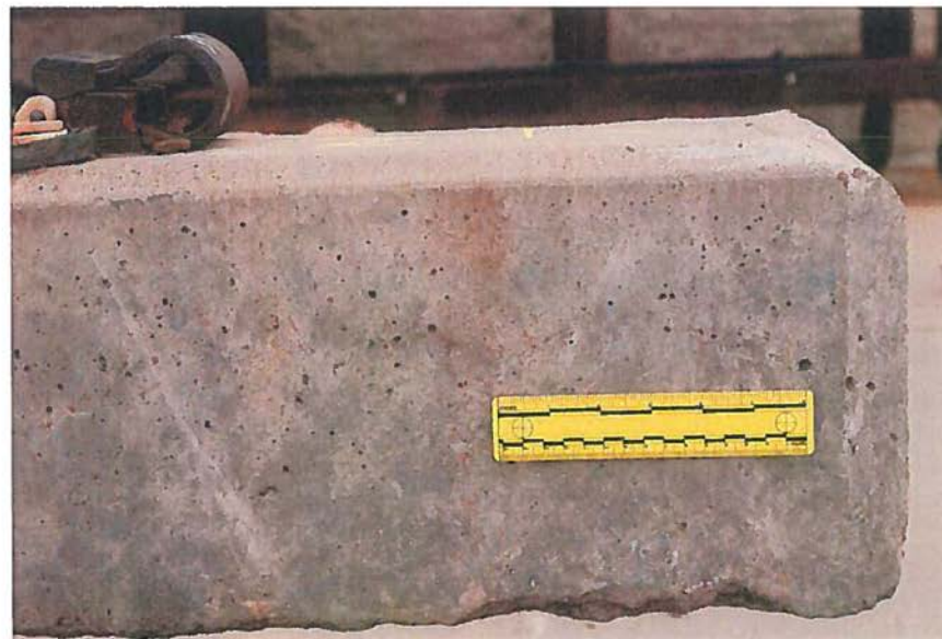
Figure 10. Close side view at north end of tie NDT #7, visible crack not outlined. L3672 102312 08
