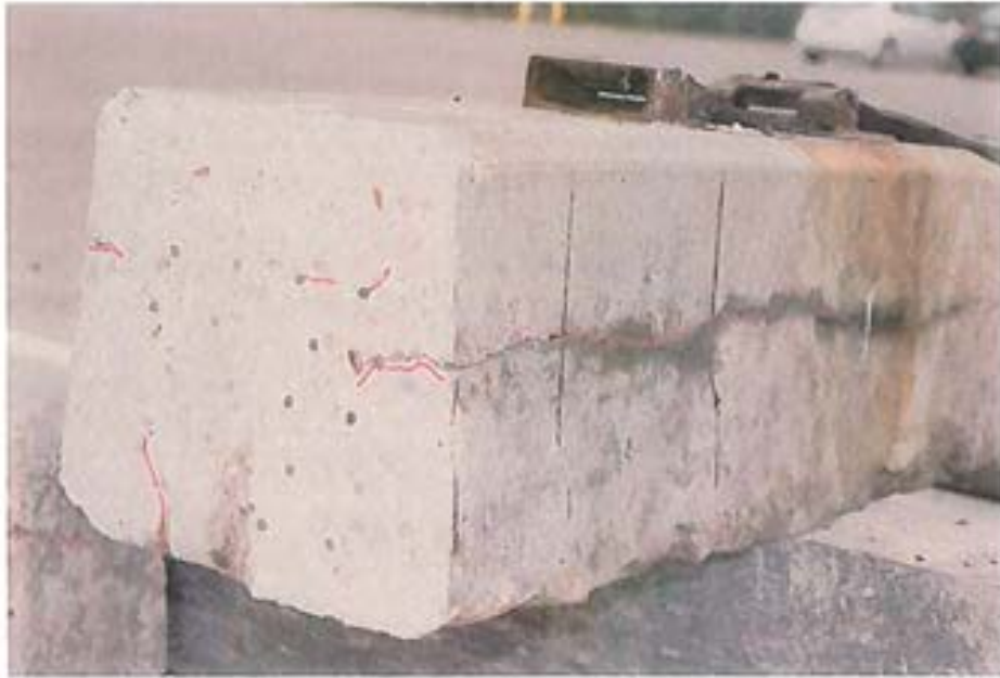
Figure 61. Opposite side oblique view of south end of tie NDT #1 after removal of 4 inches. L3672 103312 80
