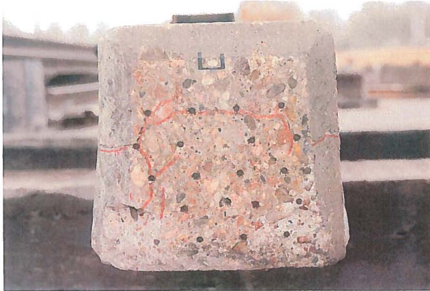
Figure 53. South end of tie NDT #2, cracks outlined in red. 1.3672 102312 64
