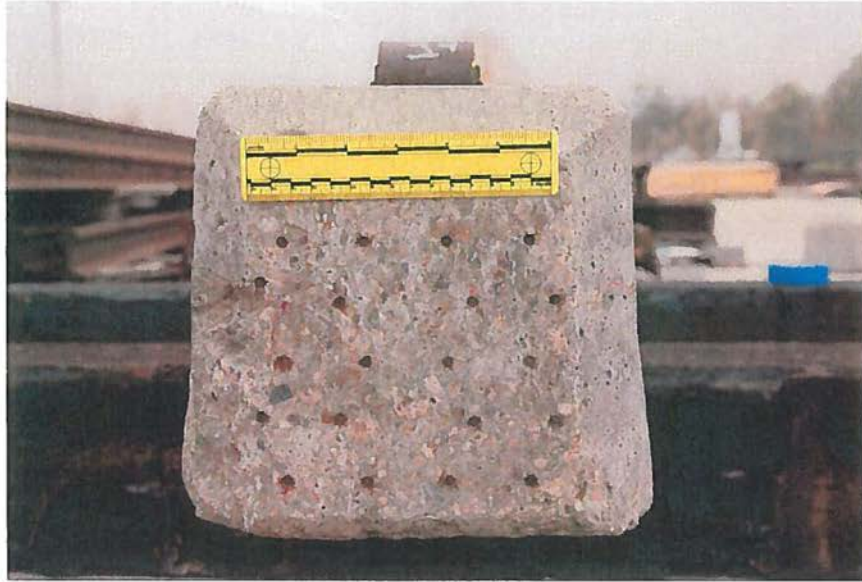
Figure 17. South end of tie NDT #7 without outlining of cracks. L3672 102312 11
