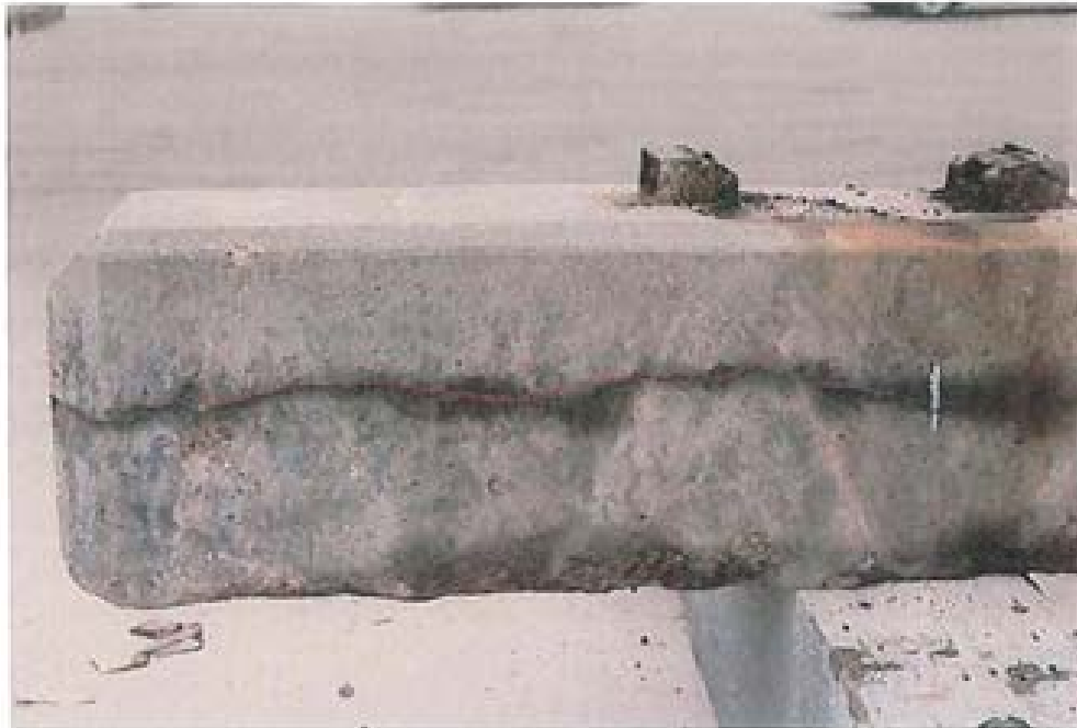
Figure 57. Side view of south end of tie NDT #1 with horizontal crack 21 inches long outlined in red. L3672 102512 74
