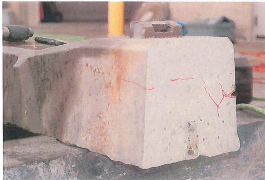
Figure 46. Oblique side view of tie NDT #2 after removal of 21 inches at end, center of rail pad. L3672 102312 58
