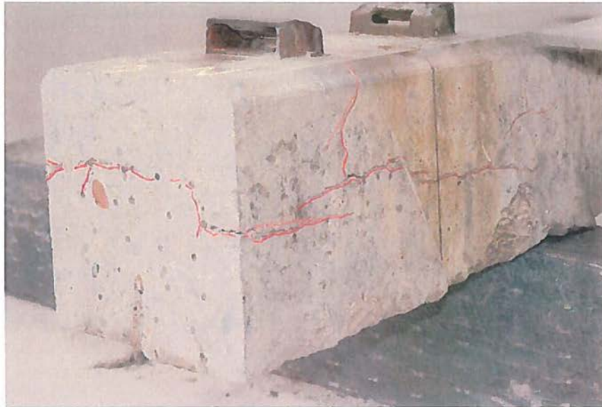
Figure 45. Opposite side oblique end view of tie NDT #2 after removal of 10 inches at end. L3672 102312 52
