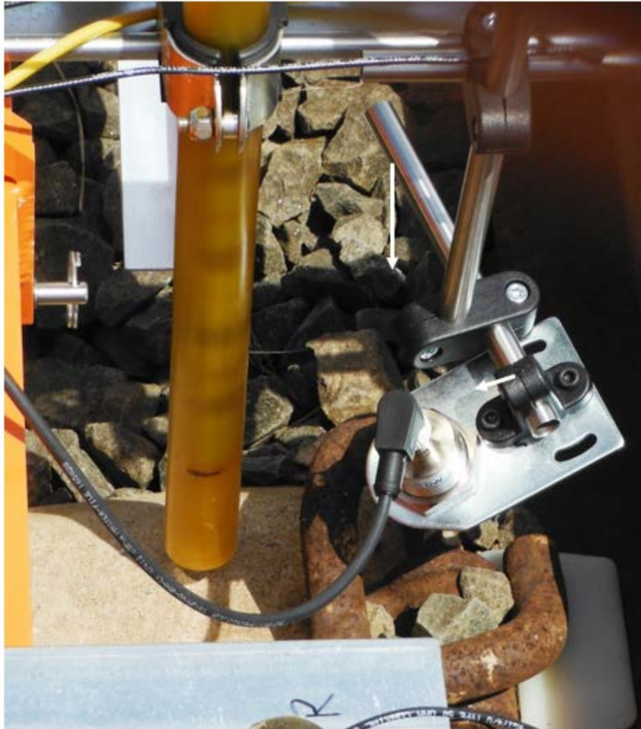
Figure 19. Magnetic Proximity Switch Installed on ACTT-2
