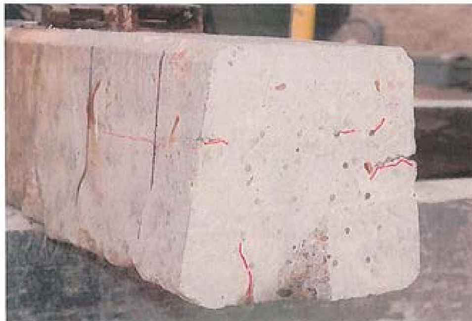
Figure 60. Oblique view of south end of tie NDT #1 after removal of 4 inches, cracks outlined in red. L3472 102312 77
