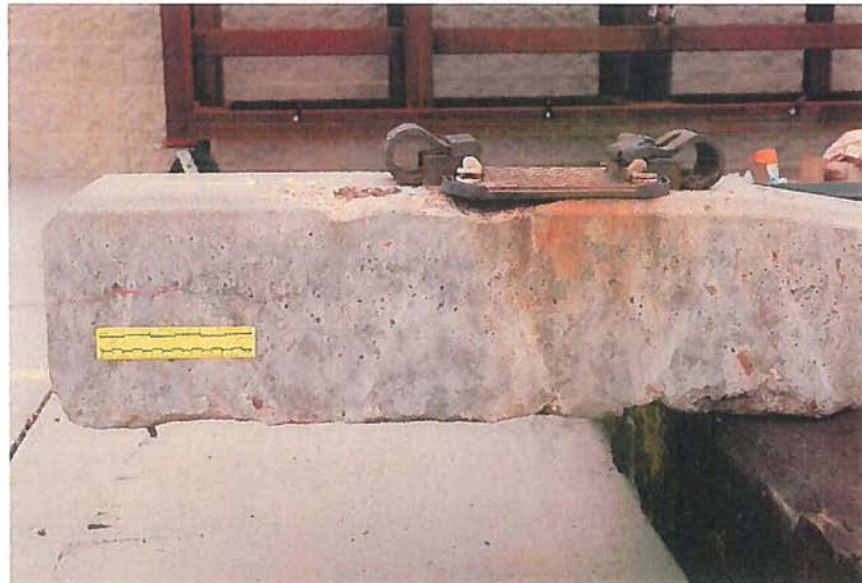
Figure 18. Side view at south end of tie NDT #7. L3672 102312 12
