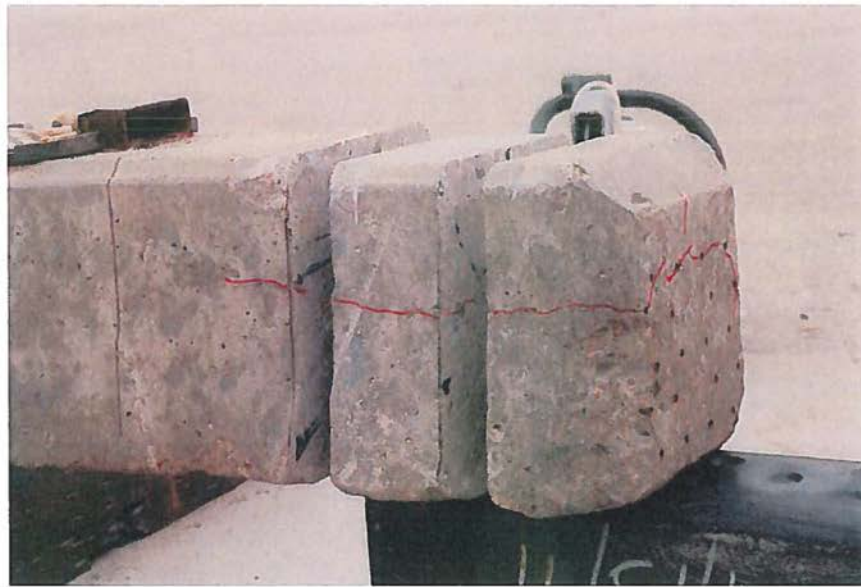
Figure 22. Oblique view of sections removed at 4 inches and 8 inches from south end of tie NDT #7 with cracks outlined in red. L3672 102312 19
