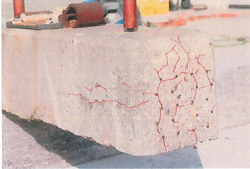
Figure 29. Opposite side oblique north end view of tie NDT #69. L3672 102312 34
