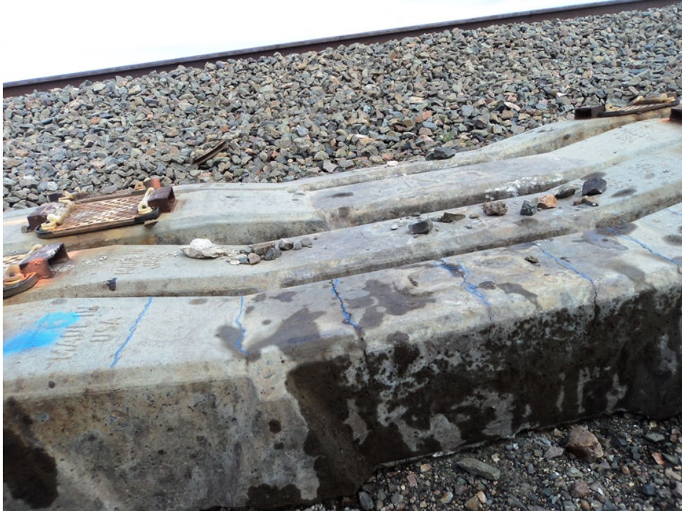
Figure 11. UP Ties with Center Cracking
