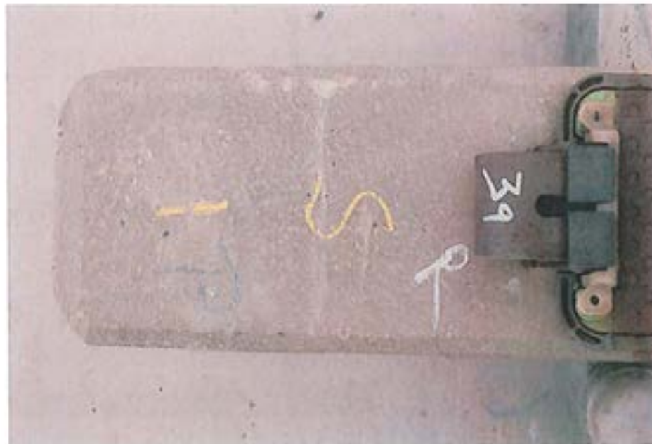
Figure 56. Top surface of south end of tie NDT #1 rated condition "3" by NDT and condition "1" by visual. L3672 102512 73
