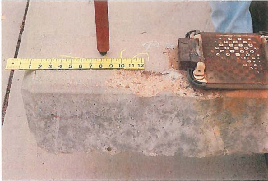
Figure 3. Closer view at the south end of tie NDT #7 showing distance from most outboard transducer to the end of the tie during testing. L3672 102312 17
