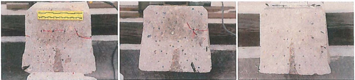
Figure 14. Cross-sections at saw cut locations on tie NDT #7 at 4 inches (left), 14 inches (center) and 21 inches (right) at center of rail pad, all visible cracks outlined in red.
