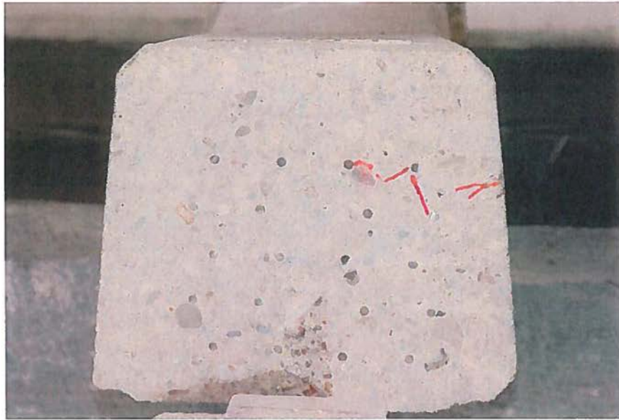
Figure 49. Cross-section at saw cut 28 ½ inches from north end of tie NDT #2, inboard of rail pad towers. L3672 102312 60
