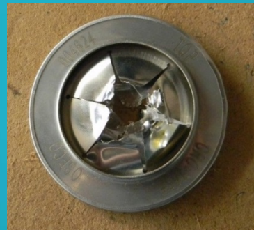
Blown Rupture Disc
