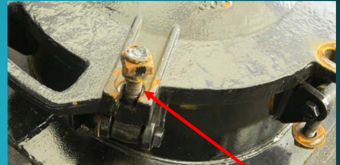
Safety eyebolt slightly loose in place with nut still attached.
