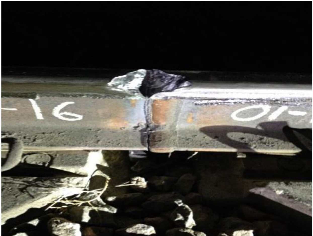
Figure 10. FAST Log Broken Rail Picture
