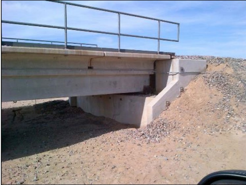
Figure 4. HTL Bridge with Fiber Optic Conduit
