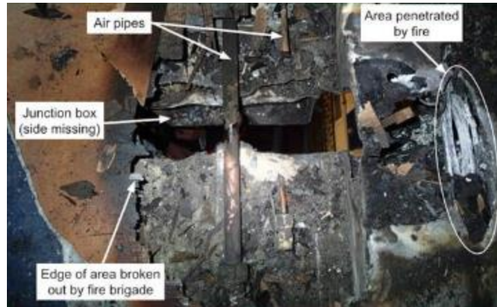
Figure 2-1. Photograph of Damage to Floor Inside Tram Rail Car from UK Incident on January 30, 2015
