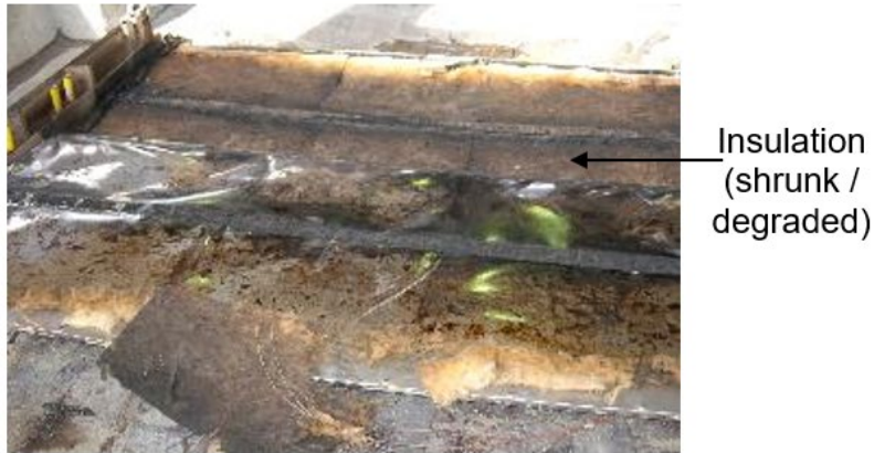
Figure 6-5. Post-Test Pictures of the Unexposed Surface of a Rail Car Floor Showing Shrunken/Degraded Insulation
