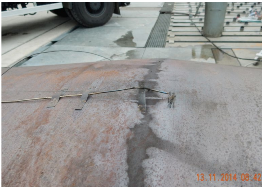
Figure 91. Test 5 with Insulation Removed. View of tank deformation at location of insulation gap and separated thermocouple.
