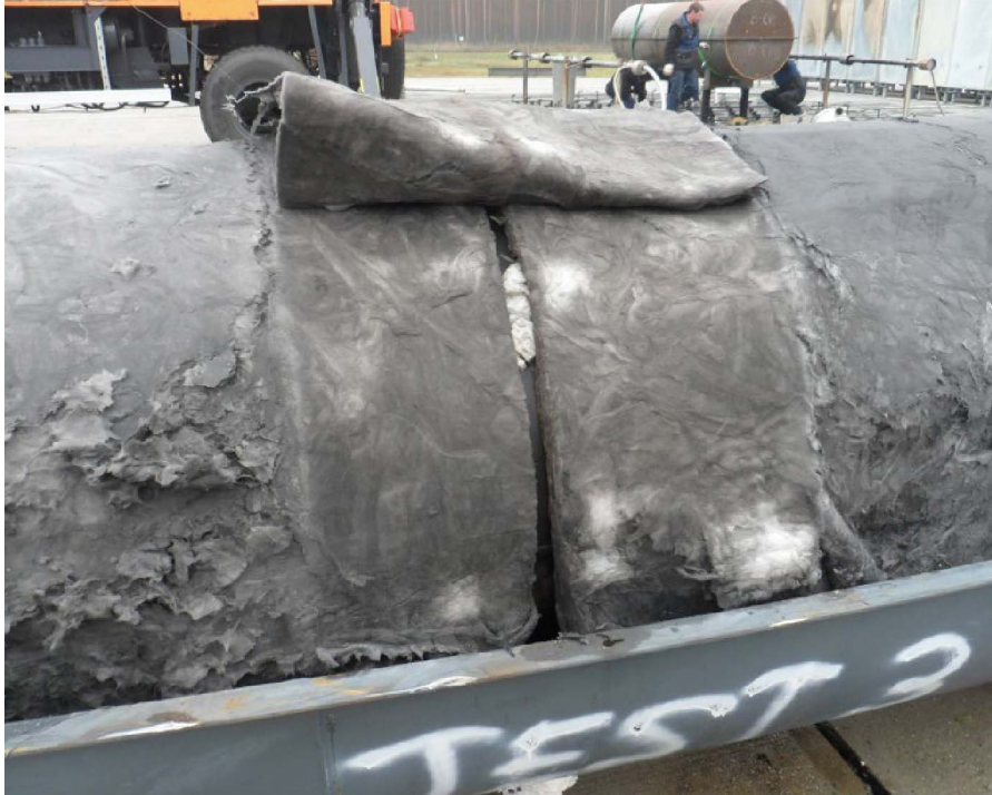
Figure 72. Test 3 - View showing Second Layer of Insulation Lifted to Show Gap. Note condition of protected insulation.
