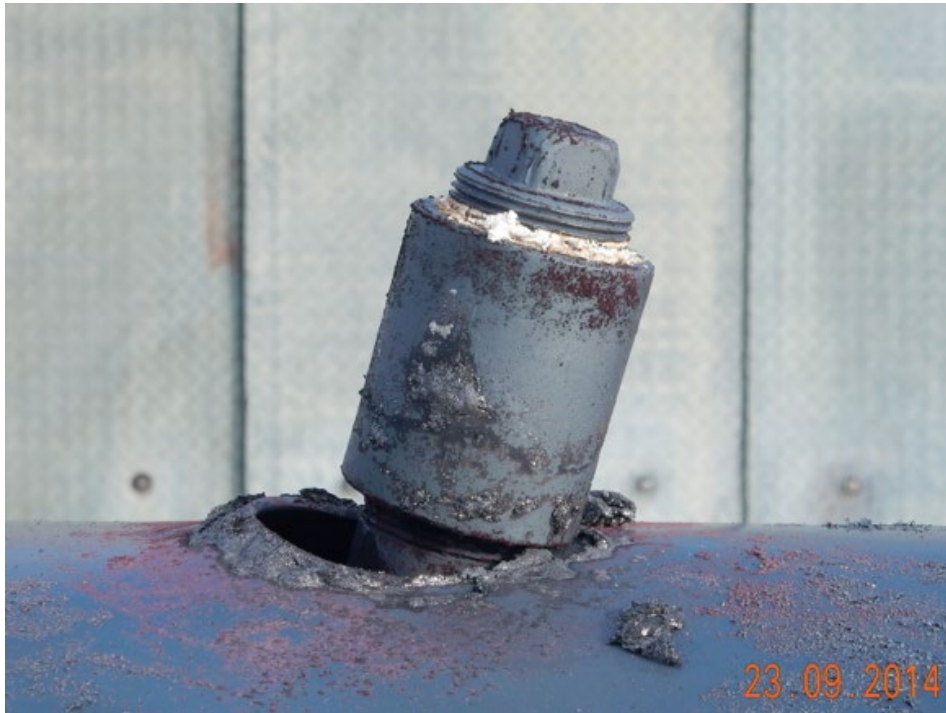
Figure 42. Test 1 - View of Damaged Fill Pipe on B-End (East) (Location of Minor Failure)
