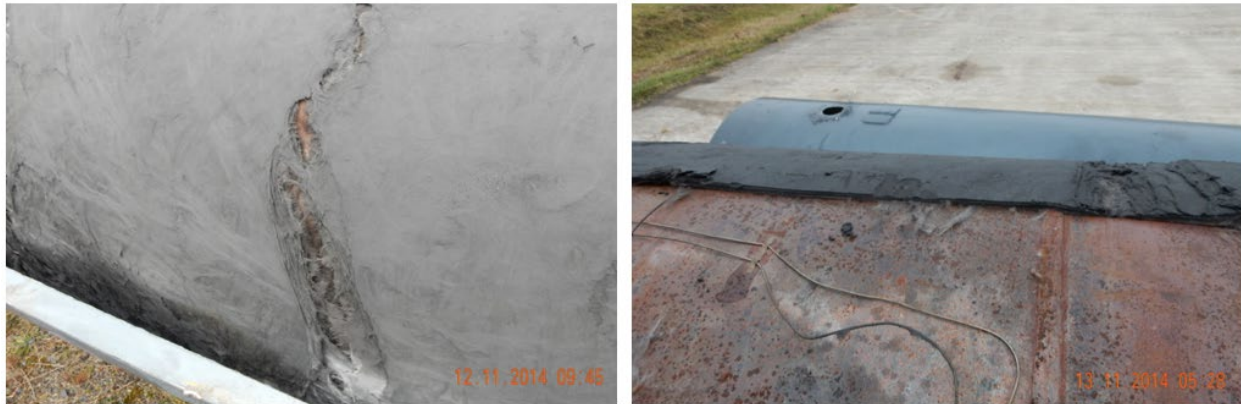
Figure 29. Test 4 – Images of Insulation Failure
