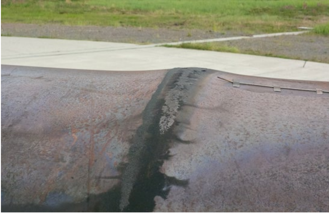
Figure 45. Test 1 - Plastic Deformation at Location of Separated Insulation
