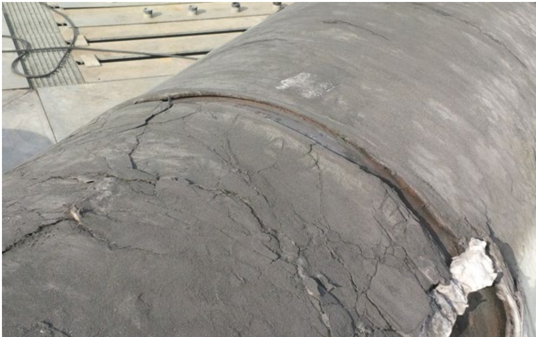
Figure 44. Test 1 - View of Separated Insulation on Tank Top at Mid Span Picture also shows severe thinning of insulation.
