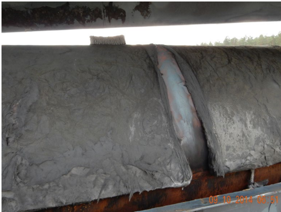
Figure 62. Test 2 - Insulation Gap at Mid Tank
