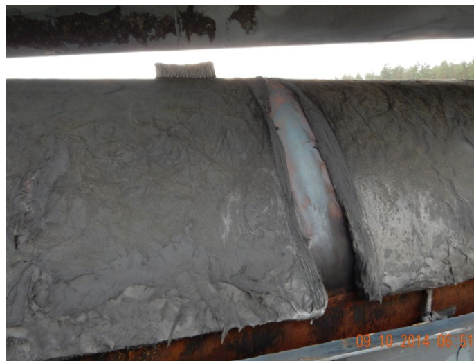
Figure 17. Test 2 - Insulation Separation at Mid-Tank
