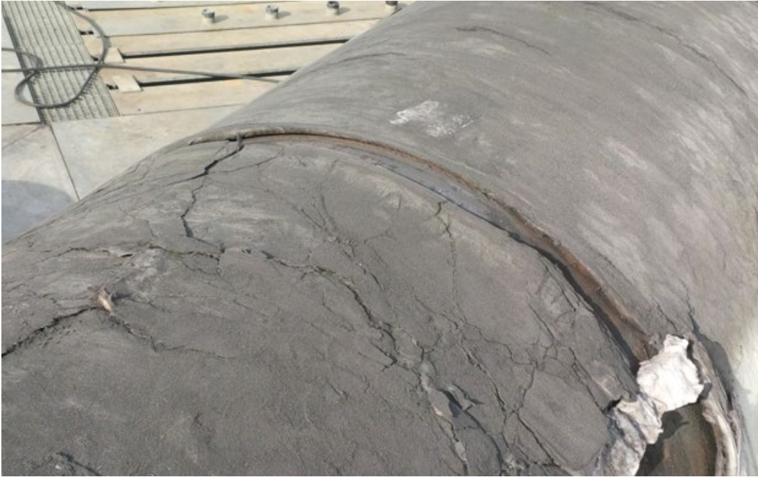
Figure 15. Test 1 - View of Separated Insulation on Tank Top at Mid Span. Picture also shows severe thinning of insulation.
